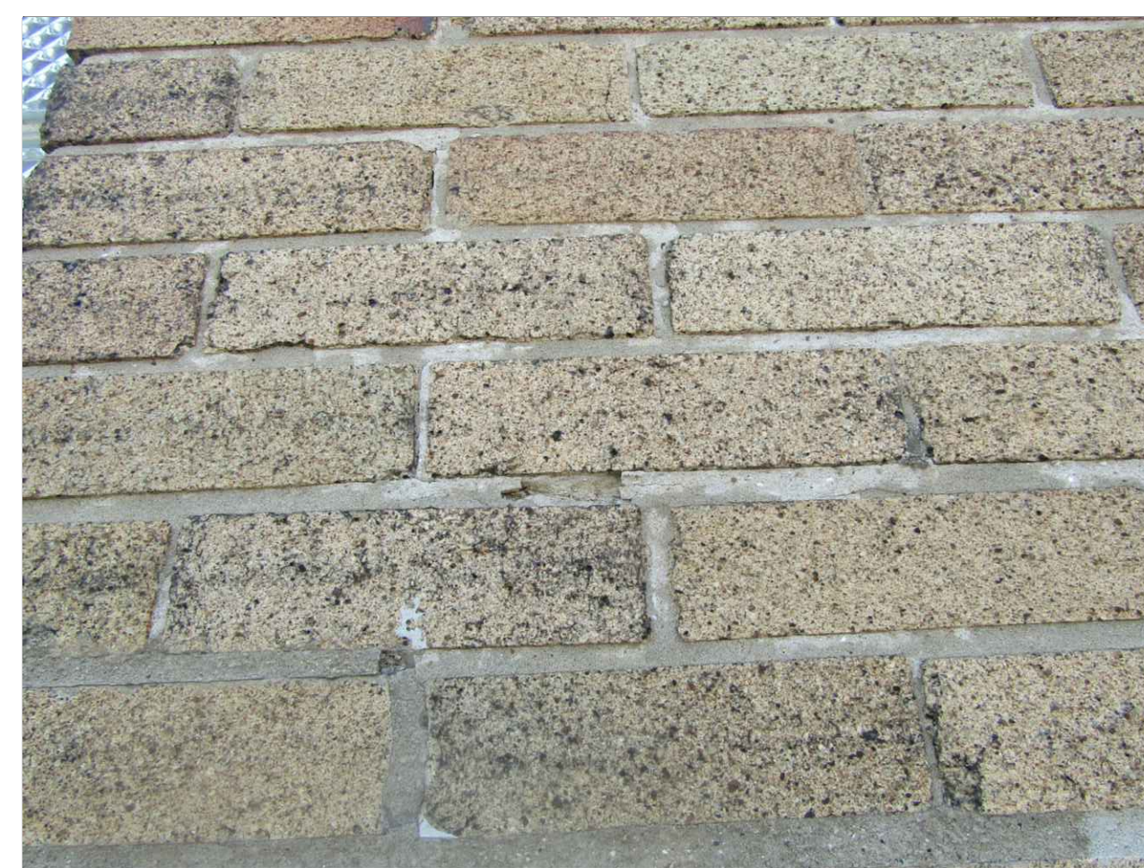
DETERIORATED MORTAR JOINTS
