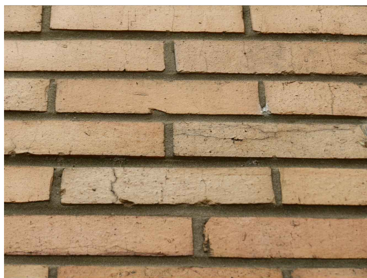
CRACKED AND SPALLING FACE BRICK
