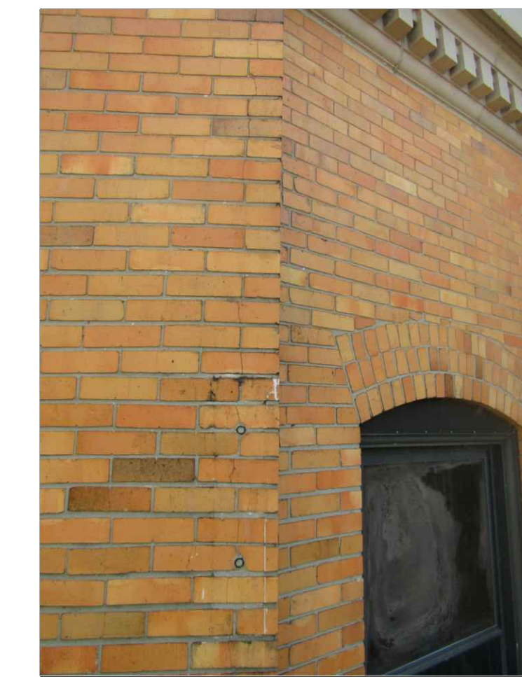
FACE BRICK CRACKING AT CORNER
