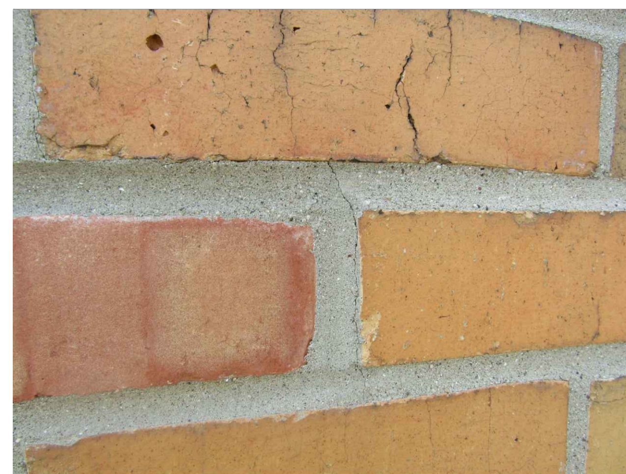
CRACKED AND DETERIORATED MORTAR JOINTS
