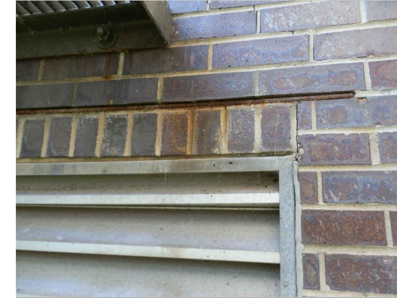
MORTAR DETERIORATION DUE TO CORROSION AT LINTEL
