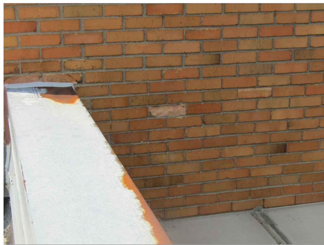
SPALLED FACE BRICK
