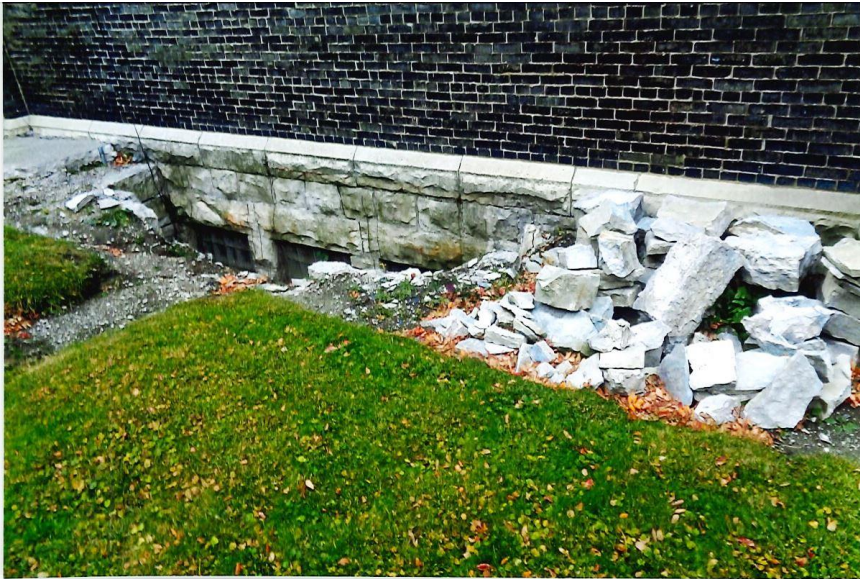
LEFT: Collapsed window well.
