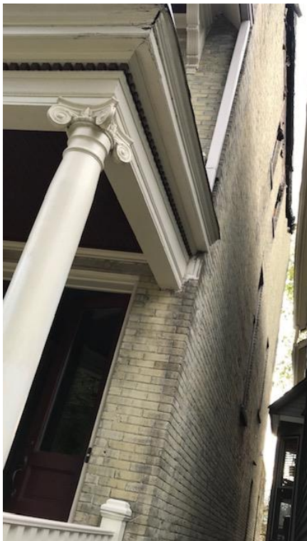
NE View Toward Damaged Wall
