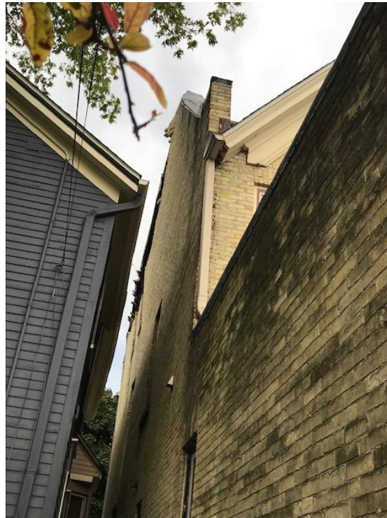
NW View Toward Damaged Wall
