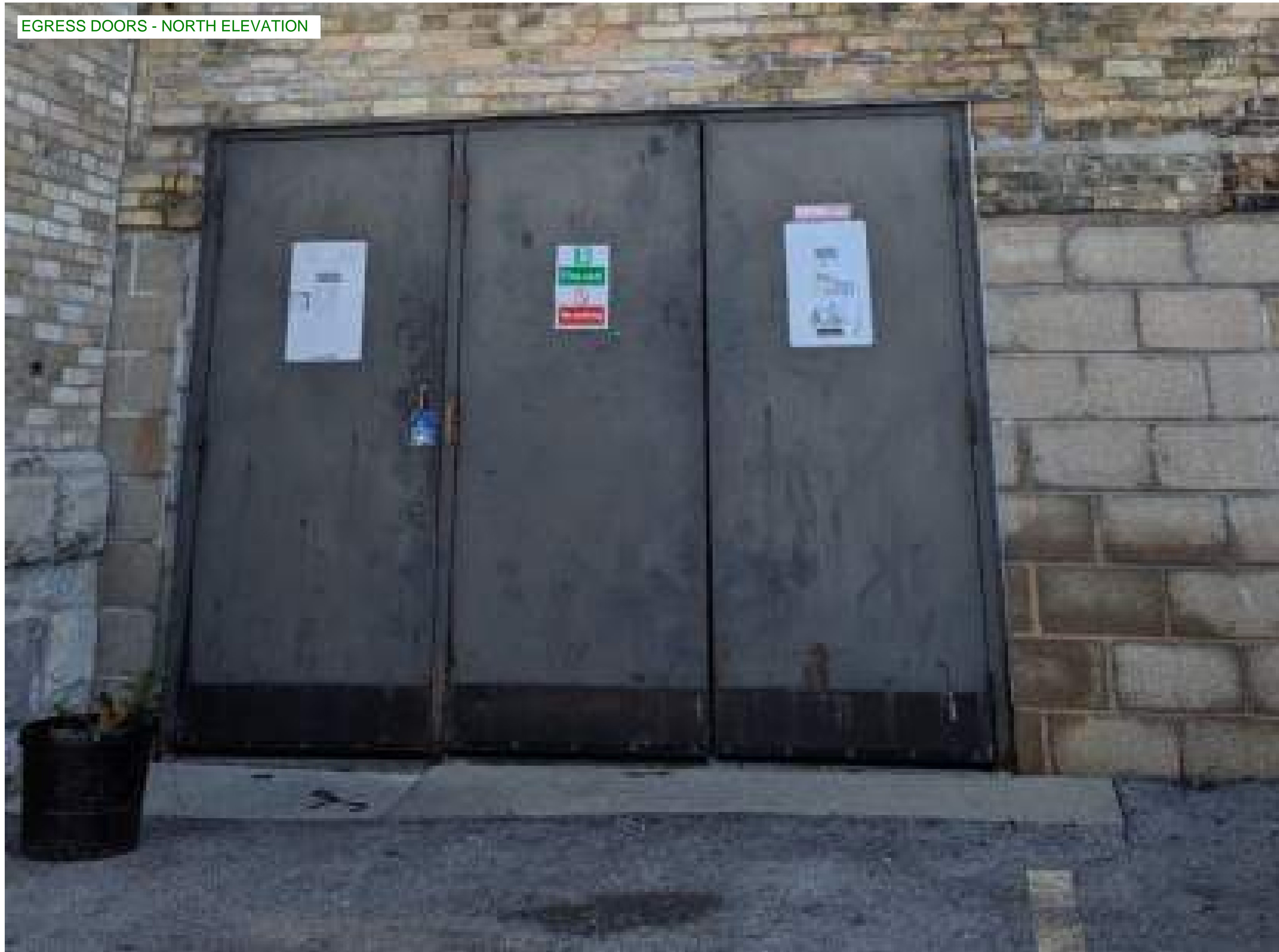
Non-original metal doors, in non-original opening to be replaced with new metal single panel doors. Doors and frames to be painted cream to match adjacent historic brick
