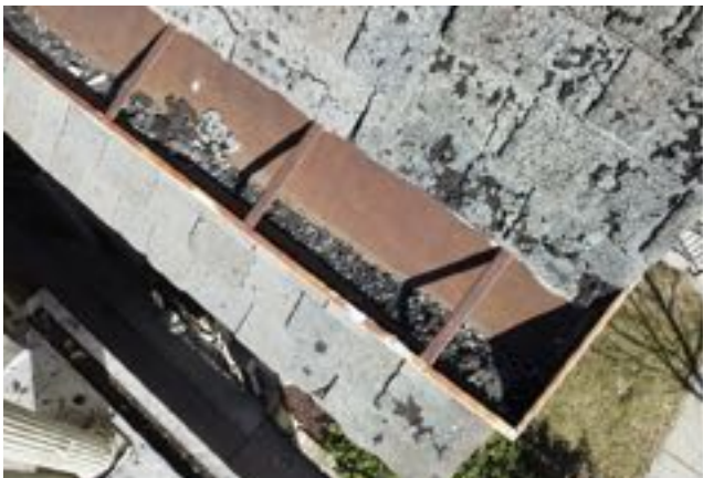
IMAGE 2: South roof slope, east edge eave and surface-mounted gutter corrosion.
