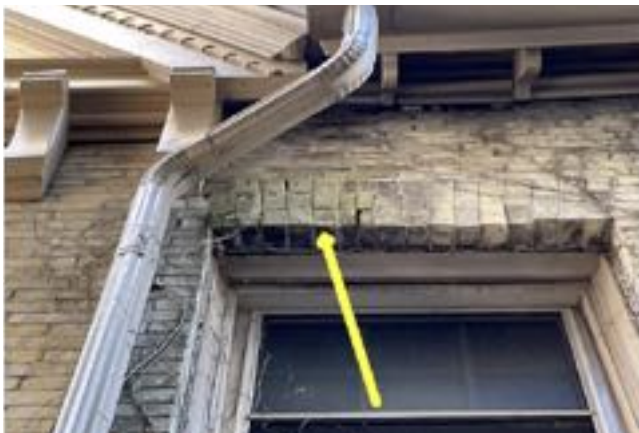
IMAGE 8: North elevation third-floor window head is near collapse.
