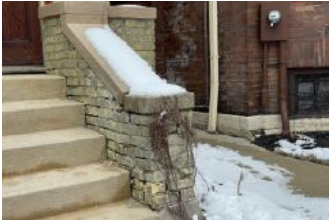
IMAGE 7: Stair check wall masonry deterioration.
