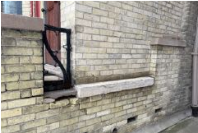
IMAGE 9: Main entry porch remnant with wrought iron on the north elevation.
