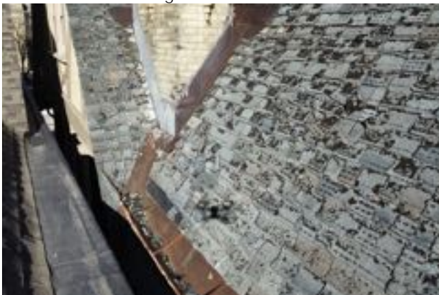
IMAGE 3: South roof slope, east edge eave, chimney flashing, and surface-mounted gutter corrosion.
