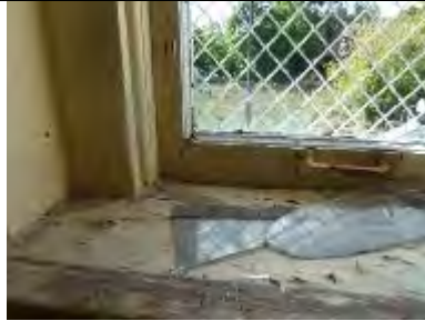
S323-02: Rotted interior sill & damage to lower rail
