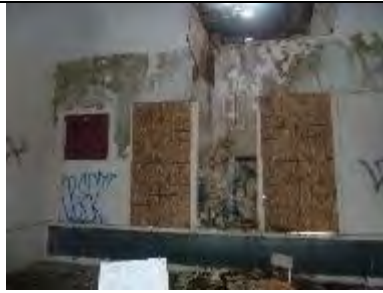
N320-02: Water damage above window
