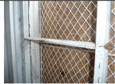
N217-03: Broken muntin bar
