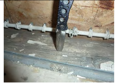
W211-03: Rotted sill
