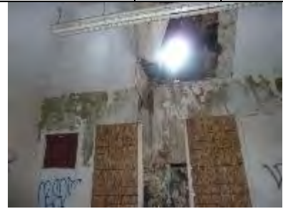
N320-03: Hole in roof & ceiling above window
