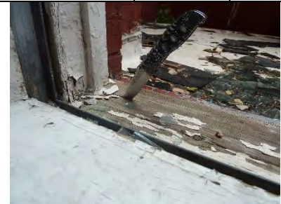
LC209-03: Exterior sill decay
