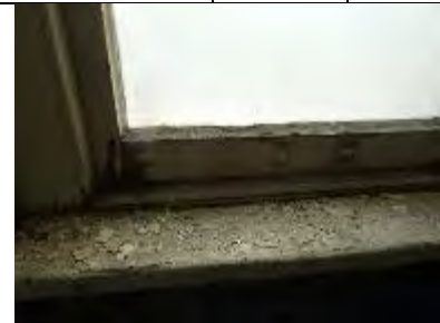
E310-03: Damage along lower rail
