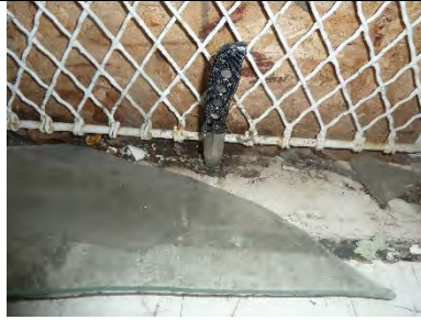
N241-02: View of rotted sill
