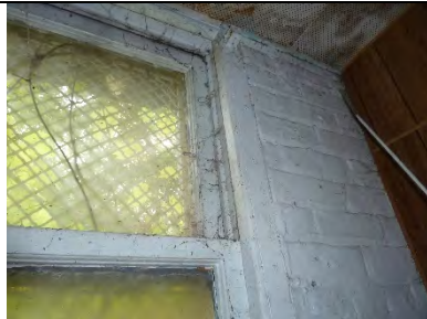
S102-02: Open corner at upper sash right
