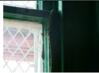
S337-03: Broken rope for weight
