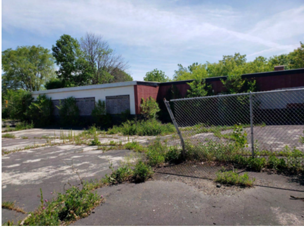
West Elevation of one story addition. (Partially obscured by vegetation.) Tags are W120-W123
