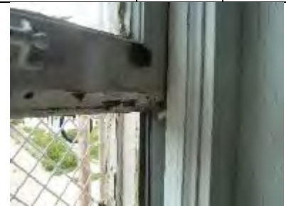
W311-03: Rotted rail of lower sash
