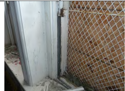
N218-03: Broken bottom rail
