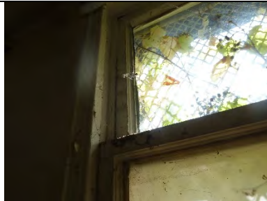
S108-02: Lower right corner of upper sash broken
