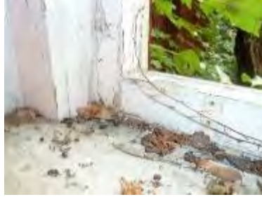
LC323-02: Damage along lower rail
