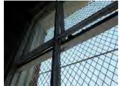
N302-03: Damage at meeting rail
