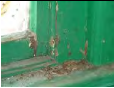
S337-02: Damage on interior sill & trim
