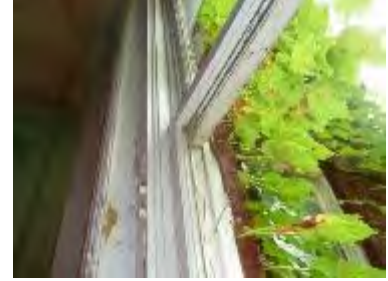
LC323-03: Jamb & meeting rail condition
