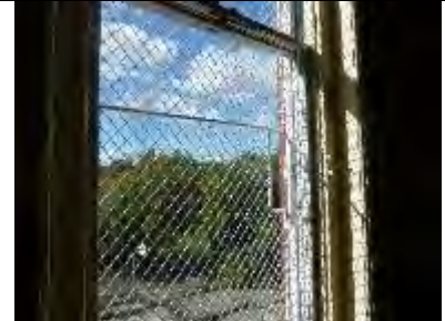
S323-03: Missing muntins on lower sash
