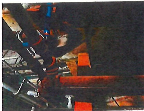
Photo #3 – Joists cut for plumbing
