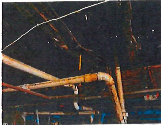
Photo #4 – Rotted &/or fire damaged joists
