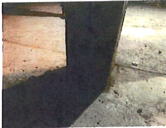
Photo #2 – Base rot on column (only 1 column was observed to have this)
