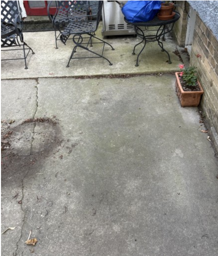
Cracked and settled rear patio to be replaced with stamped concrete patio
