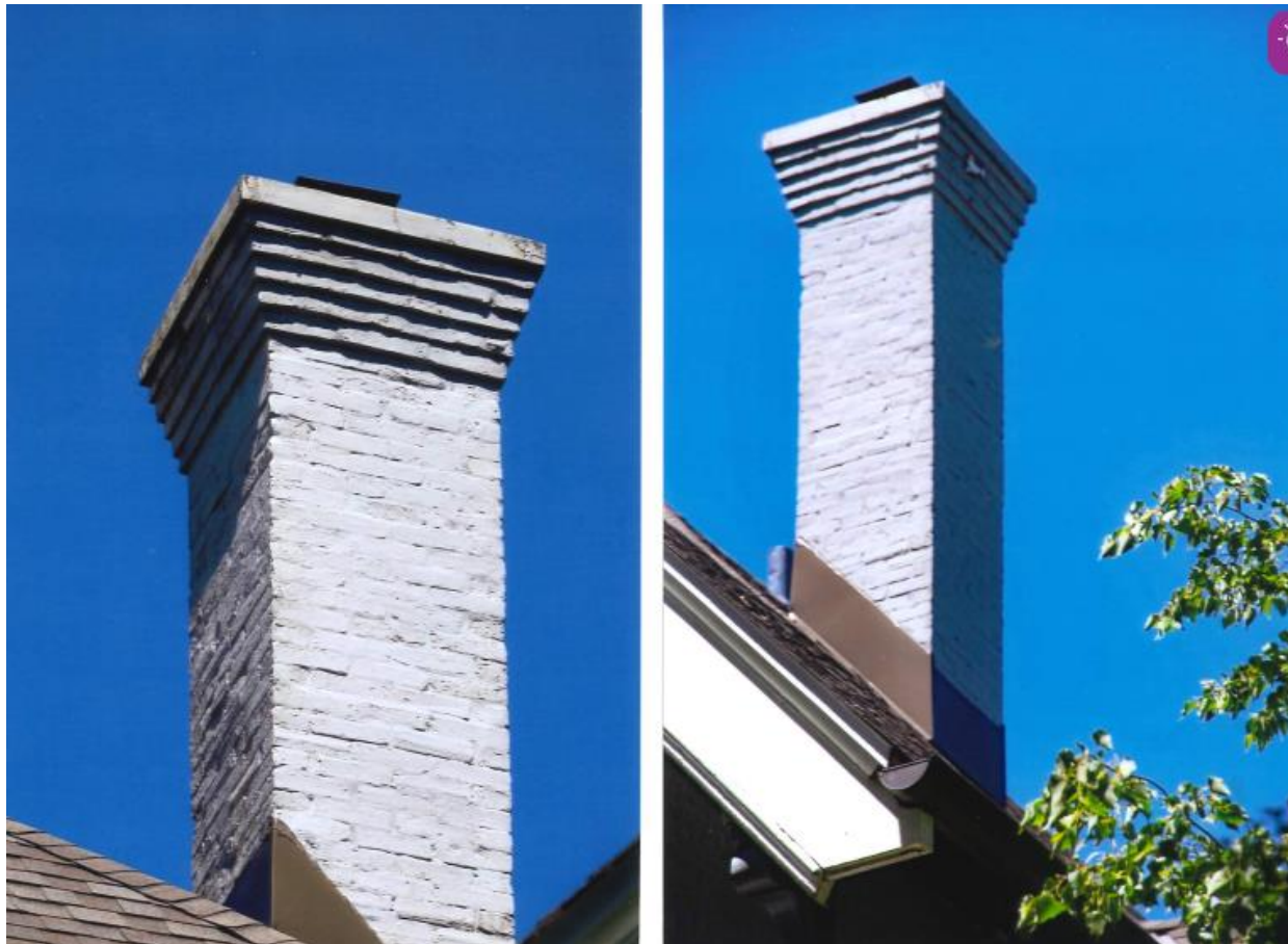
Chimney to be repaired
