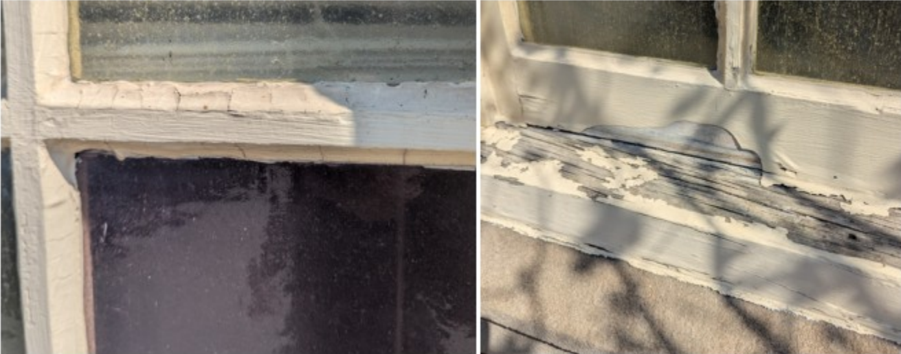
Close up of double hung windows needing repair
