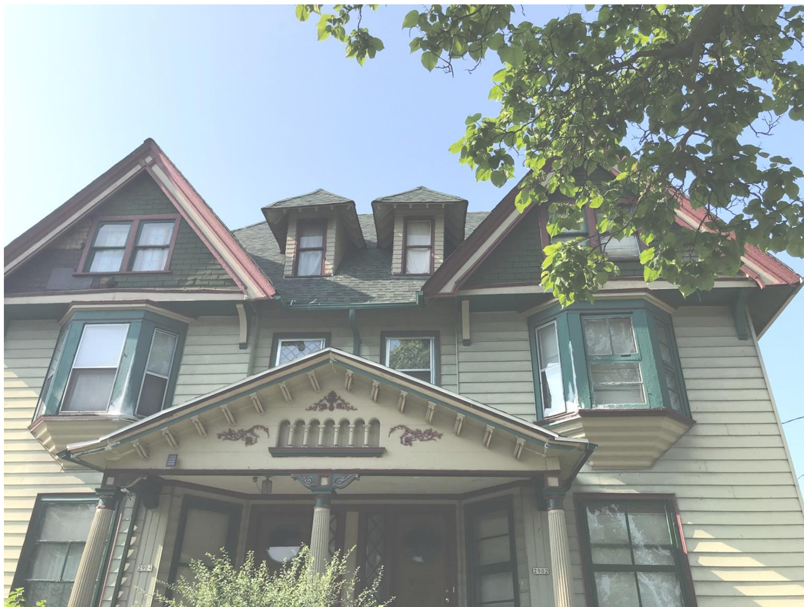
Current conditions at front showing roofing shingles used to clad the gable ends.
