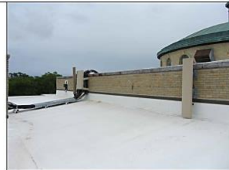
EXISTING T-MOBILE ANTENNAS - ALPHA SECTOR -
