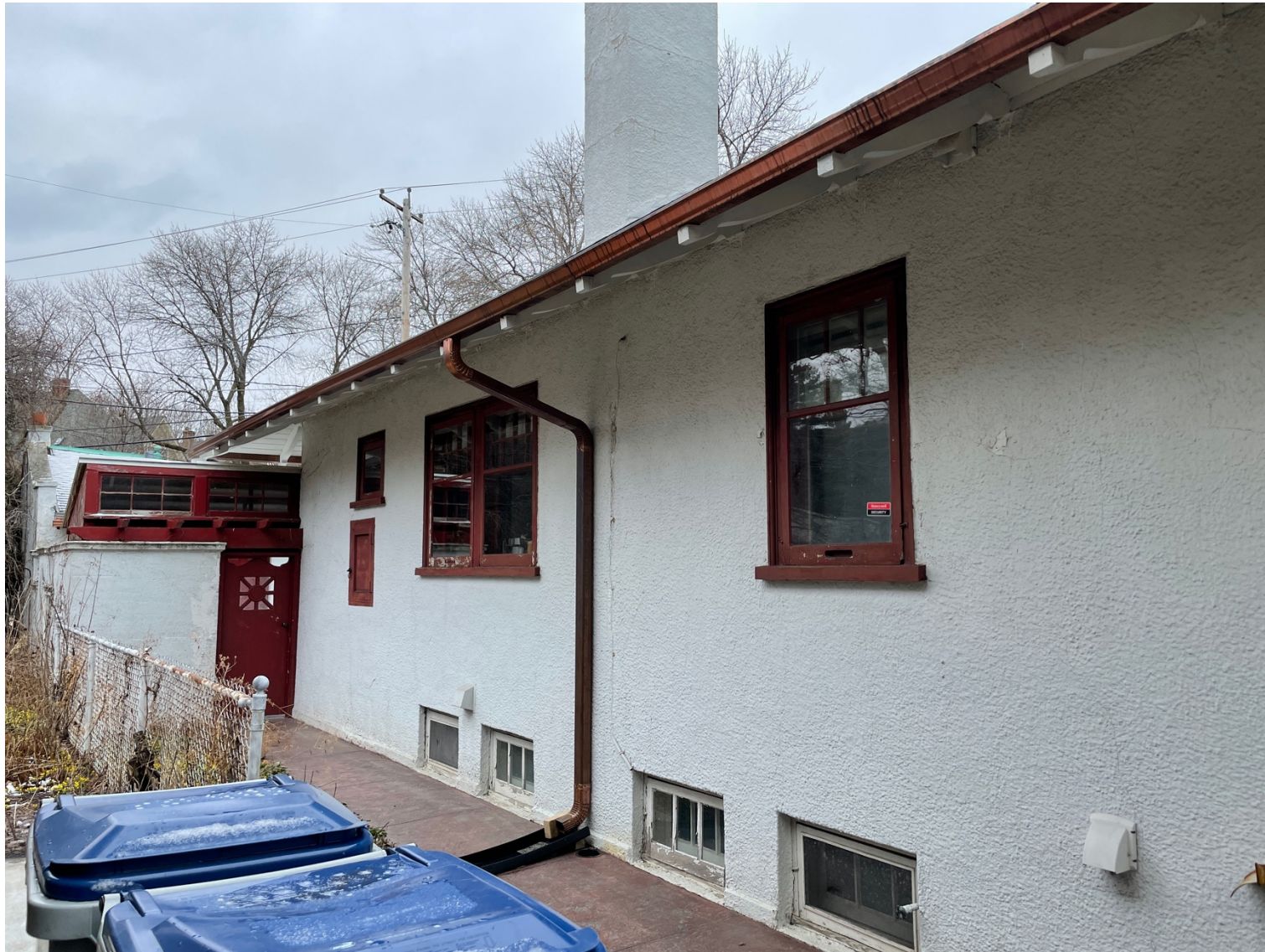
Photo 1: Existing exterior view looking towards pair of subject windows (to be shortened) and adjacent half window (to be removed and replaced with window that matches existing pair)
