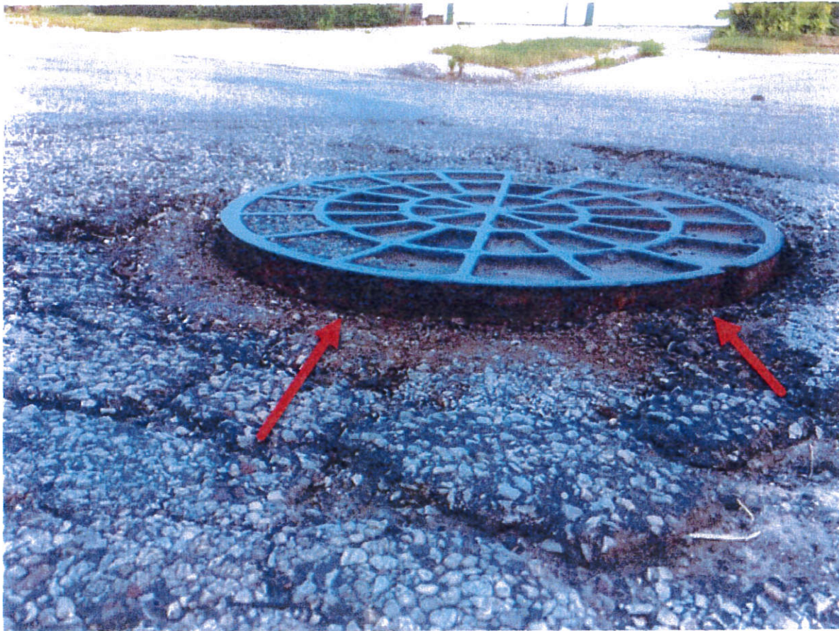
Manhole cover today (approx. 2200 E Ohio Ave.). Note still not sitting flush with street. Large 'lip' visible.
