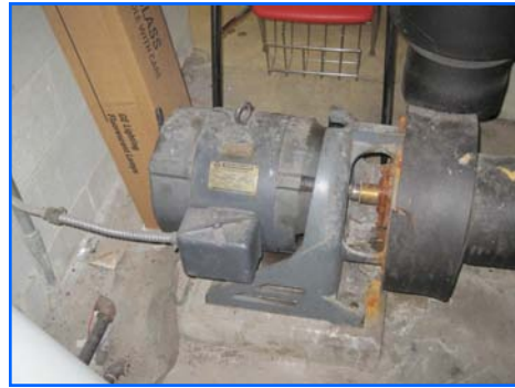
Domestic water pump
