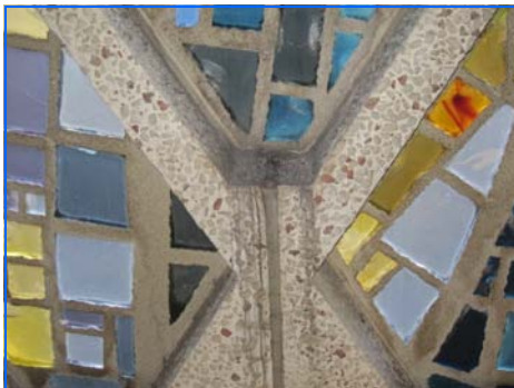
Evidence of leaks
