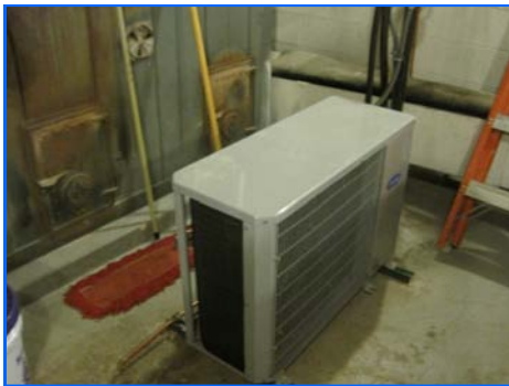
Elevator condensing unit
