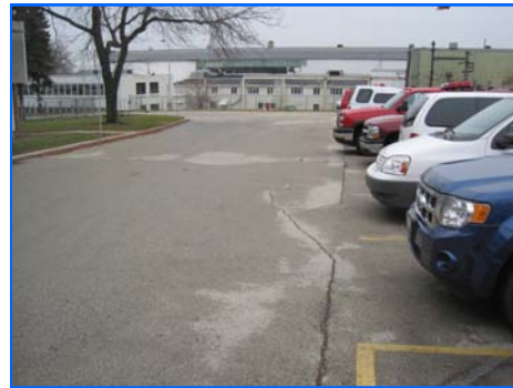
Asphalt pavement with longitudinal crack
