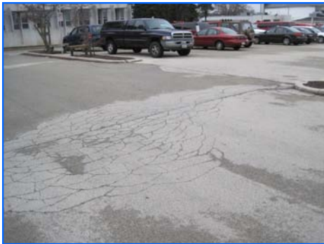
Asphalt pavement with alligator cracks
