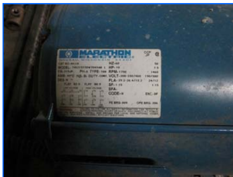
AHU motor - interim replacements and repairs funded by O+M
