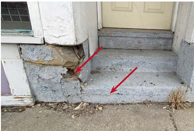
IMAGE 3: Area of impact damage and cracking at east elevation.
