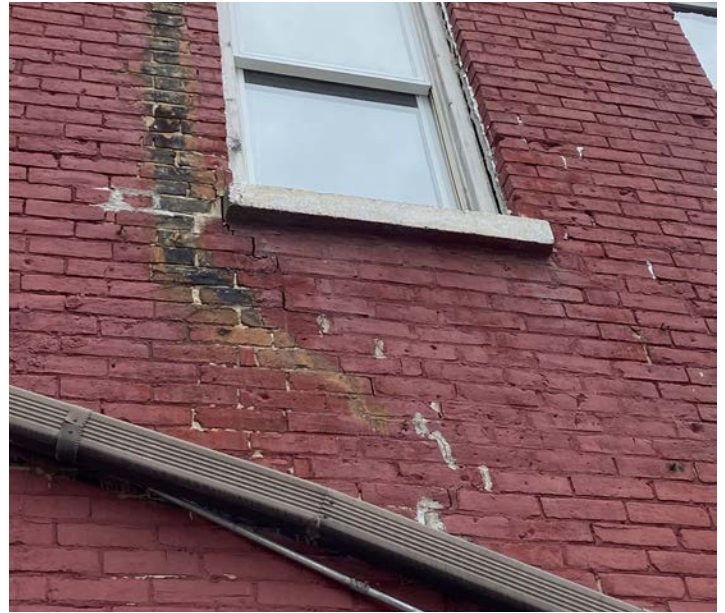
IMAGE 10: Area to be rebuilt below center second-floor window at the west elevation; large step crack and exposure to moisture has resulted in dislodged brick.
