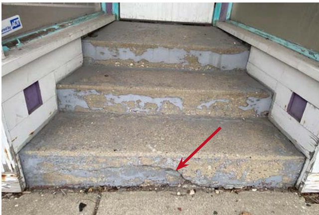
IMAGE 2: Crack at main entrance steps.
