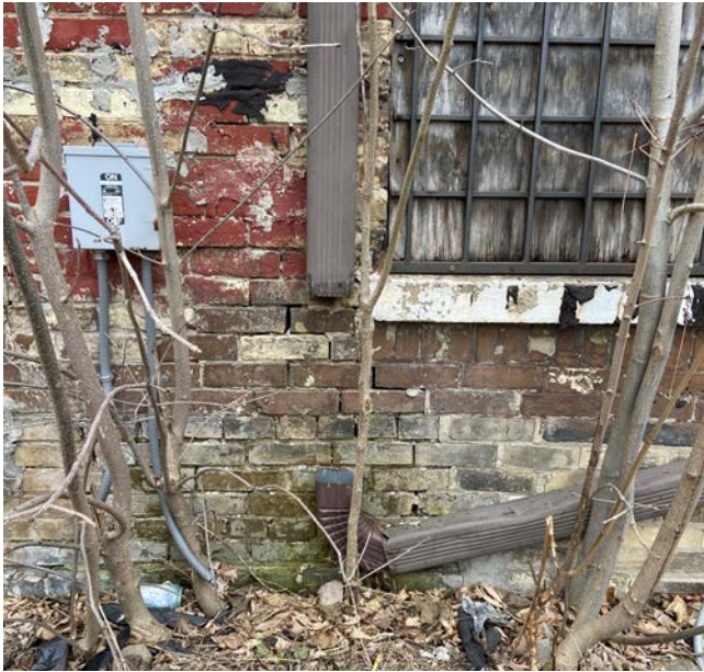
IMAGE 9: Disconnected downspouts and insufficient slope to drainage at rear west elevation near first-floor windows.
