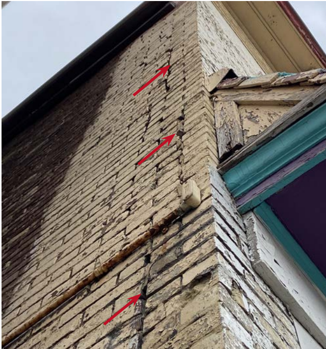
IMAGE 1: Crack at southeast corner showing signs of separation.
