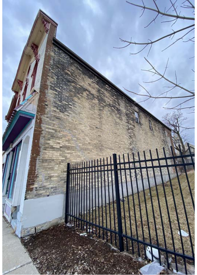
IMAGE 15: North elevation; here work is limited to masonry repairs and flashing at windows as described in the Scope Narrative.
