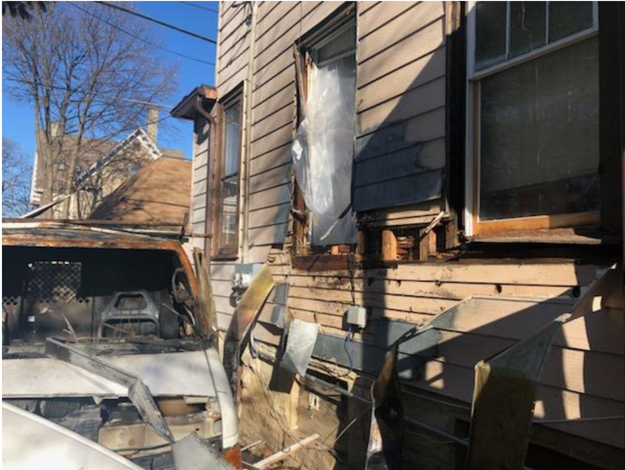
Photo of damage
