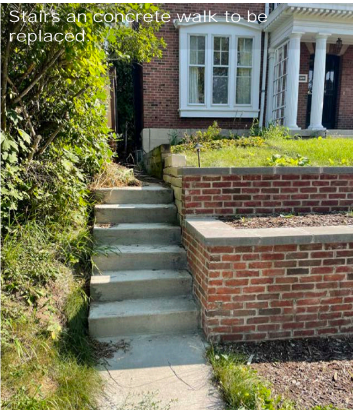
Stairs, masonry stone walls, and driveway to be replaced.
