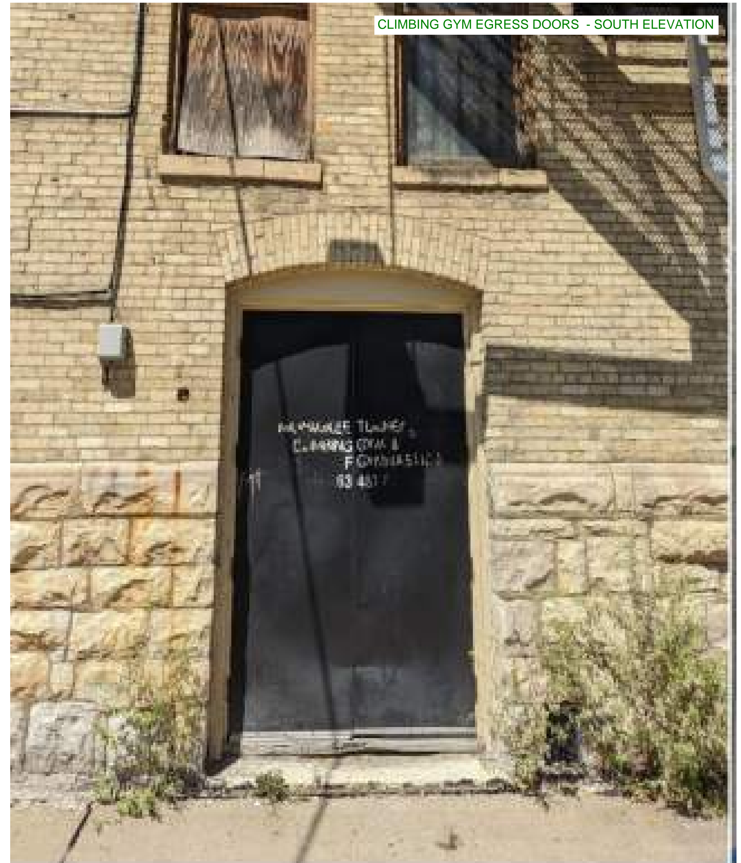
Non-original metal double doors in historic open. Historic opening to remain intact. New single panel metal double doors to be installed in existing opening. Original door configuration unknown.
