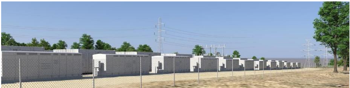
Figure 6 Constructed Battery Storage Facility
