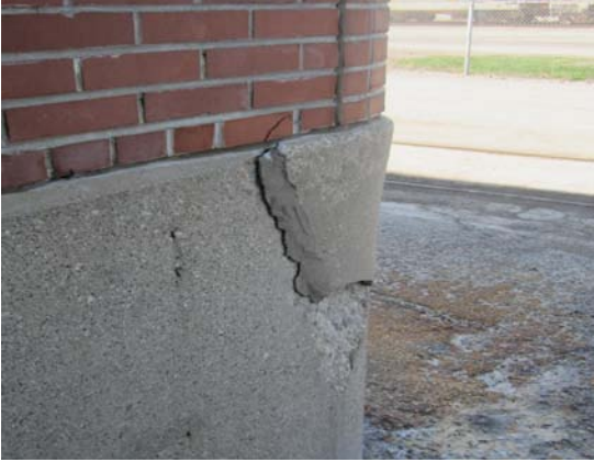
Spalled concrete at NW corner
