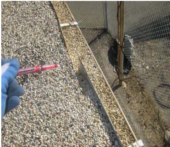
Roof-2 gutter is clogged full with gravel
