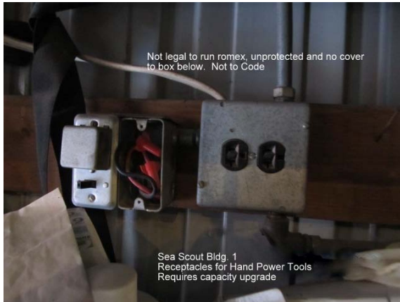
Code violation at Sea Scout 2
