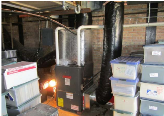
Interior forced air furnace
