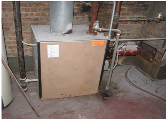
Building heat boiler
