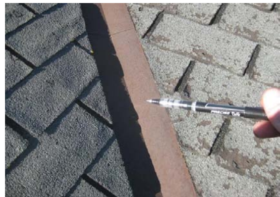
Valley flashings are rusting
