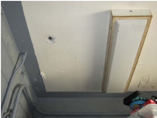
Hole in the ceiling and lighting fixture
