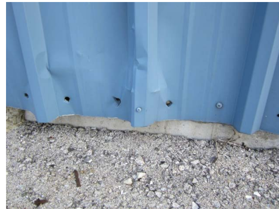
Missing fasteners west elevation
