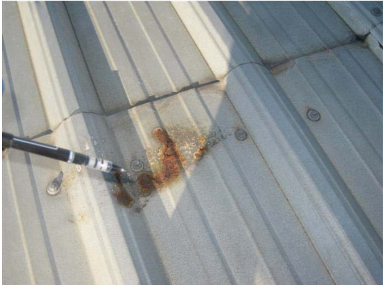
Rusted roof section – O+M repair
