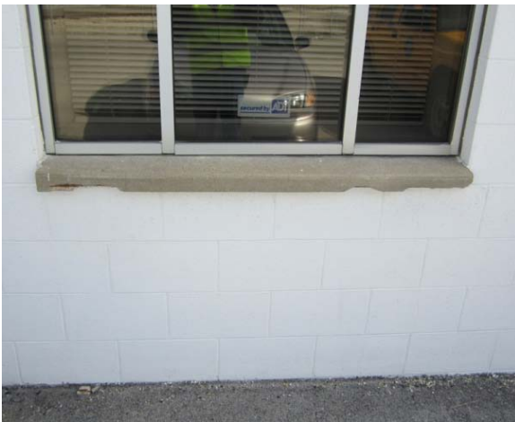
Damaged concrete sill
