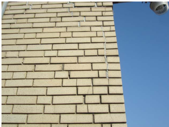
Cracked brick and sealant (not mortar) repair
