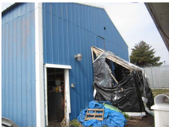
Rusted siding at SW elevation
