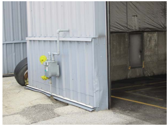
Damaged siding at doors at west elevation
