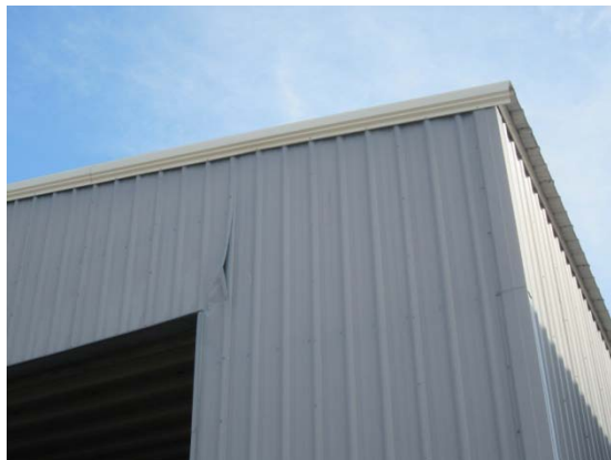
Damaged siding at west elevation
