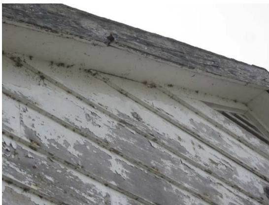
Paint finish deterioration and exposed/deteriorated wood siding
