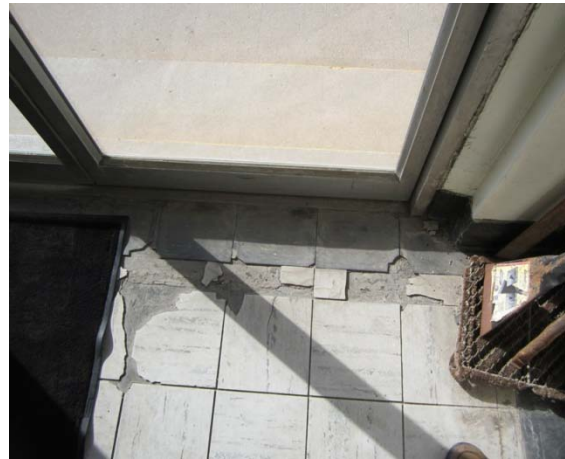
Damaged floor tiles
