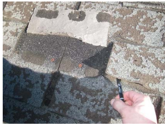
Roof Shingle deterioration
