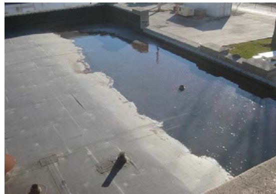
Ponding water R-1, drain stopped up
