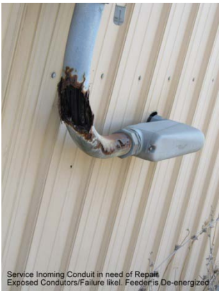
De-energized incoming service
