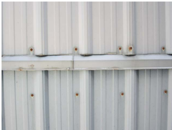
Rusted metal fasteners at siding
