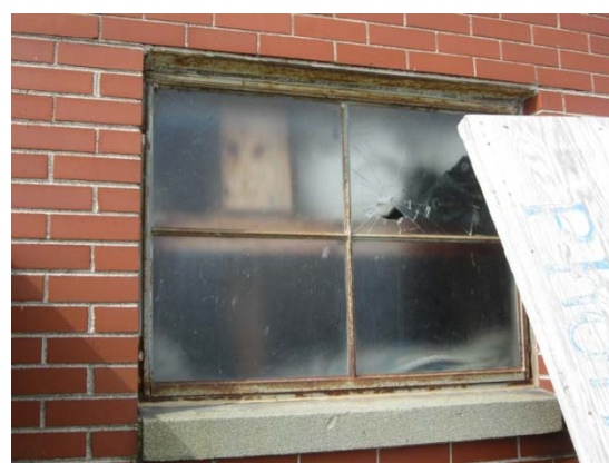
Broken window and rusted frame
