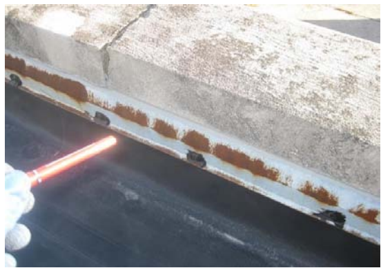
Counter flashing R-2 rusted
