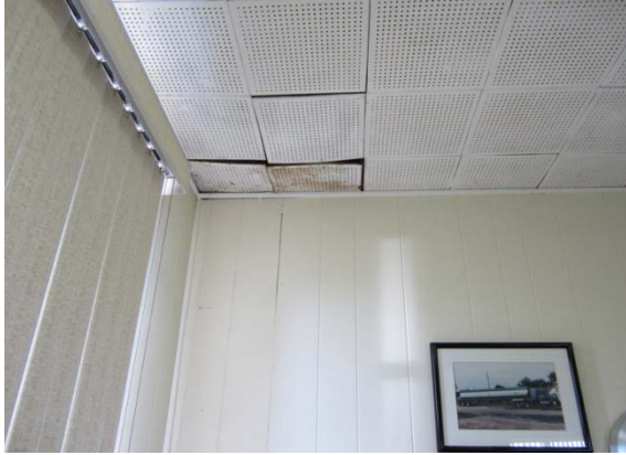
Ceiling water damage
