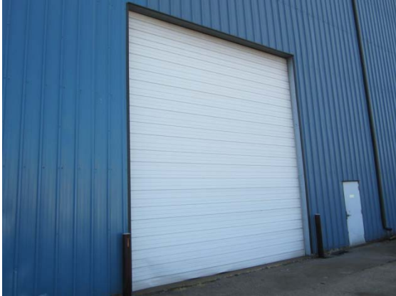
North overhead door with lower panel damage
