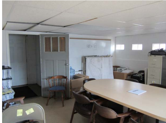
Acoustic ceiling tiles loose
