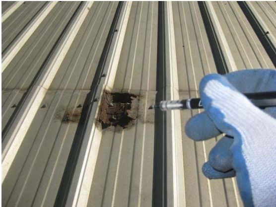
Rusted roof section – O+M repair
