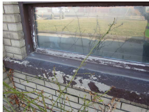
Paint finish deterioration at wood frame
