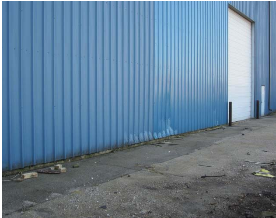
Damaged siding at north elevation
