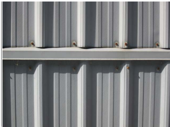
Rusted metal fasteners at siding
