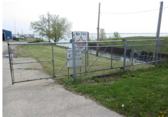
Gates and operators with some rust
