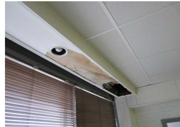
Ceiling water damage
