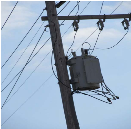
Main feeder transformer
