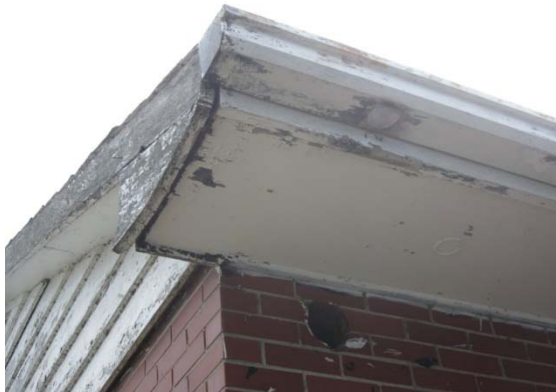
Gutters with no downspout
