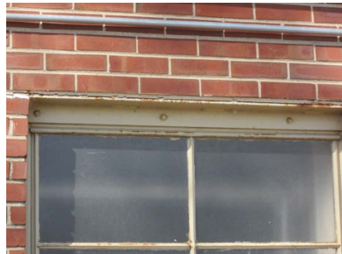
Onset of rust at window
