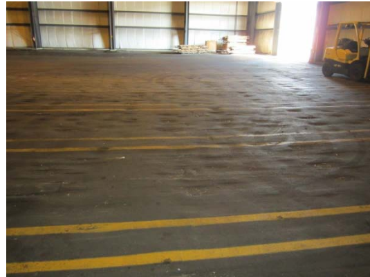
Asphalt pavement ruts and divots
