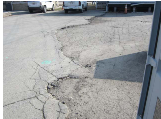
Serious erosion and uneven asphalt
