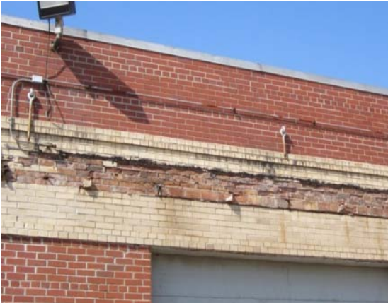
Unfinished masonry work at awning
