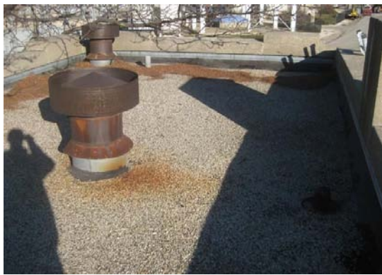
Tree debris on R-3 and gutters clogged
