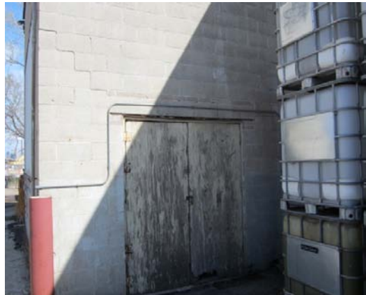
West service doors with deterioration
