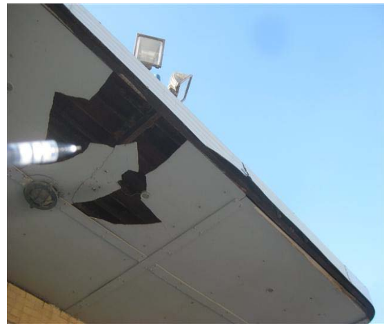
Roof-4 soffit from awning collapsing
