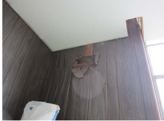
Damaged wall finish
