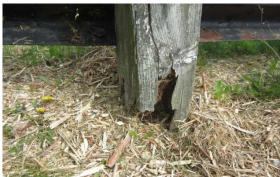
Deterioration at post
