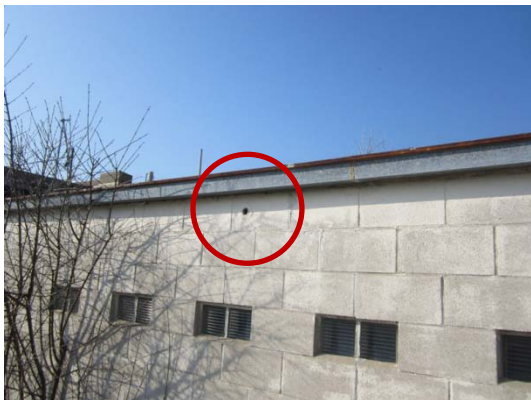
East elevation 2" hole in CMU
