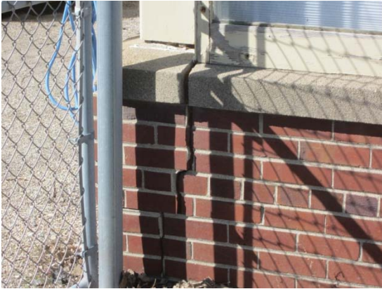
Cracked brick mortar at east elevation
