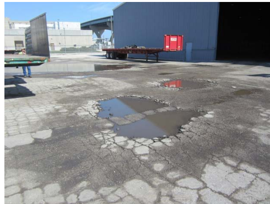
Large cracking and water pooling at the southwest entrance
