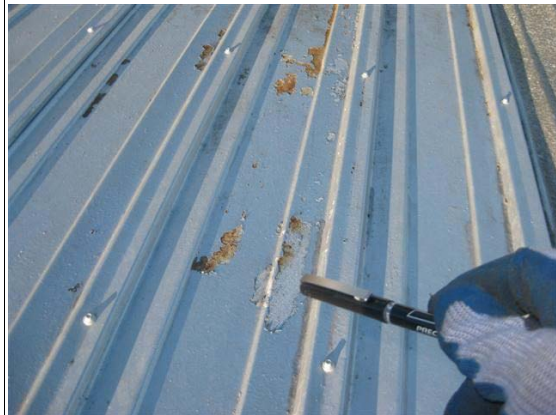
Damaged roof section
