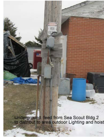
Underground utility meter
