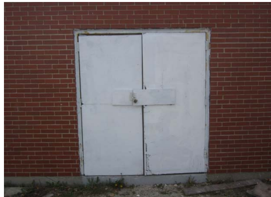
Damaged wooden doors
