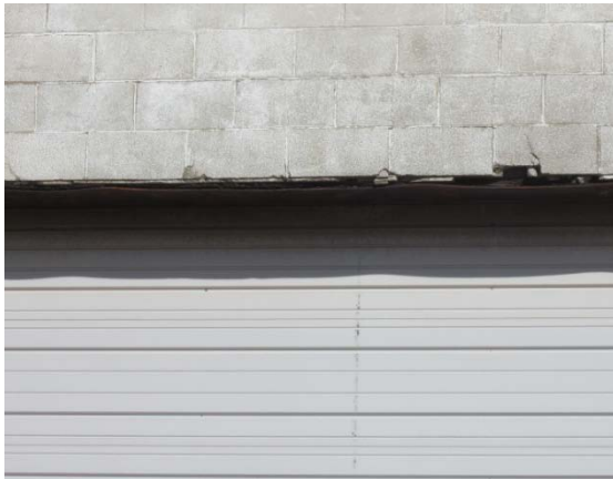
Deflected/damaged lintel and CMU
