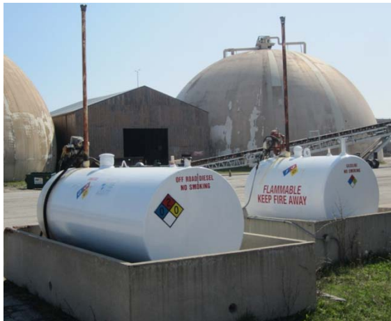
Fuel tanks and dispenser system
