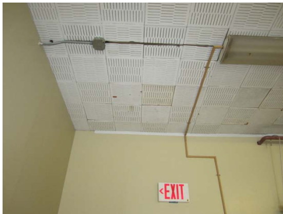
Emergency/Exit light fixture
