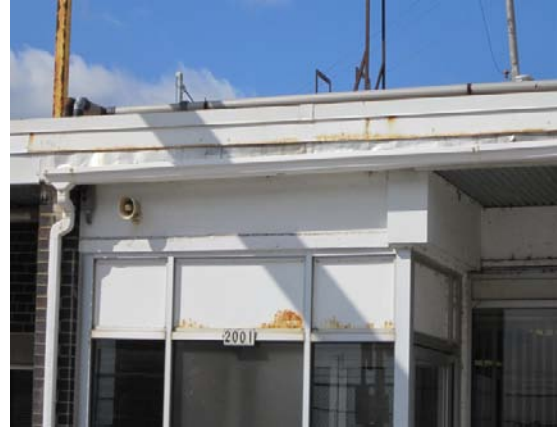
Rusting panels and facade
