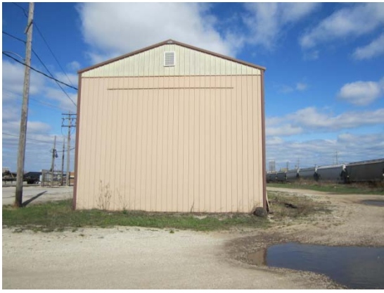
Rusted metal fasteners at siding
