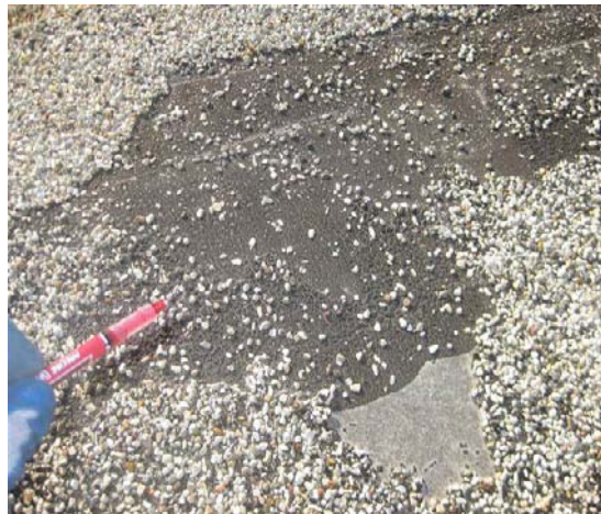
Roof-2 tar dry and cracking
