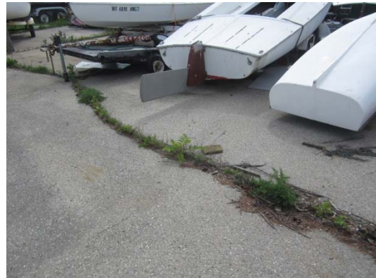
Large cracking and grass growing
