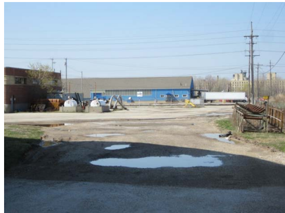
North cracking and potholes
