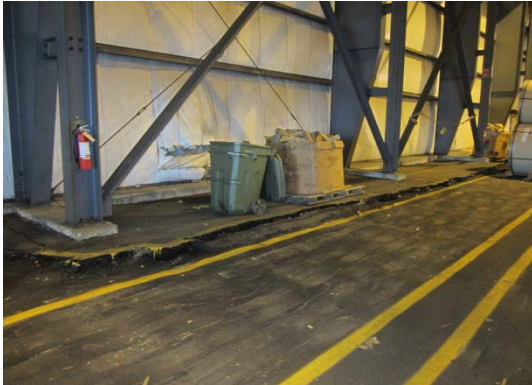
Sunken and rutted asphalt pavement
