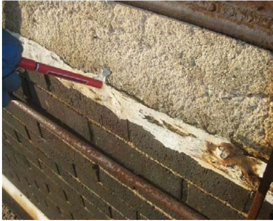
Roof-1 pan mastic is cracking
