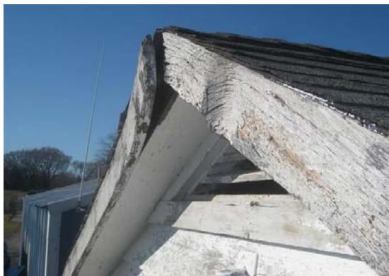
Wood fascia is weathered, damaged, and rotting
