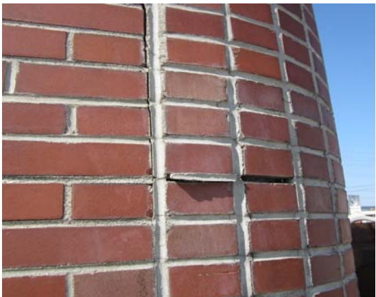
Mortar/brick separation at NE corner
