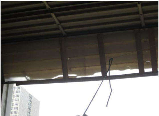
Overhead door with fiberglass damage
