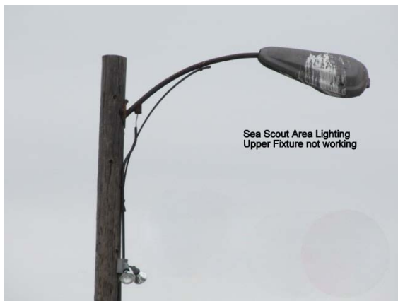
Non-functional light fixture
