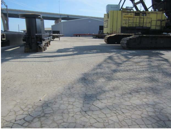
Severe cracking asphalt pavement
