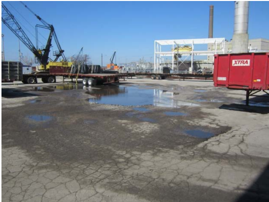
Water pooling & failed pavement
