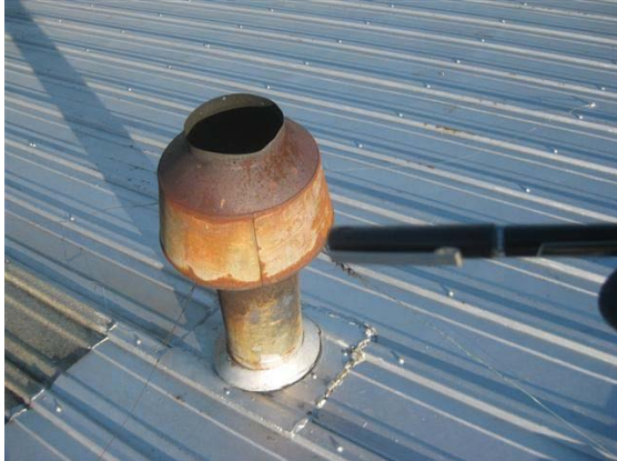
Rusted heater vent
