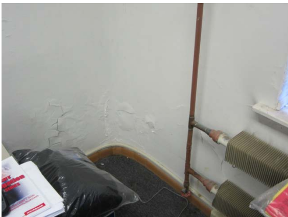
Damaged wall finish
