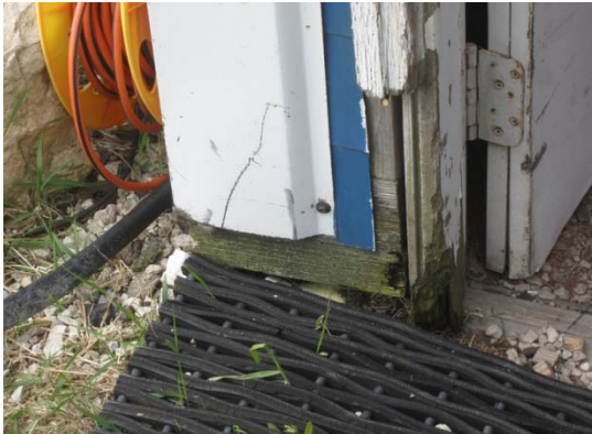
Door with lower door frame damage
