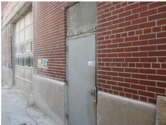
Onset of rust at west door
