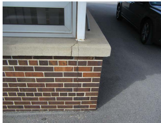
Cracked brick and sill at SE corner
