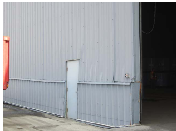
Damaged siding at doors at west elevation
