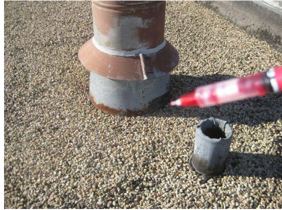
Roof-2 metal penetration rust
