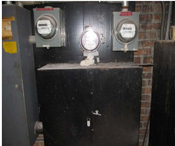
Incoming service with revenue meter
