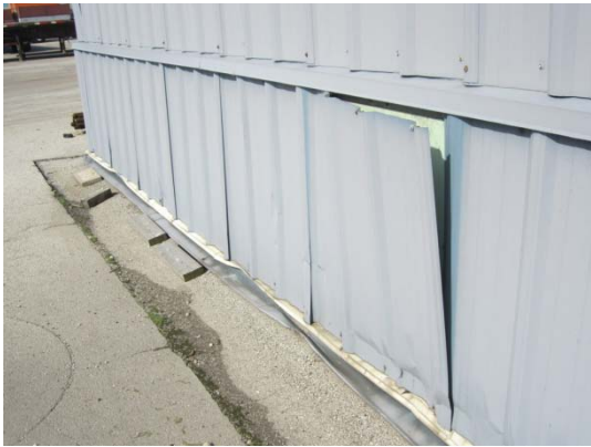
Damaged siding at south elevation
