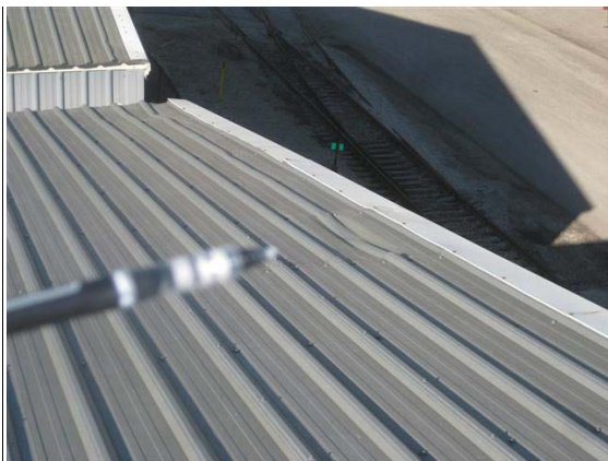
Damaged roof section
