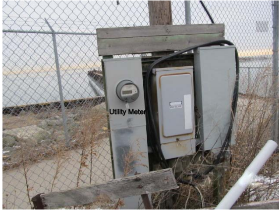
Secondary distribution and utility meter
