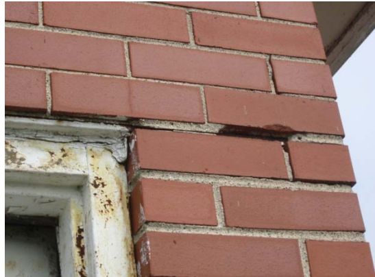
Cracked brick mortar at east elevation
