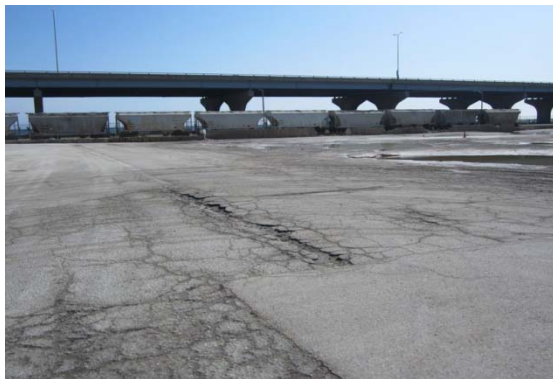
Alligator cracks and prior repairs
