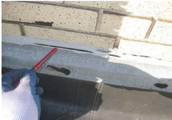
Flashing sealants for R-1 is cracking
