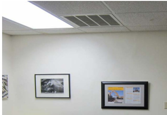
Unit-2 return air and evaporator
