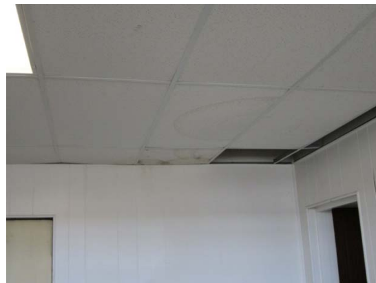
Stained and missing ceiling tiles
