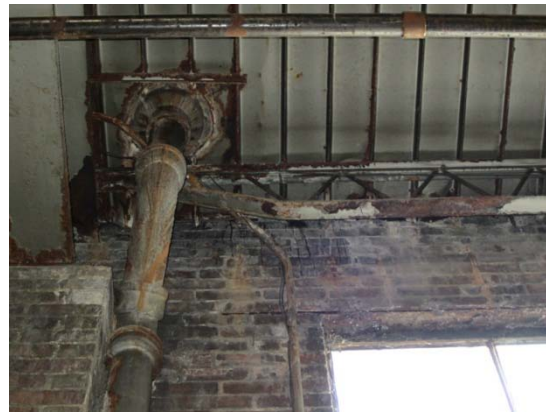
Rusted steel components
