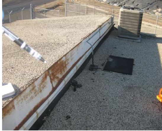
Roof-2 edge metals rusting
