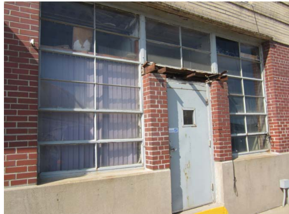
Onset of rust at east door
