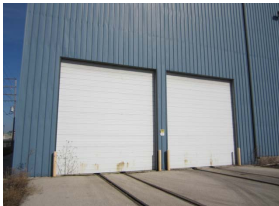
SW overhead door rusted lower panels
