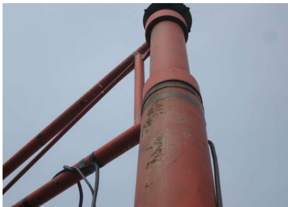
Onset of rust
