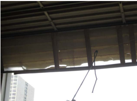
Overhead door with fiberglass damage
