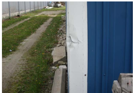
Damaged siding NW corner
