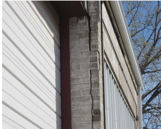
Cracked brick at south elevation
