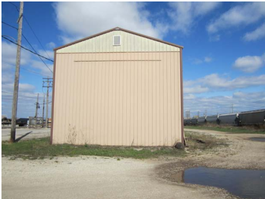
Rusted metal fasteners at siding
