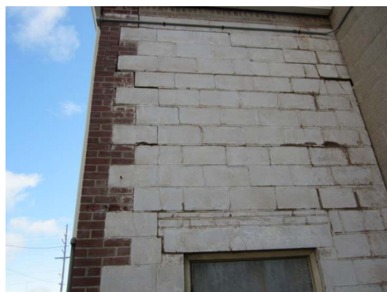
CMU and brick step cracking
