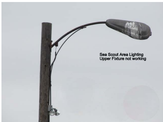
Non-functional light fixture
