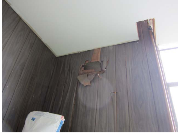
Damaged wall finish
