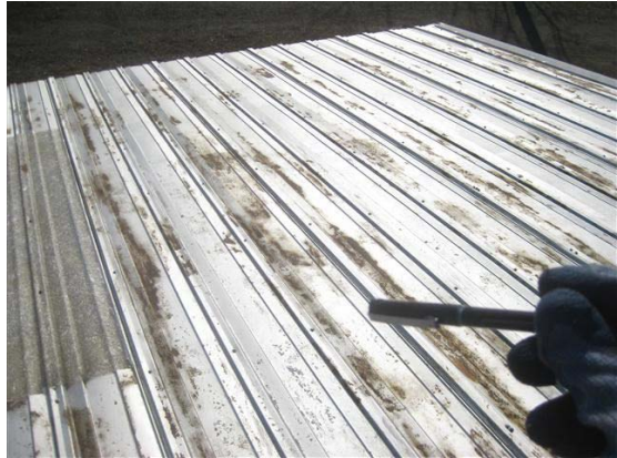
Rusted roof section
