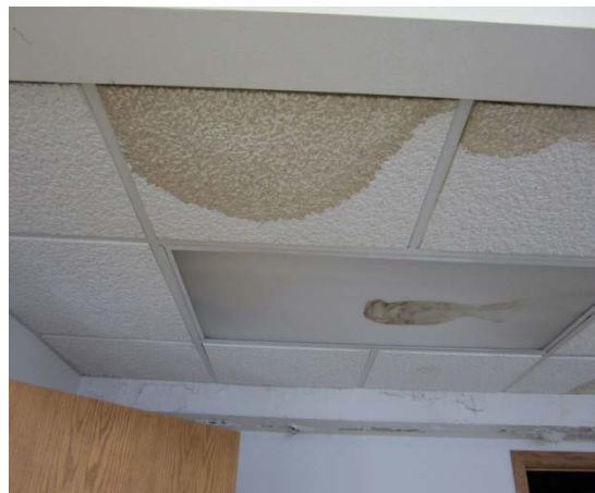
Ceiling tiles with water damage
