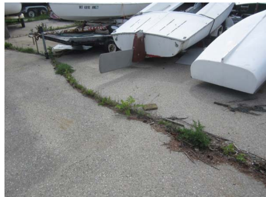
Large cracking and grass growing
