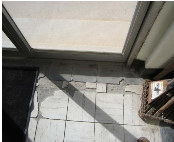
Damaged floor tiles
