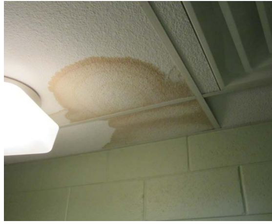
Water damaged ceiling tile
