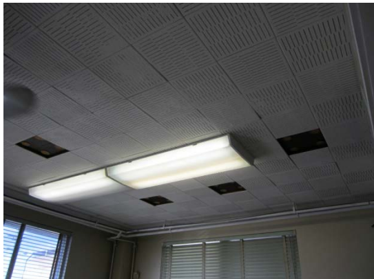
Fluorescent light fixtures
