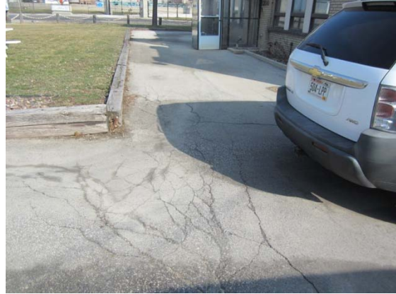
Front entrance asphalt cracking
