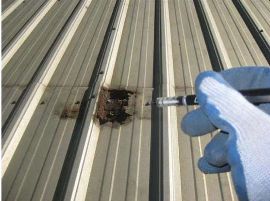
Rusted roof section – O+M repair
