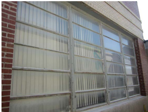
Window at southwest elevation with reported leaks
