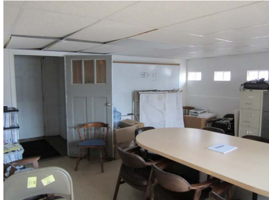
Acoustic ceiling tiles loose
