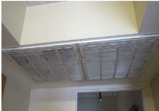
Unit-1 return air and evaporator
