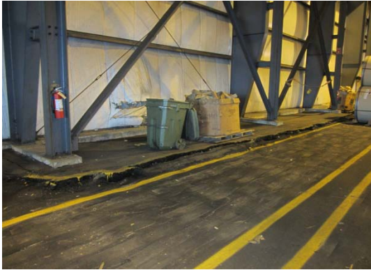
Sunken and rutted asphalt pavement
