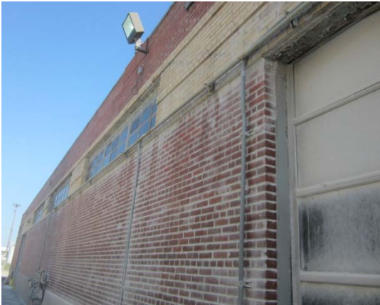
West elevation rusting lintels
