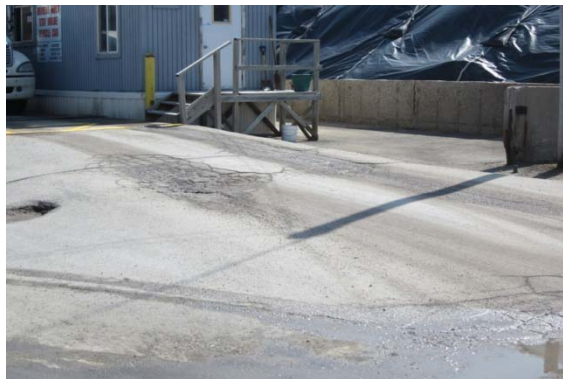
Longitudinal cracking near scale house
