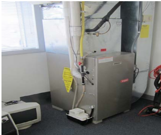
Furnace heating unit
