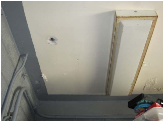
Hole in the ceiling and lighting fixture
