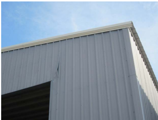
Damaged siding at west elevation
