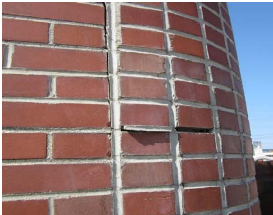
Mortar/brick separation at NE corner
