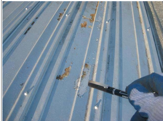
Damaged roof section
