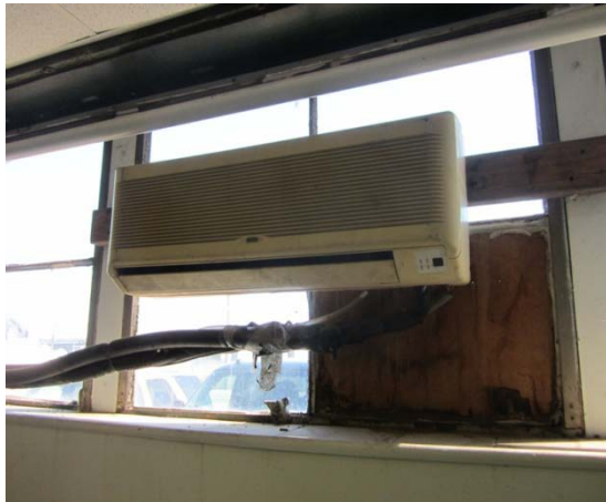
Air Conditioner unit
