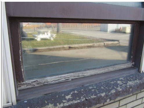
Paint finish deterioration at wood frame
