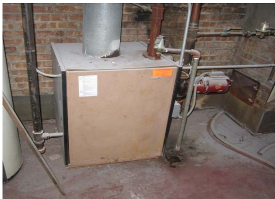
Building heat boiler
