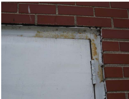
Displaced door frame caulking
