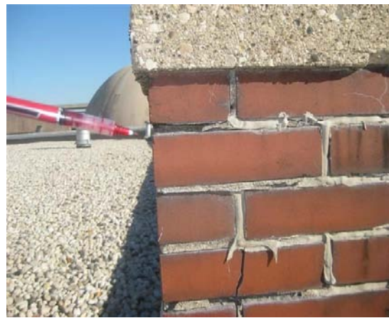
Roof-1 parapet deterioration
