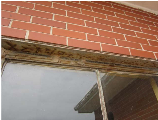
Rusted window lintel
