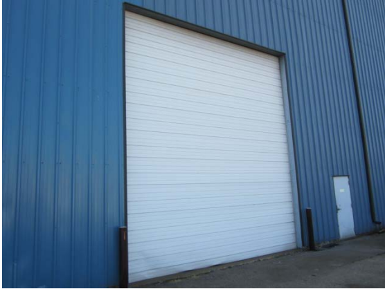
North overhead door with lower panel damage
