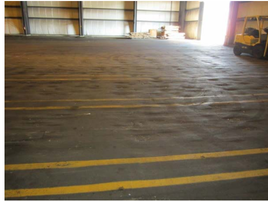
Asphalt pavement ruts and divots
