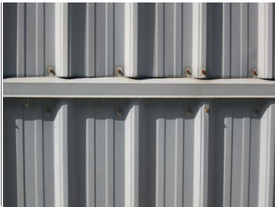
Rusted metal fasteners at siding
