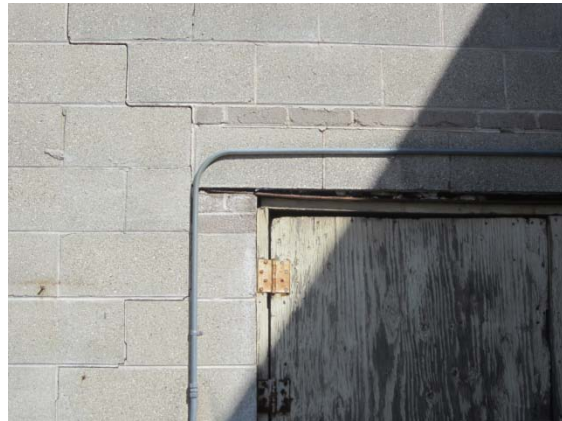
Step crack and lintel deflection
