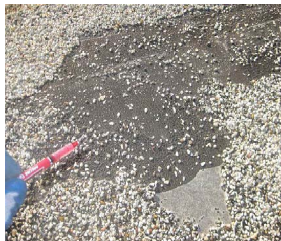
Roof-2 tar dry and cracking
