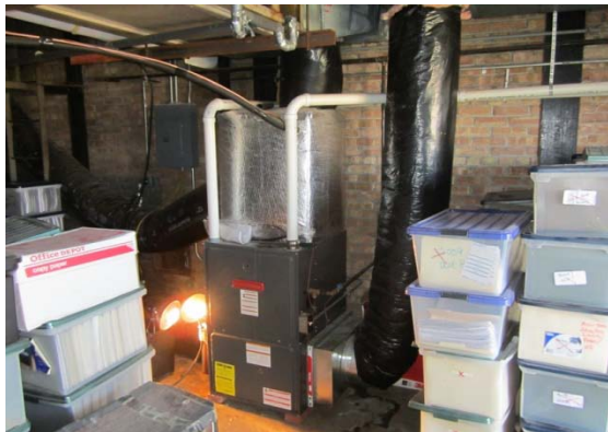
Interior forced air furnace
