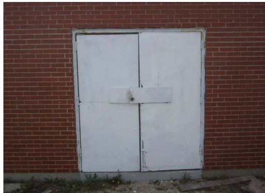
Damaged wooden doors
