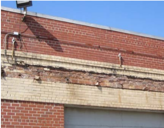
Unfinished masonry work at awning
