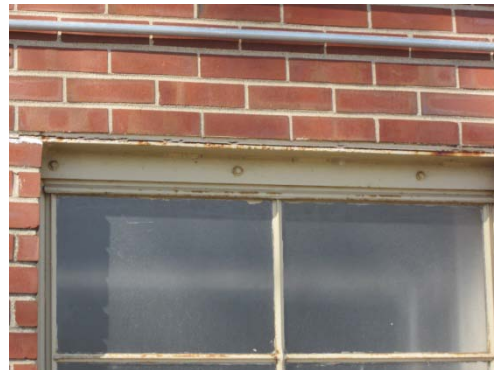
Onset of rust at window
