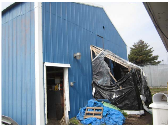
Rusted siding at SW elevation
