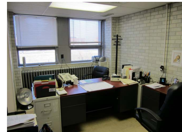
Office with abandon radiator
