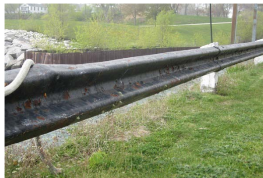
Guard rail rusting and dented
