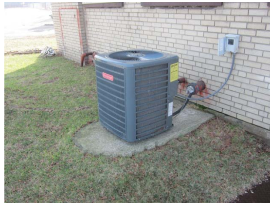
Air Conditioner unit
