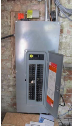
Main service panel
