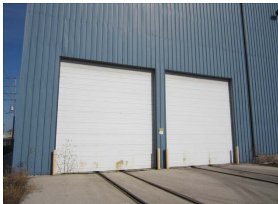
SW overhead door rusted lower panels
