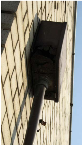
Weathered exterior conduit
