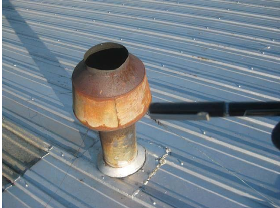
Rusted heater vent
