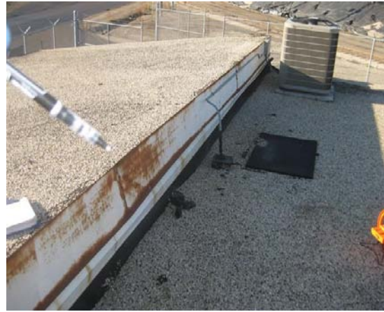
Roof-2 edge metals rusting
