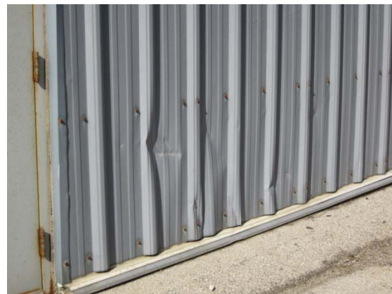
Damaged siding at east elevation
