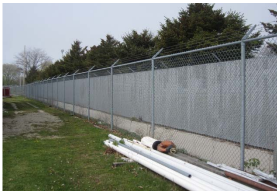
Rusted/Misaligned chain link fence
