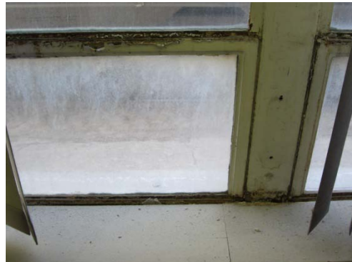
SW window rusted interior frame
