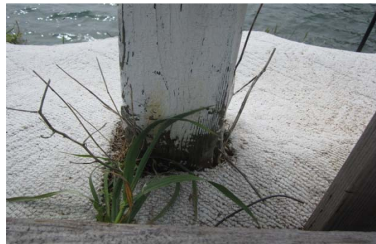
Paint finish deterioration at landscape line
