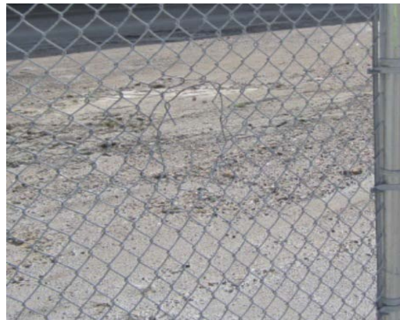
Damaged chain link section
