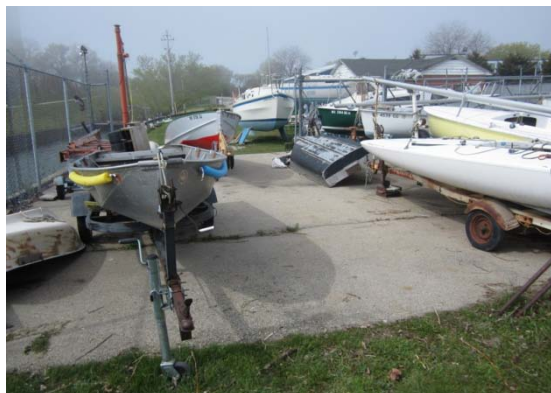
East elevation cracking asphalt pavement
