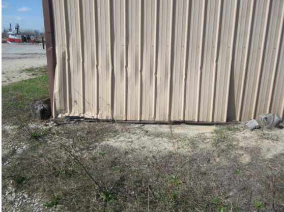
Damaged siding at east elevation
