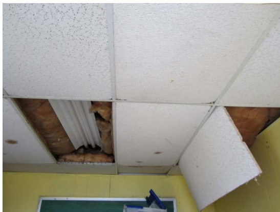
Acoustic ceiling tile missing
