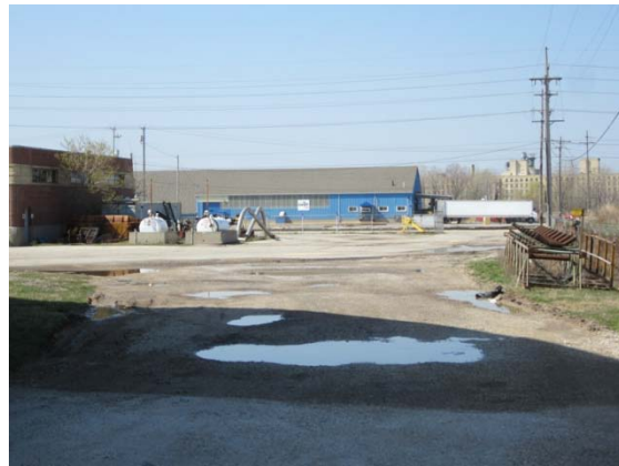
North cracking and potholes
