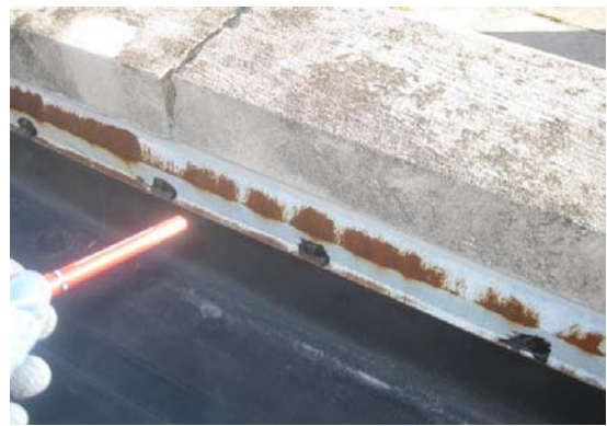
Counter flashing R-2 rusted
