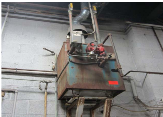
Building heat boiler
