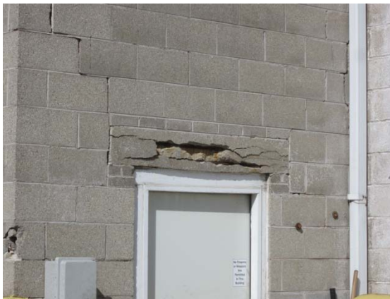
Deteriorated lintel at south elevation
