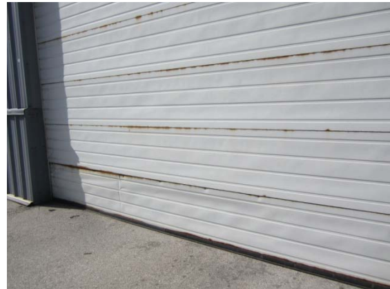
East overhead door with damage and rust
