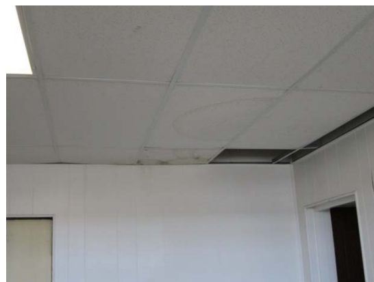
Stained and missing ceiling tiles
