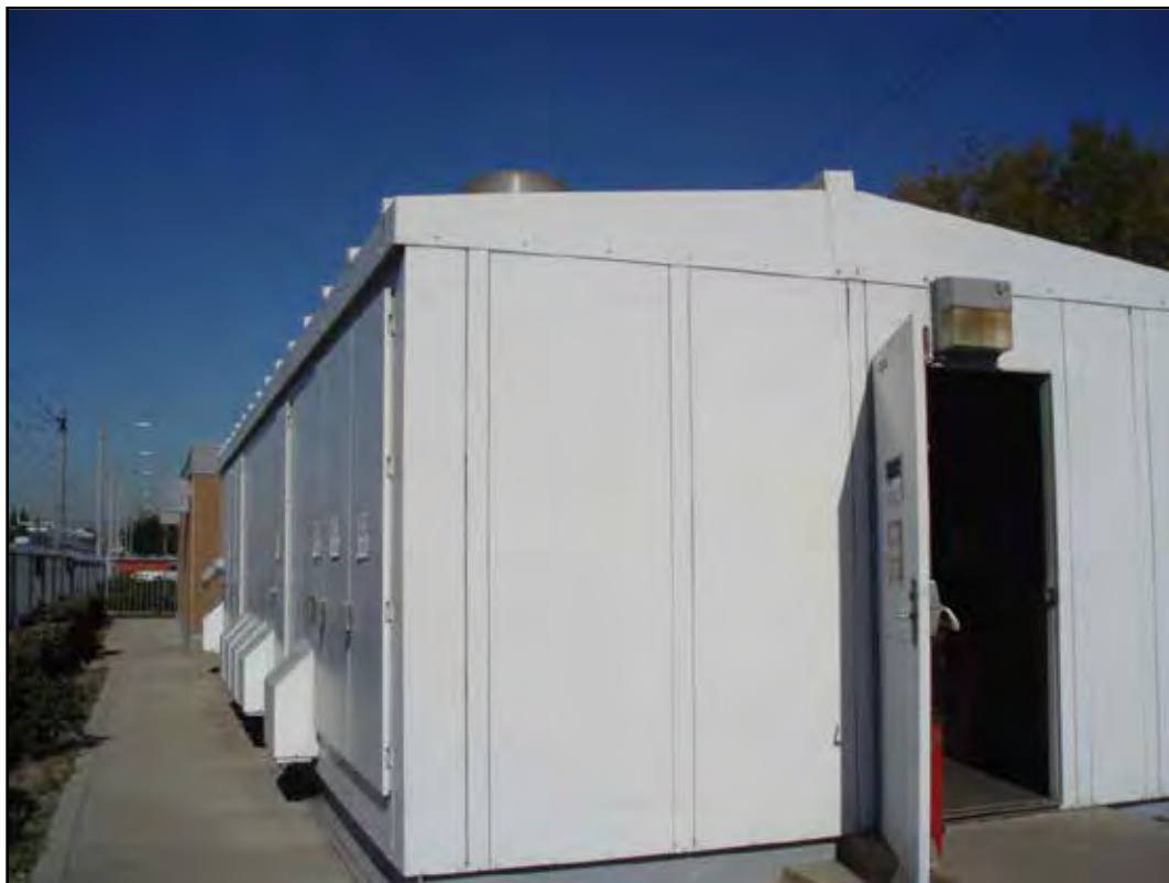
Figure 37: Example Photo of a Power Substation
