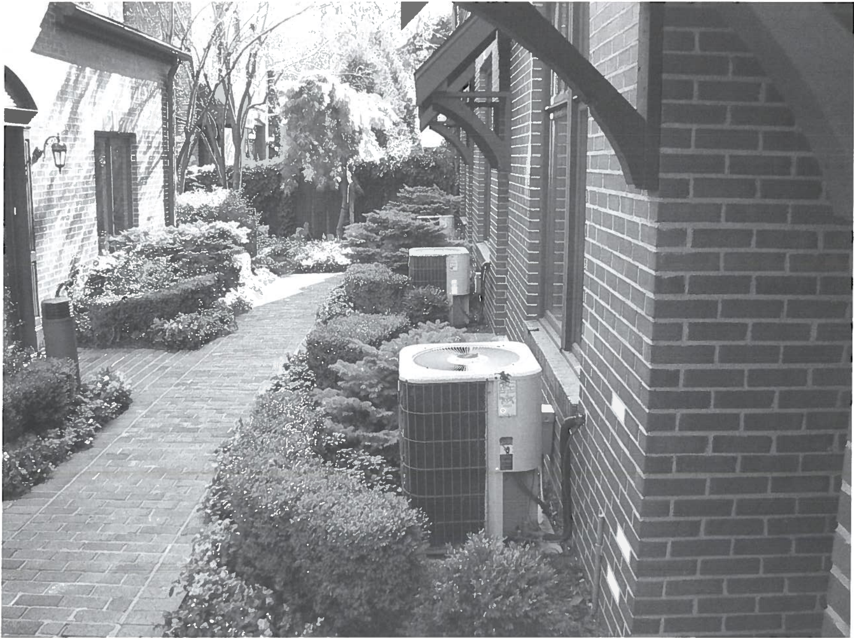
Replace AC unit, middle unit as shown in this image. New unit to be of similar size and configuration.
