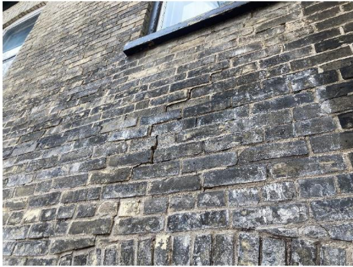
Section above shows signs of delamination. Portion of wall to be disassembled and rebuilt.
