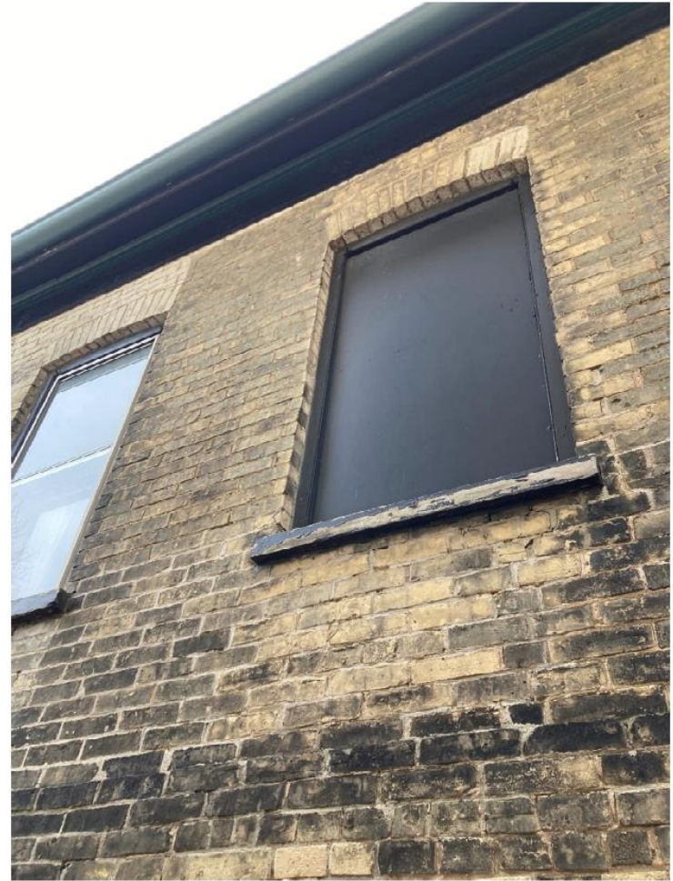
Wooden Sills to be replaced with Stone. Closed Window to be opened. New window to be installed. (North Face)
