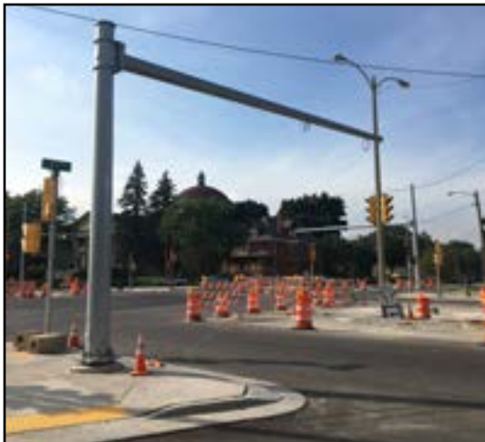
Current monotube installed at the intersection of North 27th and Highland Avenue.
