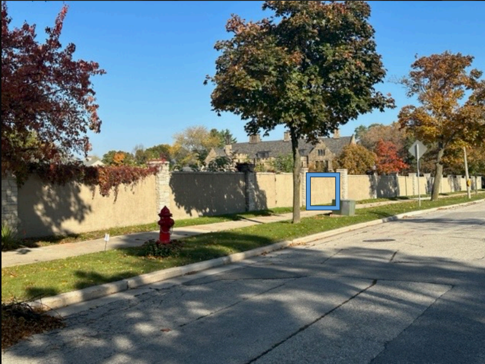
Northeast street view (Kenwood Blvd) of current wall. (proposed cut for driveway would be here)
