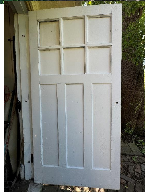
Garage to receive new roof, soffit and fascia repairs, new gutters, door repair, and removal of flat plywood on front of doors to expose historic door design.
