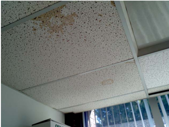
Stained ceiling tile
