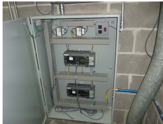
Building automation system monitoring devices
