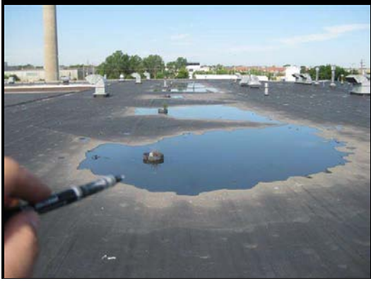
Ponded water at Lincoln Garage
