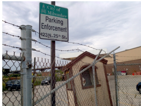
Damaged fence rail and barbed wire
