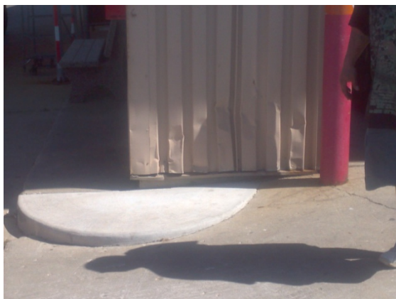
Damaged metal siding
