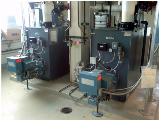
Building heat boilers
