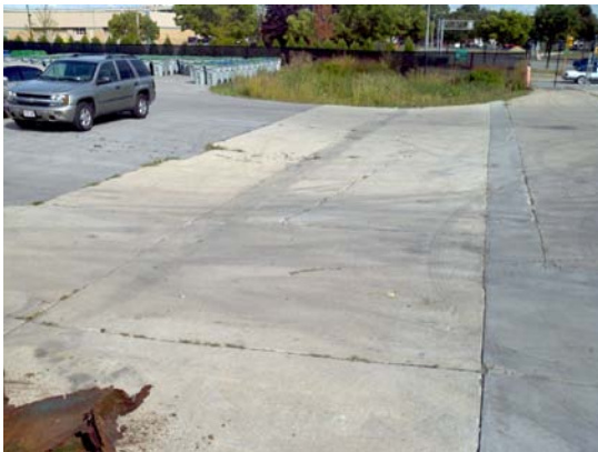
Cracked driveway near rain garden
