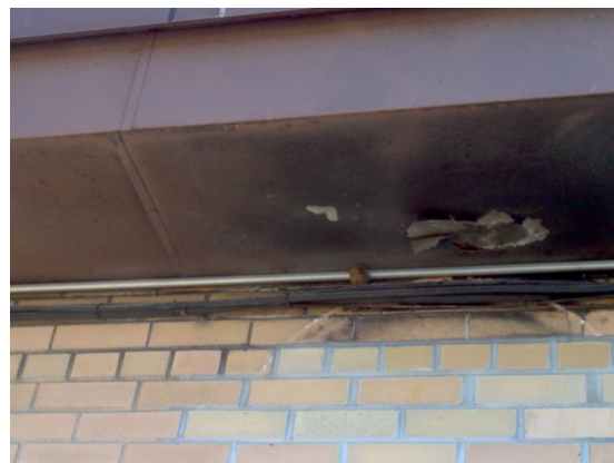
Damaged fascia at rear elevation
