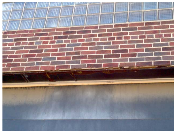
Rusted metal lintel at north elevation
