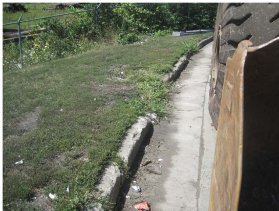
Deteriorated curb near Transfer Station
