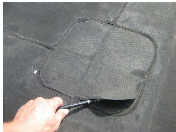
Loose patch at Lincoln Garage roof
