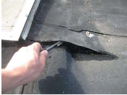
Split roof membrane at Lincoln Garage
