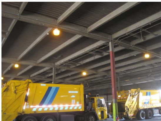
Typical Lincoln Garage light fixture
