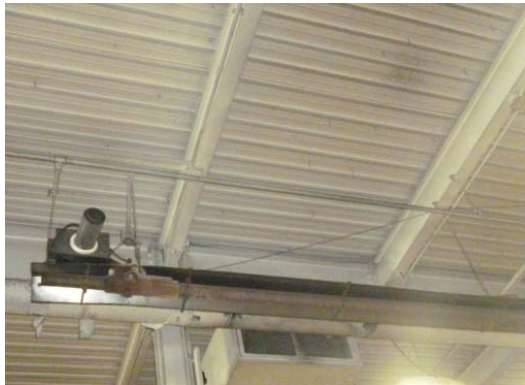
Rusted tube heater
