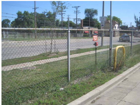
Chain link fence
