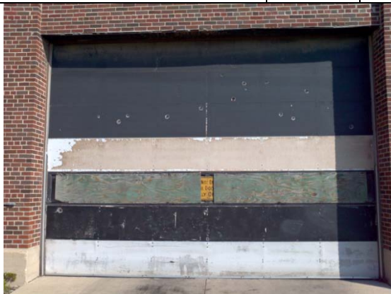
Garage door w repairs at Office Building
