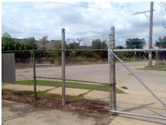
Rusted/damaged fence at adjacent lot
