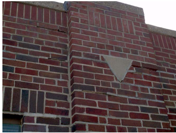
Mortar loss at west elevation
