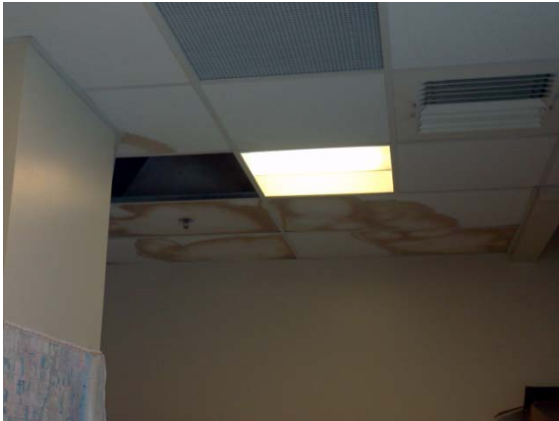
Stained ATC 2 nd floor southeast office
