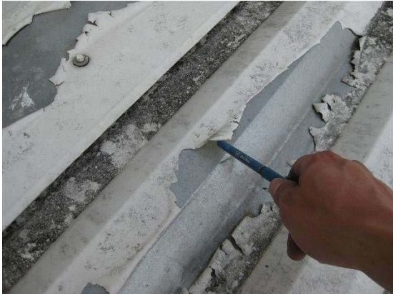
Delaminated surface coating
