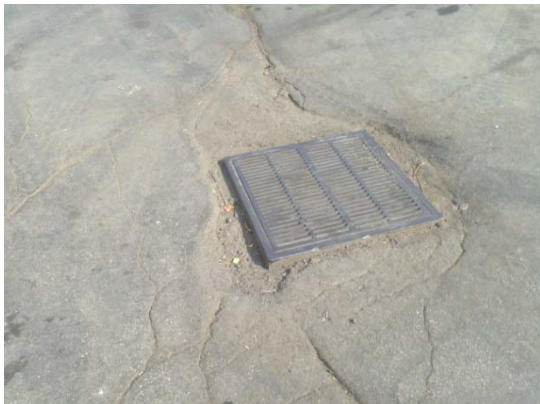
Settled catch basin
