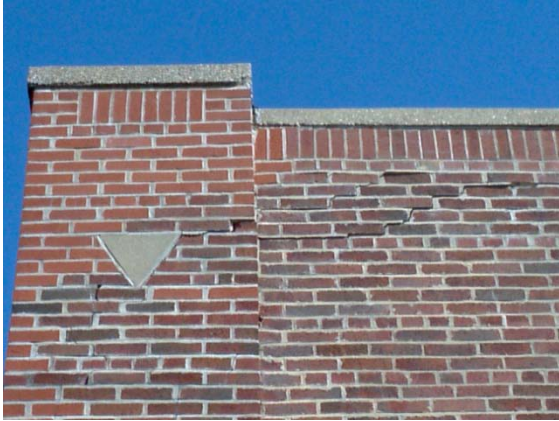
Mortar step crack at south elevation
