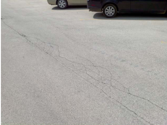
Alligator cracking/failed pavement
