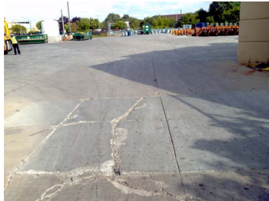
Cracked concrete at entrance drive
