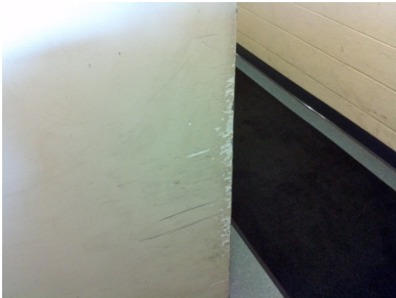
Damaged/begrimed wall finishes
