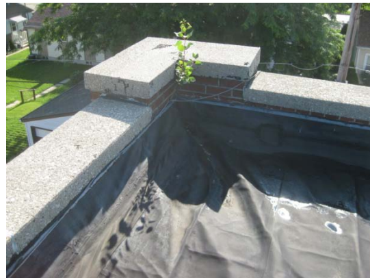
Roof #1 – delaminated membrane
