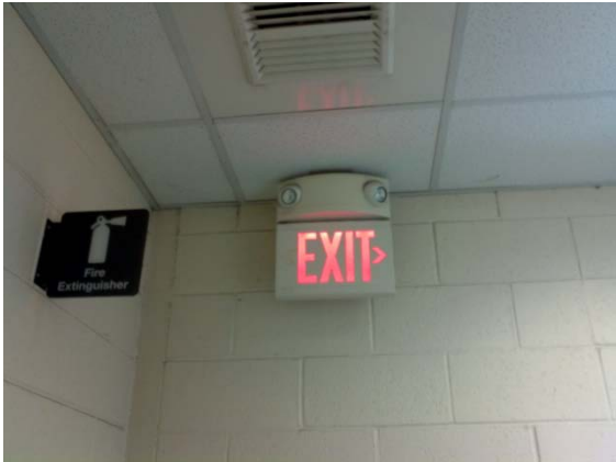
Emergency/Exit light fixture
