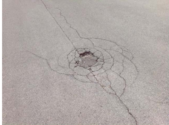
Failed pavement/pot hole
