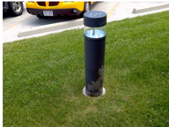
Bollard light w factory finish deterioration
