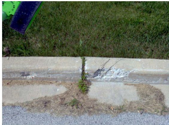
Damaged concrete curb
