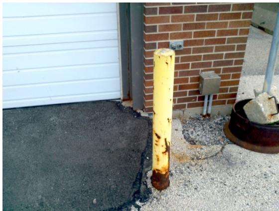
Typical rusted bollard
