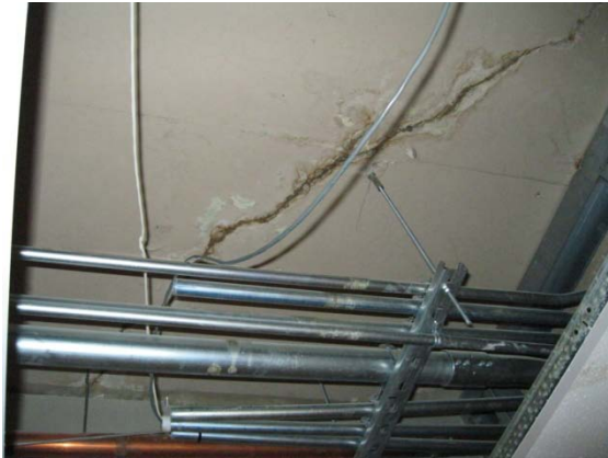
Roof deck underside is cracked and leaks
