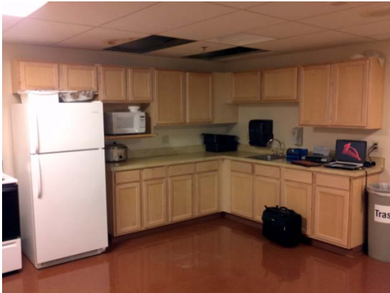
Third floor kitchen, note damaged ATC
