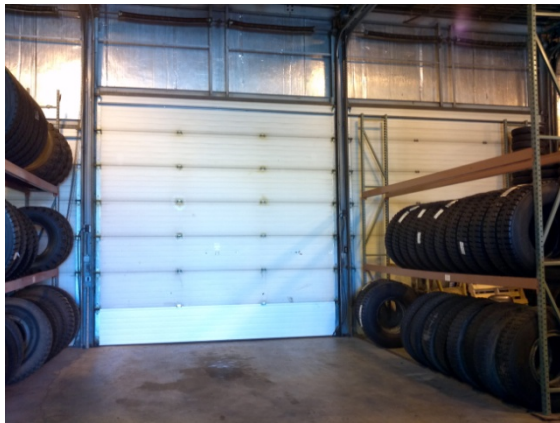
Garage door with replaced lower panel and rusted panel hinges
