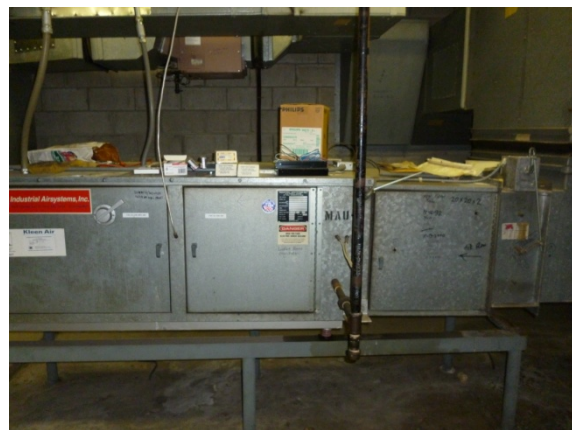
Storage room MAU
