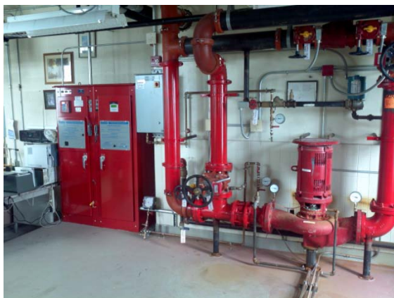
Fire control equipment and pump
