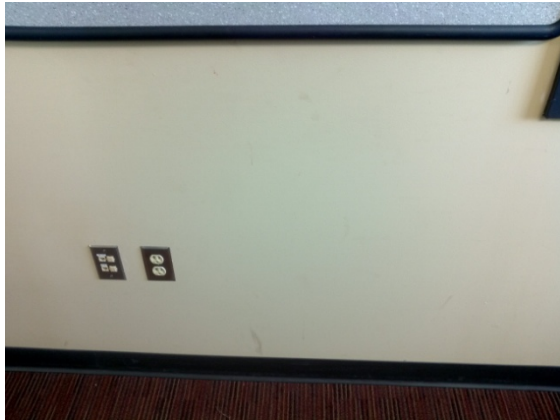
Begrimed wall surface
