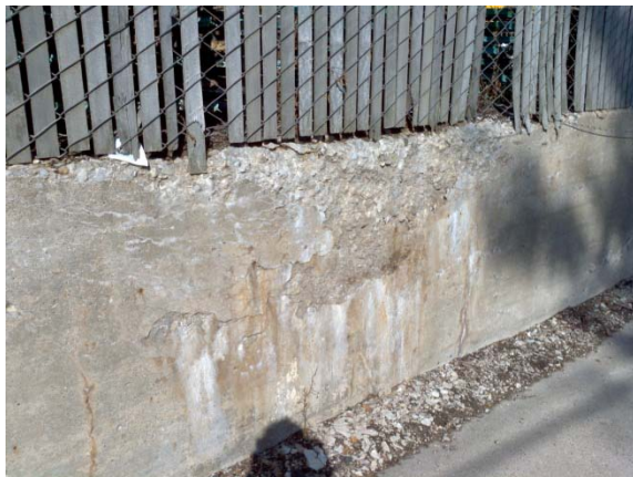
Spalled concrete retaining wall
