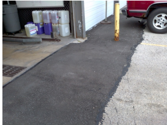
Pavement patch at garage/lot threshold
