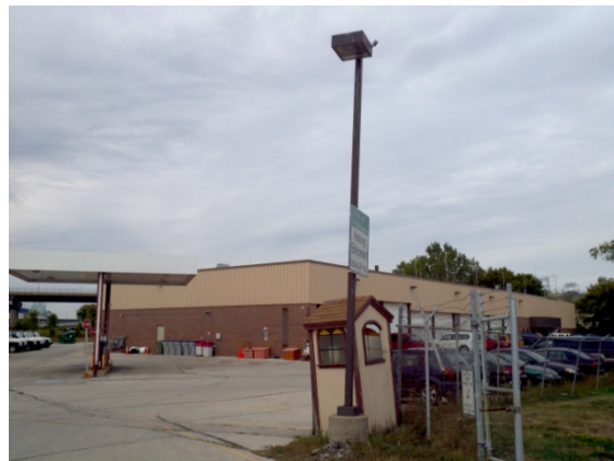
Light pole and fixture at east lot
