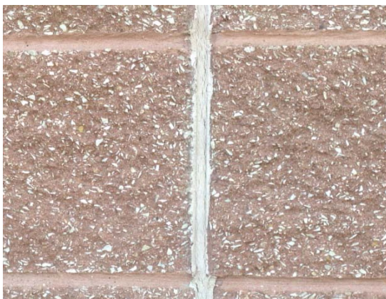
Control joint sealant is cracked/brittle
