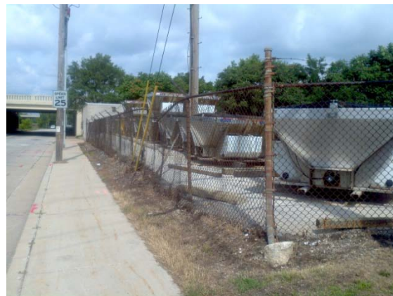
Damaged fence at remote lot
