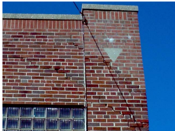
Parallel step cracks east elevation
