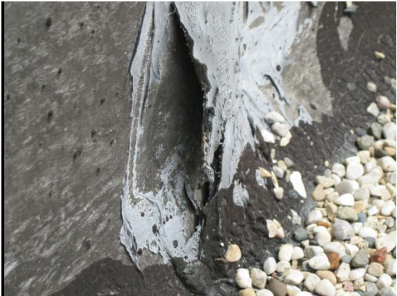
Detached membrane at Roof 2
