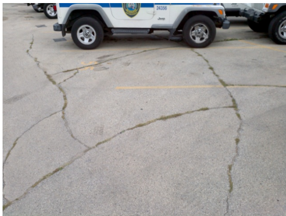
Typical cracked pavement at west lot
