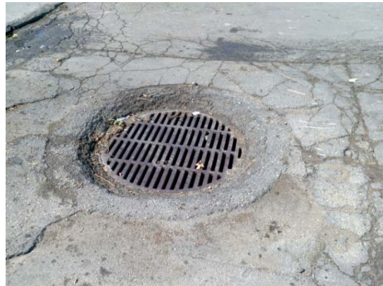
Cracked concrete at entrance drive
