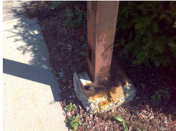
Light pole and base w paint finish deterioration and rust
