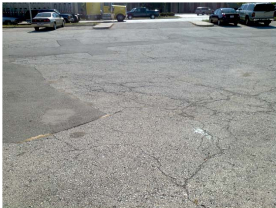
Typical failed pavement
