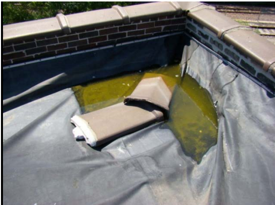
Standing water and detached membrane
