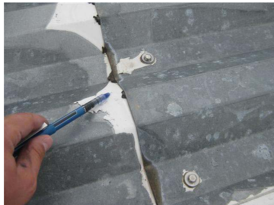
Surface coating missing
