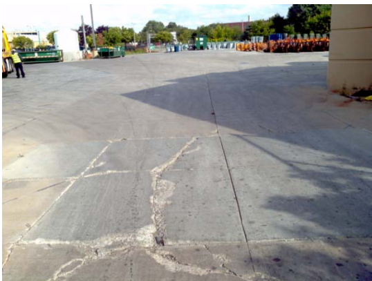
Cracked driveway near salt dome
