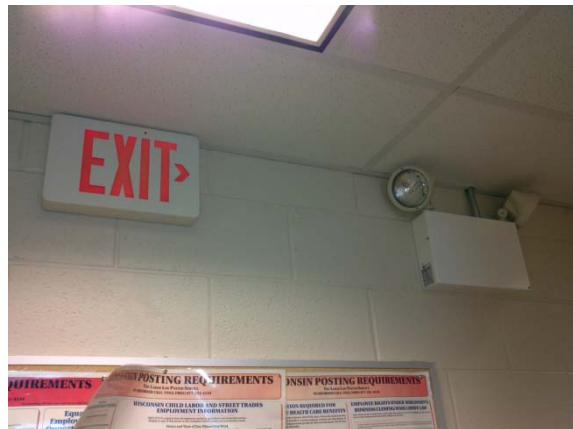
Light fixtures emergency and exit
