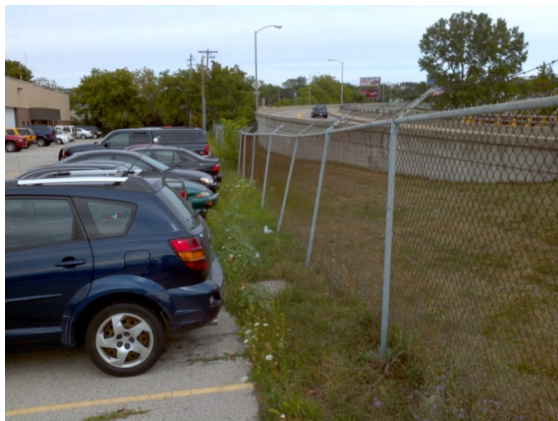
Rusted/Misaligned chain link fence
