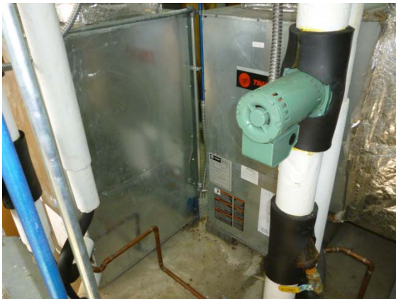
Heat pumps and circulation pump
