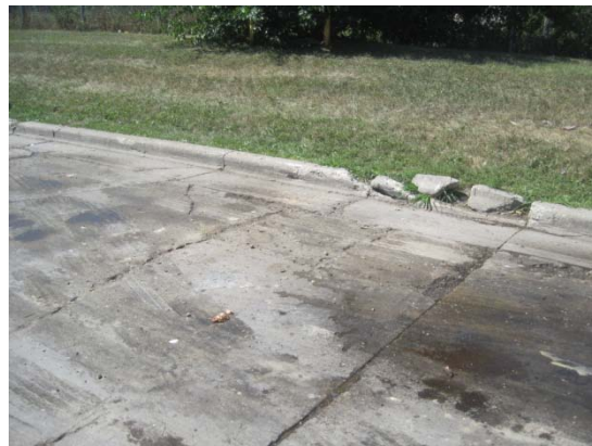
Deteriorated curb near Transfer Station
