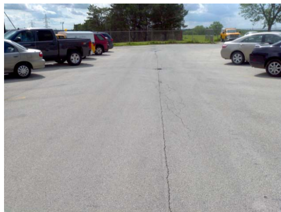
Transverse crack at centerline drainage
