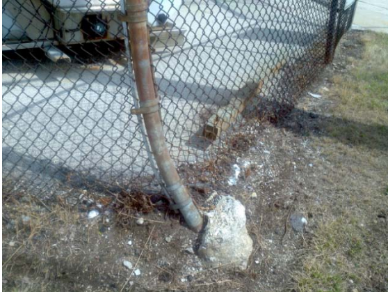
Damaged fence post at remote lot
