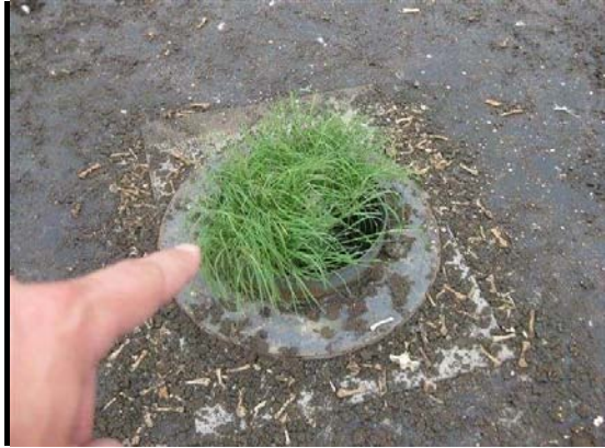
Vegetation growth atop roof near drains
