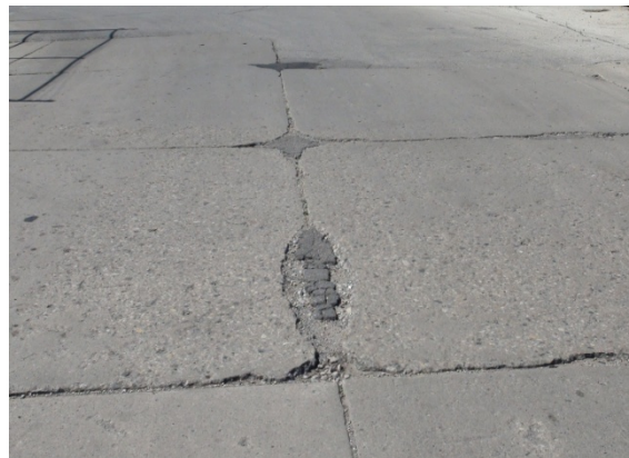
Damaged concrete with asphalt patches
