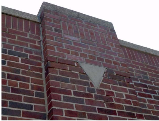
Mortar loss at west elevation
