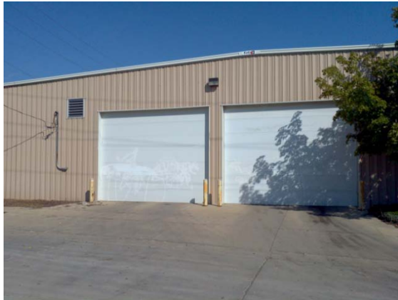
Metal siding at Storage Garage
