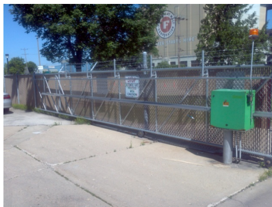
Gate and operator
