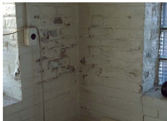
Water infiltration and damaged paint
