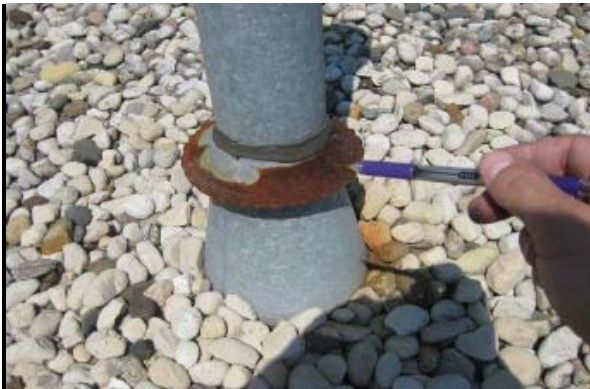
Rusted bonnet at vent
