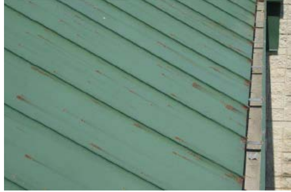
Rusted roof – typical condition
