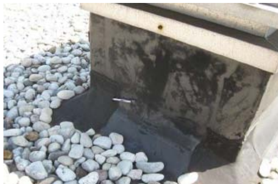
Hole at flashing
