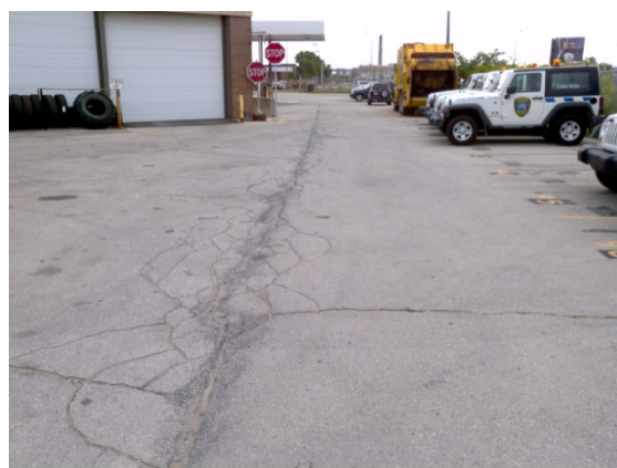
Failed pavement at west lot
