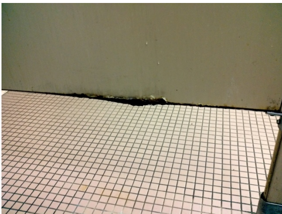
Men's partition w deterioration
