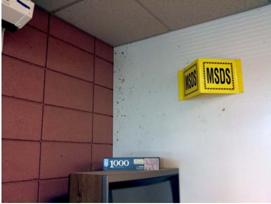
Stained wall in break room
