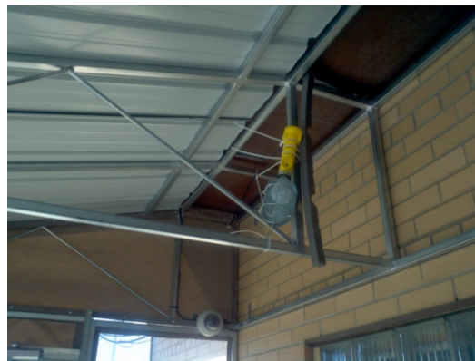
Mechanics lamp used as light fixture
