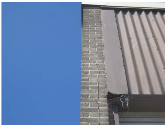
Cracked brick/mortar at Lincoln Garage
