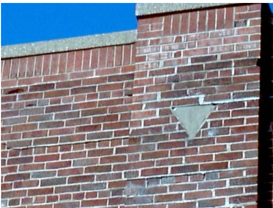
Cracked mortar/spalled brick at east elev.
