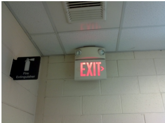
Emergency/Exit light fixture
