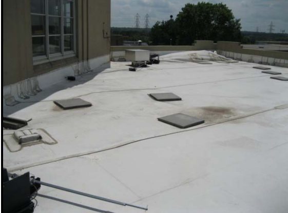
Roof 4 w ponded water
