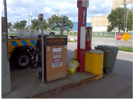
Rusted curb and dispenser
