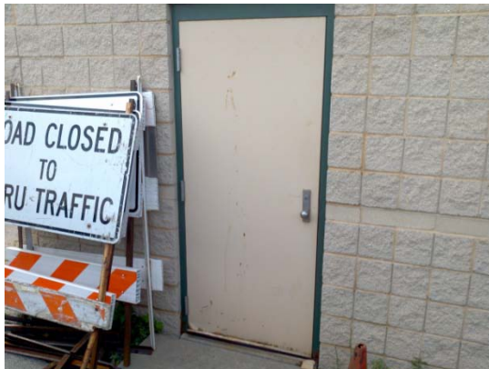
Metal door with rust
