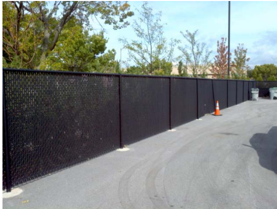
Rusted/Misaligned chain link fence
