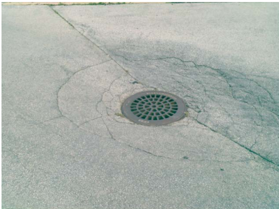
Failed pavement and settled catch basin
