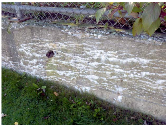
Cracked concrete w efflorescence
