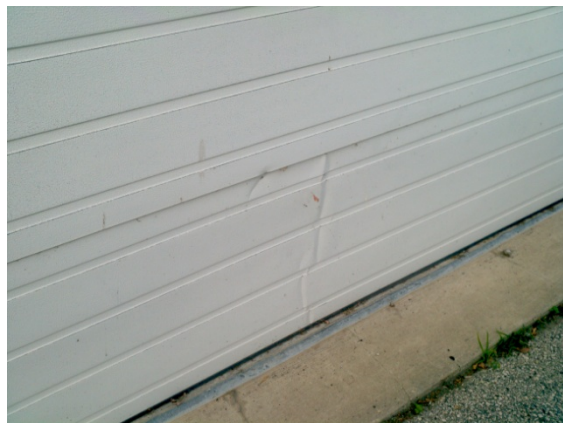
Damaged garage door – fund interim repairs from the operating budget
