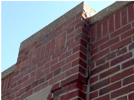
Displaced brick at west elevation
