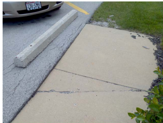
Cracked concrete sidewalk w settlement
