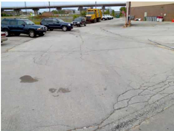
Cracked pavement at entrance
