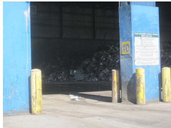
Bollards w surface rust at Transfer Station
