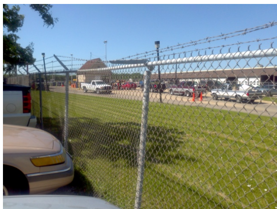
Damaged barbed wire
