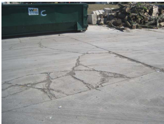
Cracked concrete at Transfer Station
