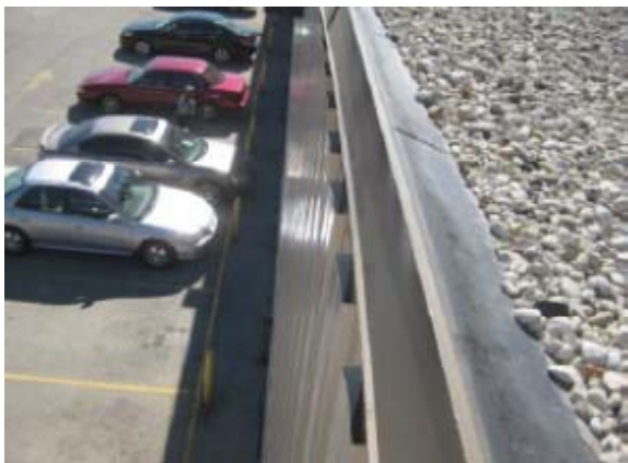
Flashing pulled from siding due to EPDM membrane normalization
