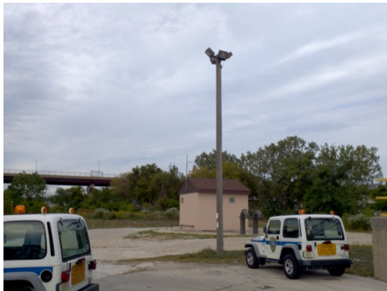
Light pole and fixture at west lot
