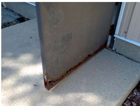
Storage Garage door succumbed to rust
