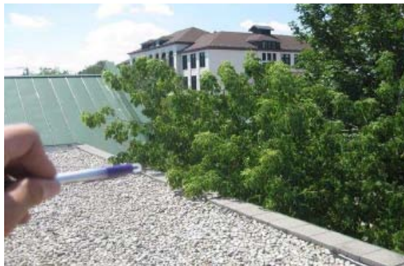
Overgrown tree deposits debris atop roof
