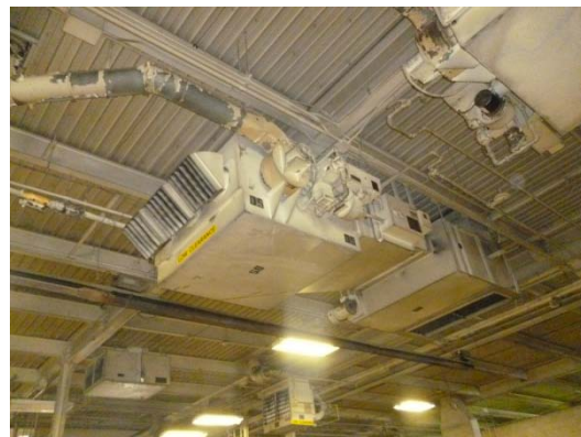
Make-Up air unit
