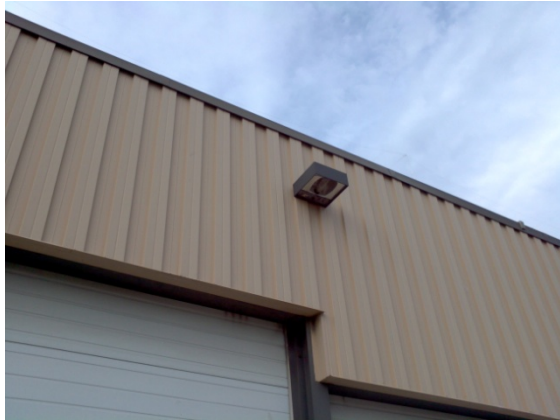
Wall mounted light fixture
