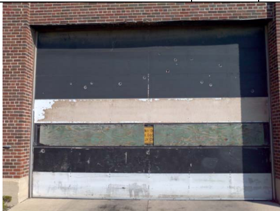
Garage door w repairs at Office Building
