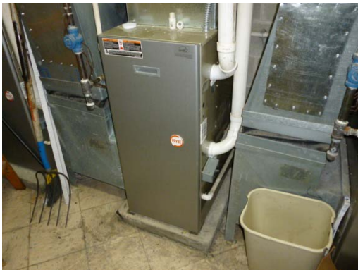
Interior forced air furnace
