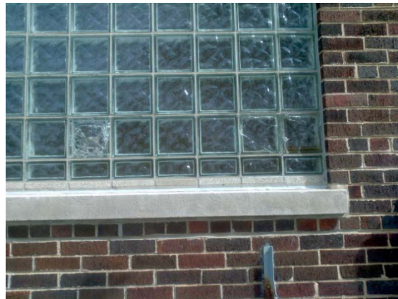
Cracked glass block windows
