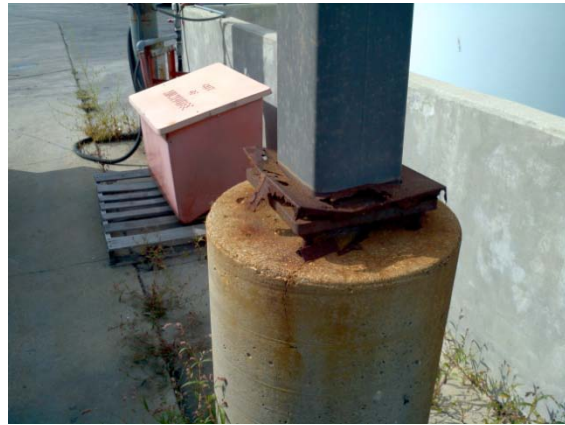
Light pole and fixture w rusted base
