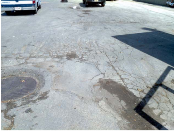
Self Help failed pavement
