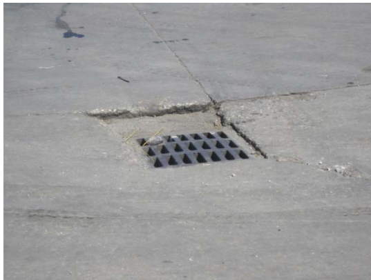
Settled catch basin near Transfer Station
