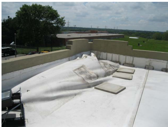
Roof 5 EPDM membrane detached
