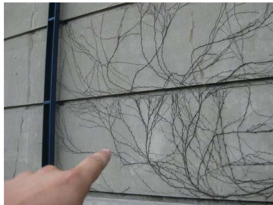
Vines exacerbate deterioration
