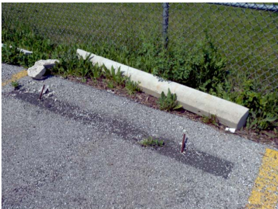
Damaged car stop
