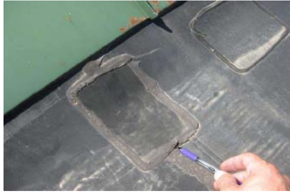
Rubber flashing w hole
