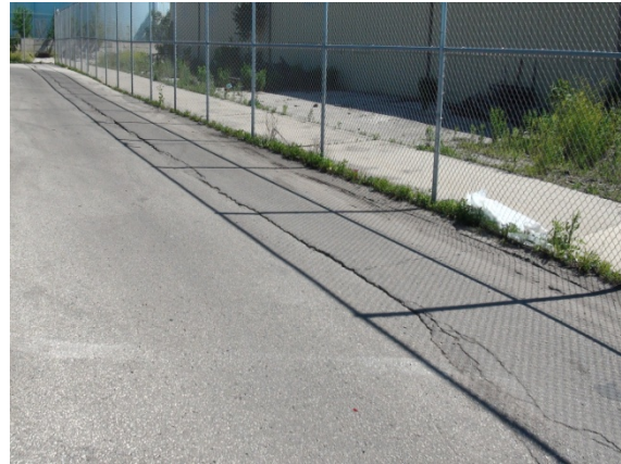
Transverse crack at eastern edge of Tow Lot
