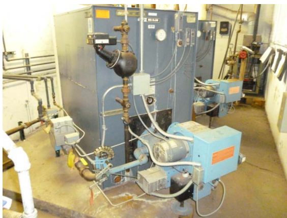
Building heat boilers
