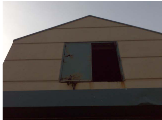
Rusted access door at salt dome
