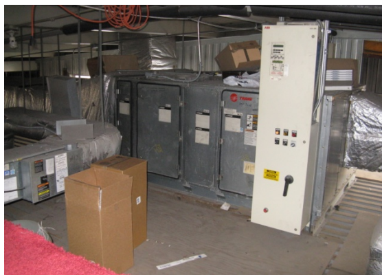
Air handling unit and variable frequency drive at the garage loft
