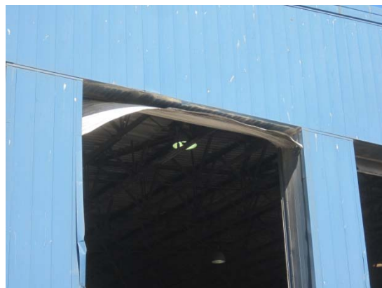
Damaged Transfer Station garage door
