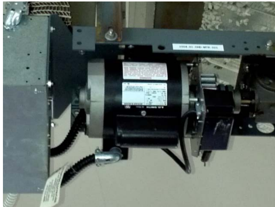
Garage door operator
