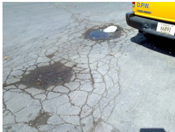
Failed pavement at Self Help
