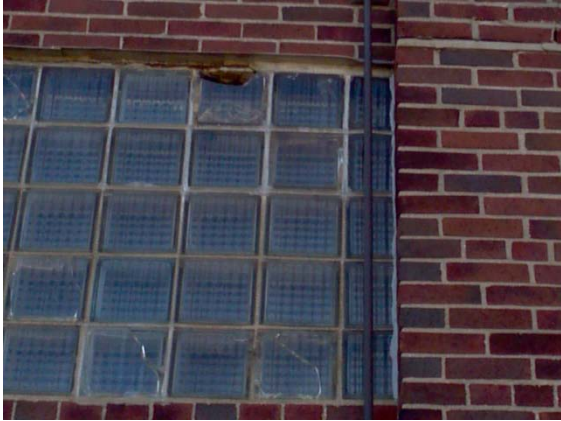
Cracked/damaged glass block
