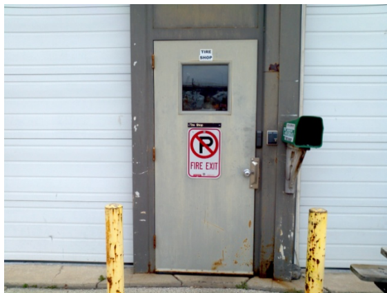
Metal door with rust
