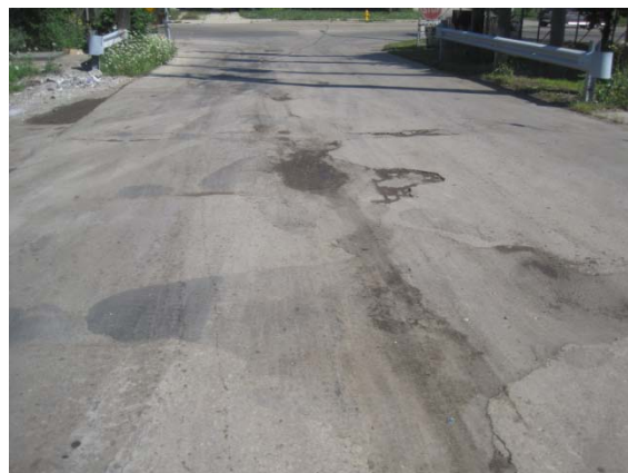
Cracked concrete at Lincoln Garage
