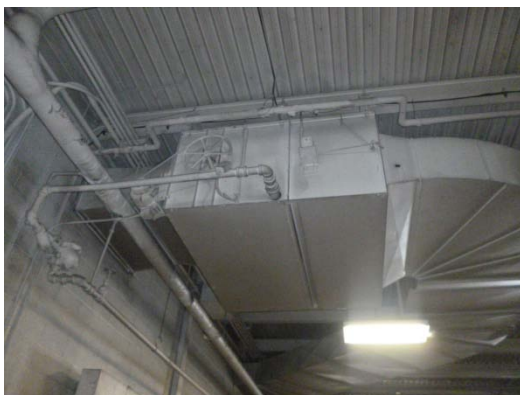
Make-Up air unit
