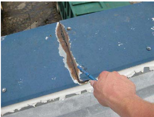
Rusted lap joint
