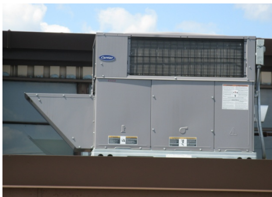
Air handling unit at south offices
