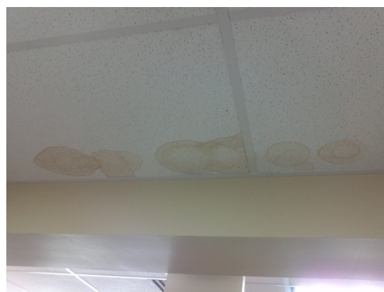
Water stained acoustic tile ceiling
