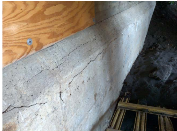
Cracked foundation wall
