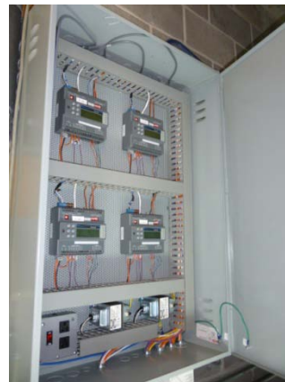
Building automation system monitoring devices
