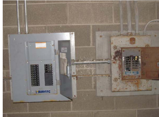
New/old branch circuit
