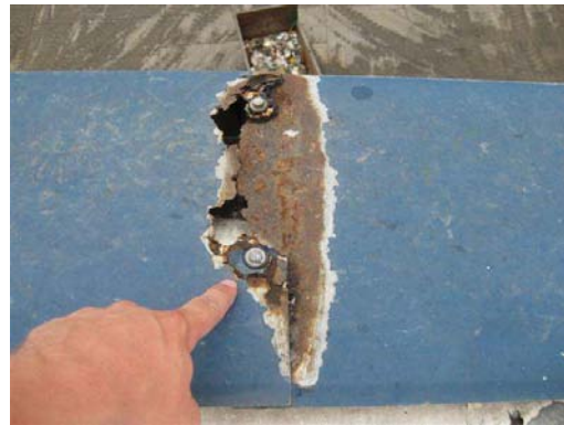
Rusted roof at fasteners every 10 feet
