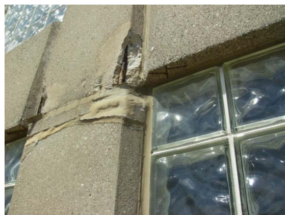
Spalled concrete facade
