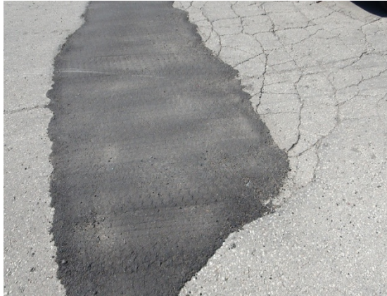
Prior patch w/ adjacent failed pavement
