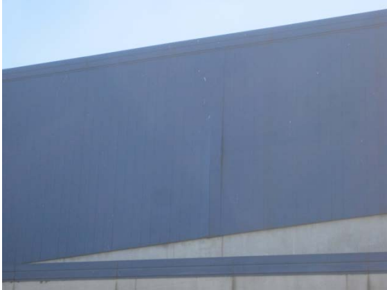
Damaged metal siding
