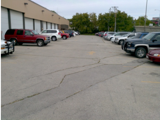
Cracked/Patched pavement at east lot
