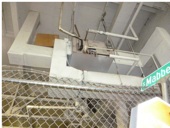
Interior forced air furnace
