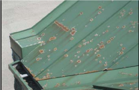
Rusted roof – typical condition
