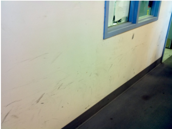
Begrimed wall surface in garage
