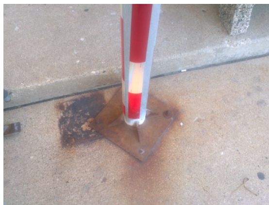
Rusted base plate with missing fasteners
