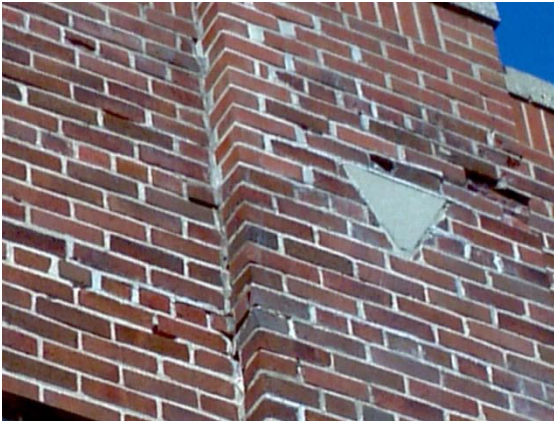
Spalled brick/mortar east elevation
