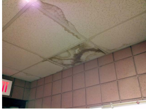
Stained acoustic tile ceiling in break room
