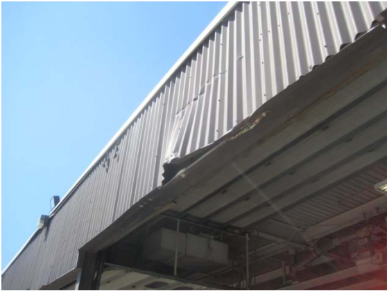
Damaged siding at Lincoln Garage
