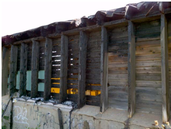
Damaged structural components
