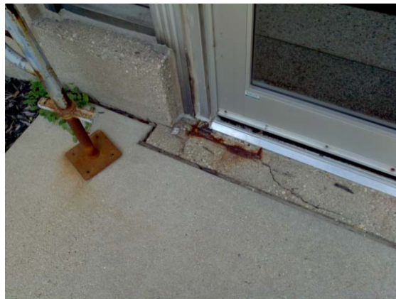
Cracked threshold at door
