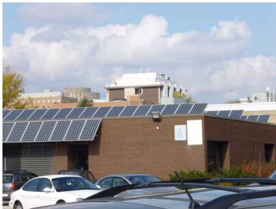
Roof mounted solar panels
