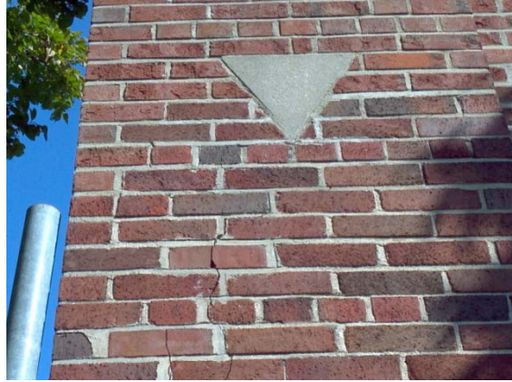
Cracked brick/mortar at south elevation
