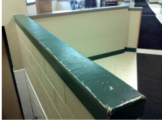
Worn paint at wall ledge
