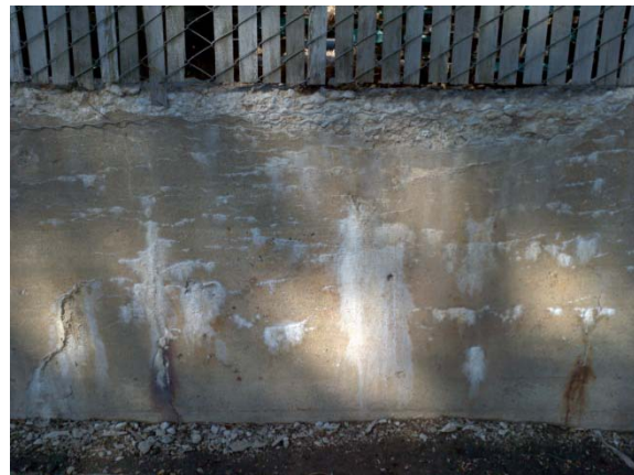
Cracked wall w efflorescence
