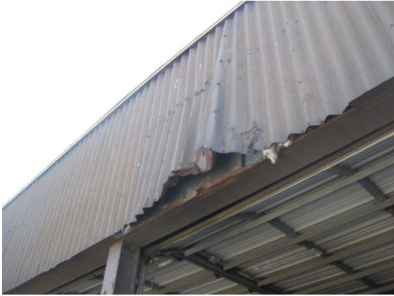
Damaged siding at Lincoln Garage
