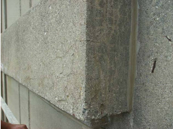
Cracked concrete eyebrow
