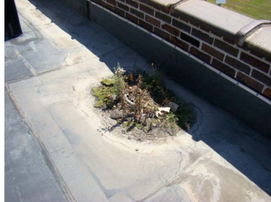
Plant growth at drain
