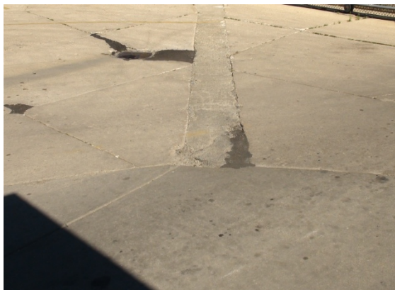
Damaged concrete with asphalt patches
