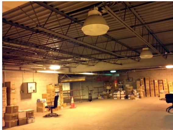
Storage room light fixtures
