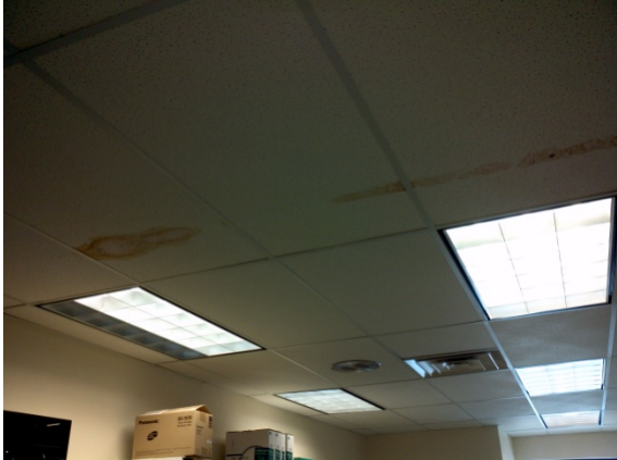
Stained acoustic tile ceiling panels
