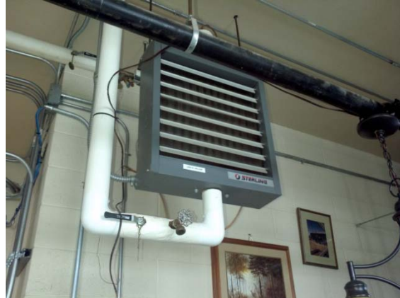
Typical unit heater
