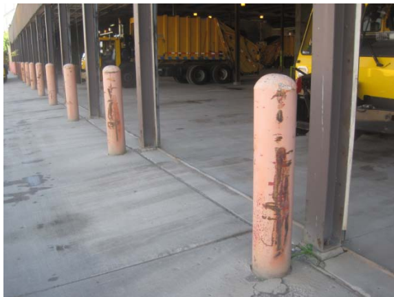
Bollards w surface rust at Lincoln Garage
