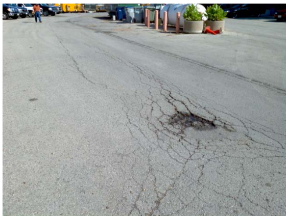
Pothole and failed pavement
