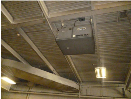
Air filter unit
