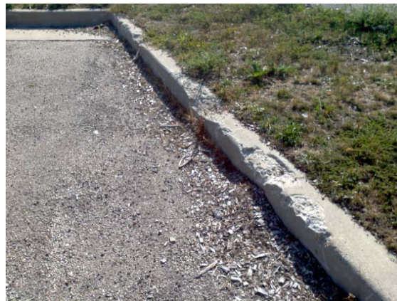
Deteriorated concrete curb
