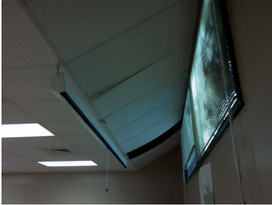
Acoustic ceiling tile missing
