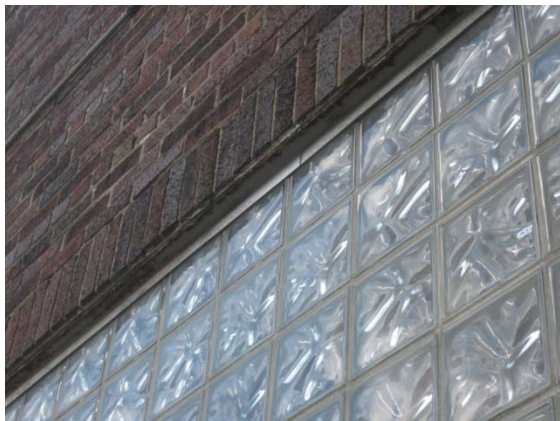
Typical rusted lintel
