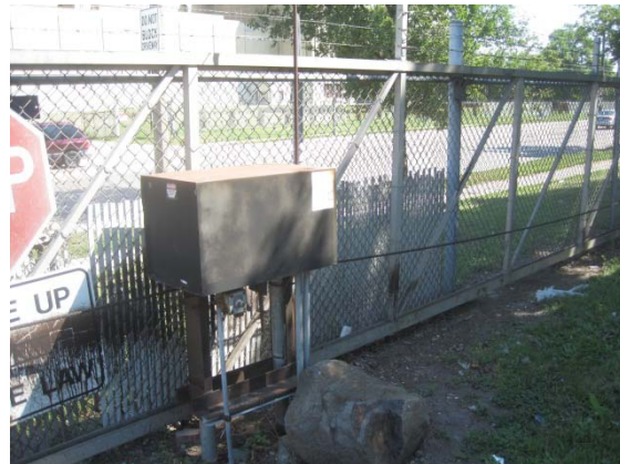
Gate and operator
