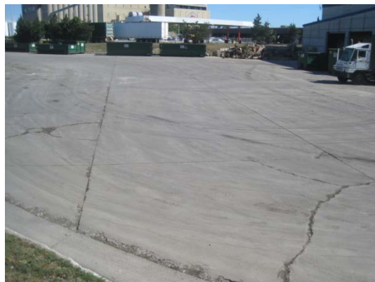
Cracked concrete at Transfer Station
