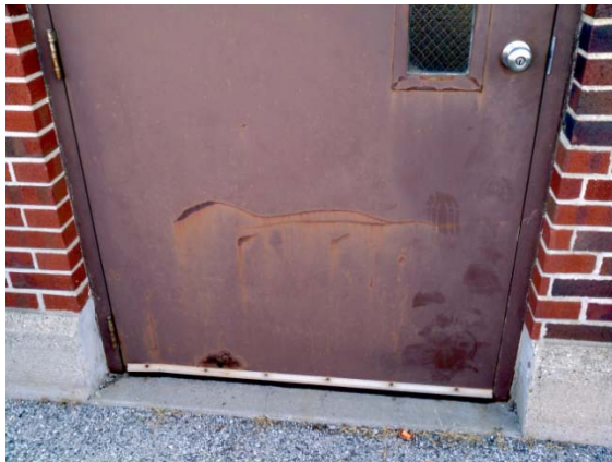
Office Building door with rust
