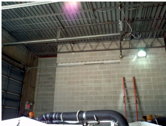
Garage light fixtures
