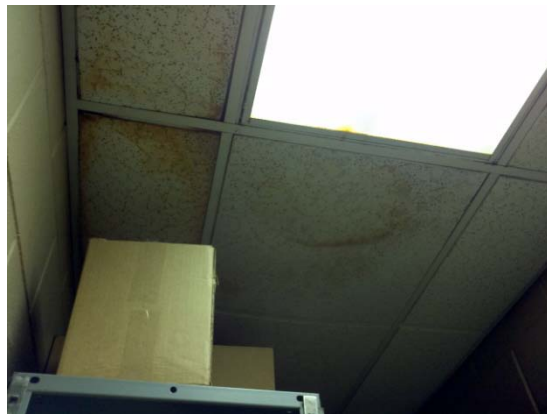
Storage room light fixture – replace damaged tile from O + M funds
