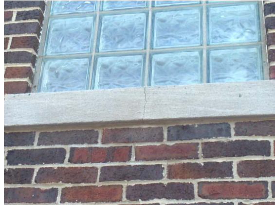
Cracked concrete sill
