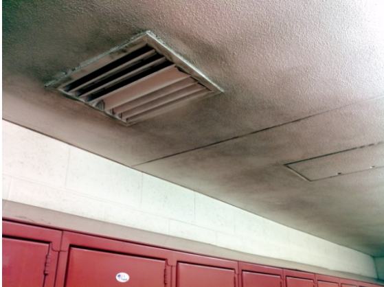
Men's rest room ceiling damage
