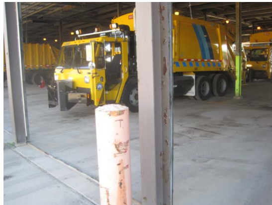
Rusted steel components
