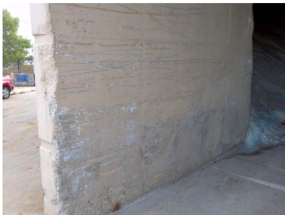
Damaged salt dome
