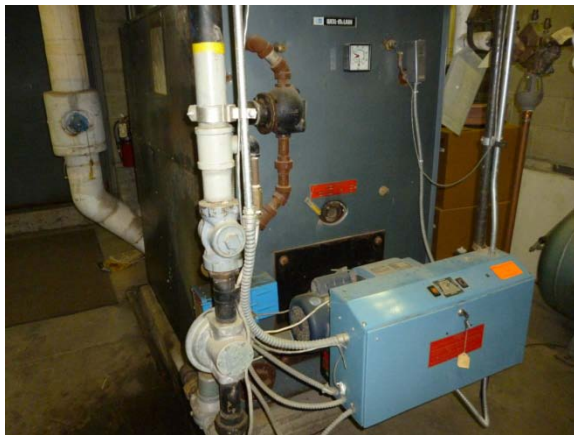
Building heat boiler
