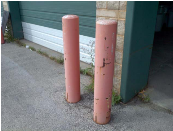
Bollard with surface rust
