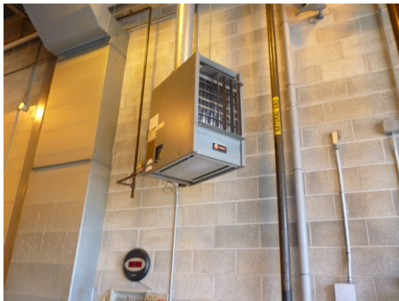
Garage unit heater
