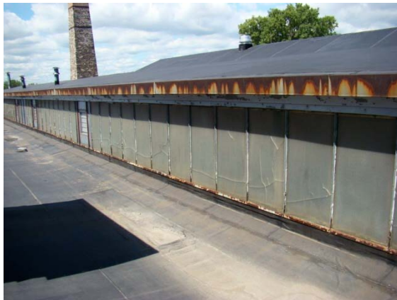
Cracked clerestory windows
