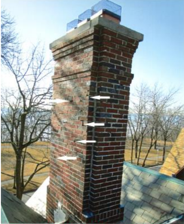
Chimney on the front of the home has large gaps in the mortar. In need of tuck pointing
