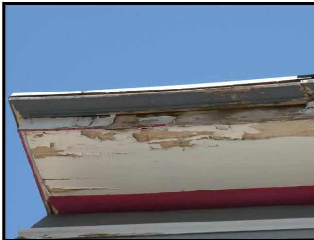
Figure 4.12. Fascia and soffit with failing paint due to moisture absorption.
