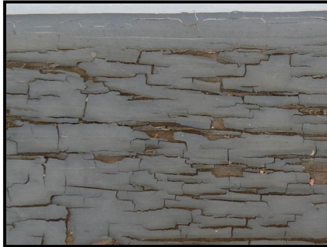
Figure 4.15. Cracking and cross-grain cracking (alligatoring) of the paint.
