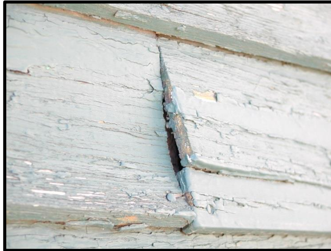
Figure 5.3. Cupping and splitting of boards on a historic theater building.
