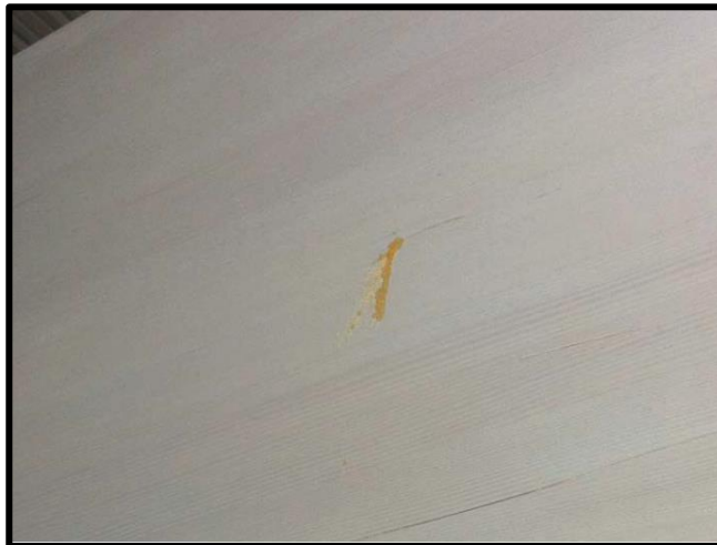
Figure 2.7. Although there is no visible evidence of a pitch pocket on the surface of the wood, the sap indicates the presence of one beneath the surface.
