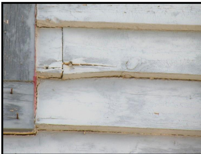
Figure 4.16. Wood siding and trim with areas of chalking. The splits in the wood are due to overdriven fasteners, not the performance of the coating.
