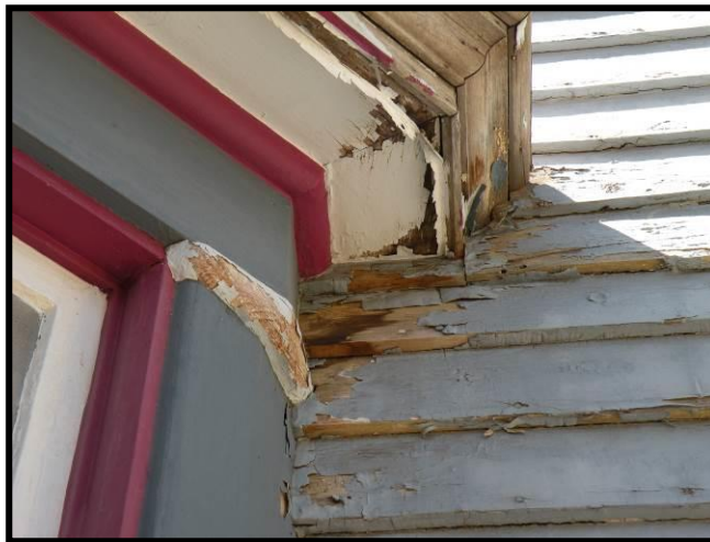
Figure 4.11. Coating failure near the end grain in an area where water flowed down the face of the exterior cladding, as evidenced by the moisture stains on the exposed wood.
