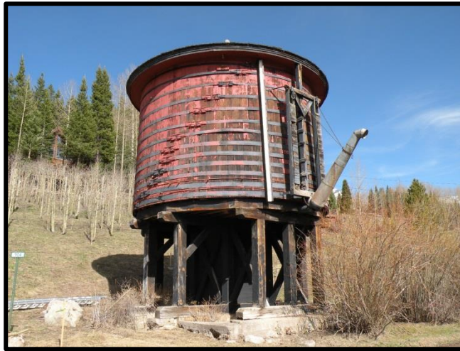
Figure 5.2. Deterioration of the staves of this water tank has resulted in friable wood surfaces that are delaminating. Given the fragile surface condition of many of the staves, repainting is not advised due to the potential damage that could result from removing the existing paint and properly preparing the surface for repainting; instead, replacement material can be painted to match the existing color, and the existing paint allowed to continue weathering.
