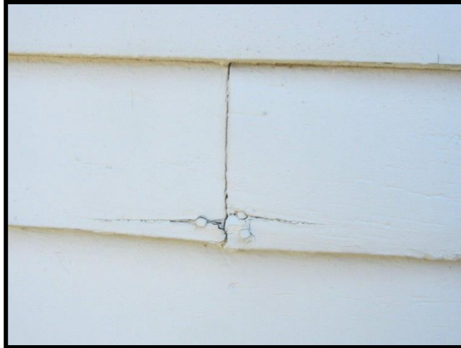
Figure 5.4. Horizontal siding with a butt joint. Note the siding has also been face-nailed in an attempt to prevent or minimize cupping. Face nailing tends to lead to board failure, as the wood is forced to move differentially, leading to splits, as shown here.
