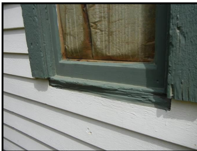
Figure 4.17. Missing window sill.
