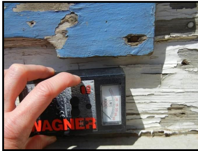
Figure 4.19. Use of a pinless (capacitance) moisture meter to determine the moisture content of siding.
