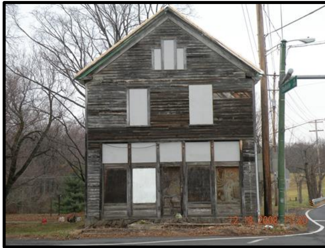
Figure 5.1 Weathered cladding from a naturally durable wood species that results in an appearance quite different than if it was painted.
