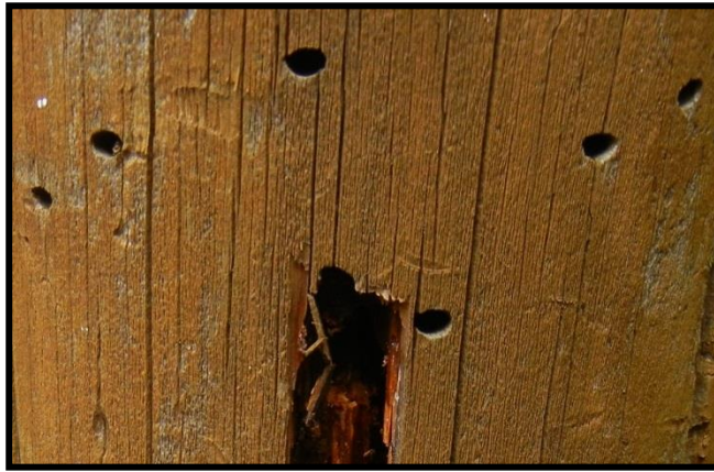
Figure 4.10. Bore holes in a stained column (also with deterioration by wood-decay fungi).
