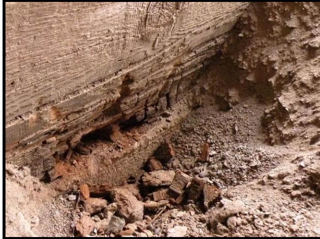
Figure 4.8. Deterioration of wood caused by wood-decay fungi.
