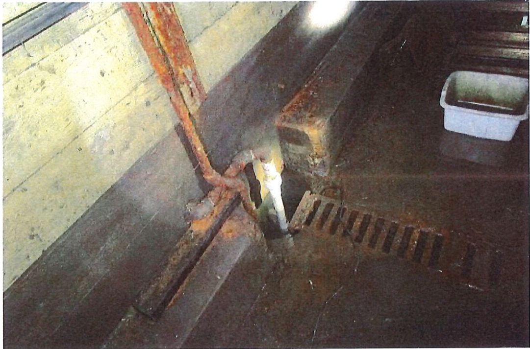
Trench drain and sump
