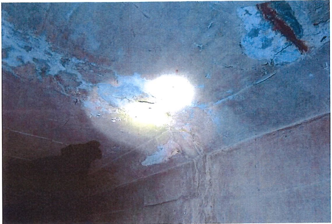
Spalled concrete and exposed rebar
