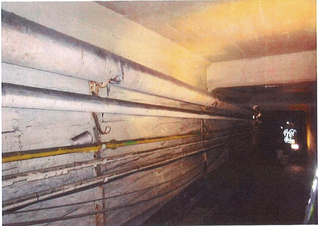
Pipes along south wall
