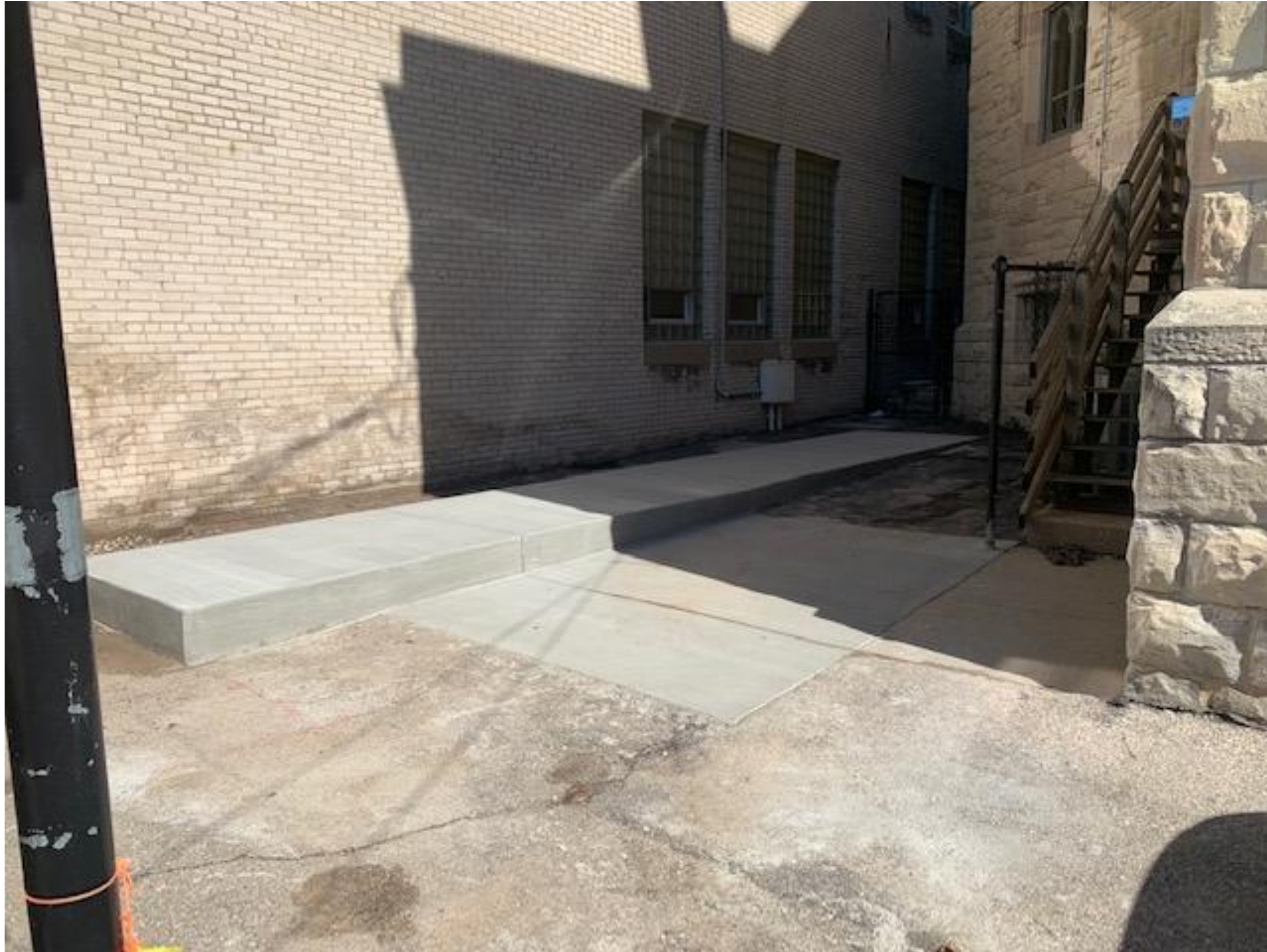
Additional image of the site and concrete platform that will house the three outdoor condenser units
