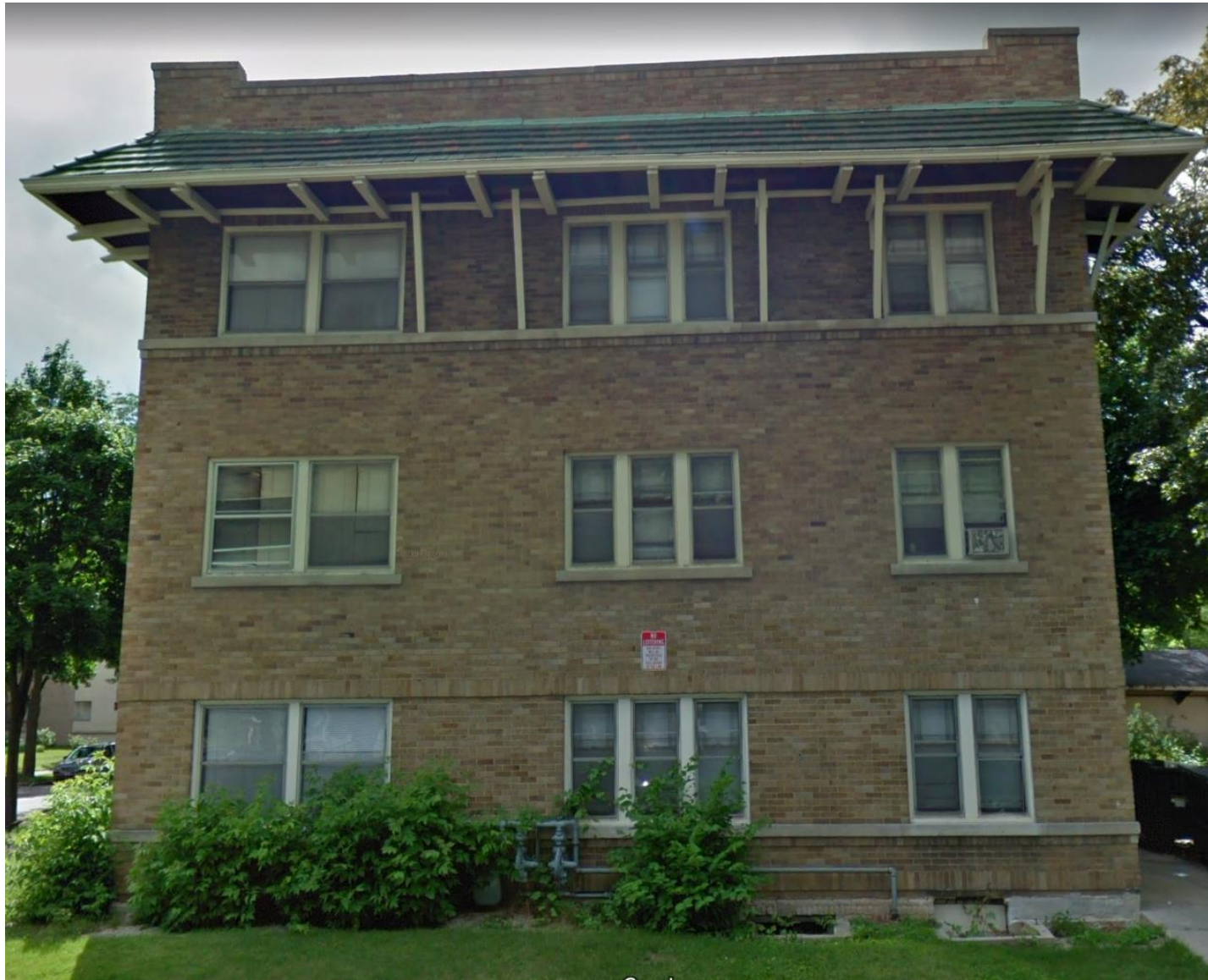
28 th Street elevation in 2011. Leftmost 8 windows are to be restored as paired 15-pane casements as in photo on page 3. West elevation shall follow these same requirements. See elevation plans on next page.
