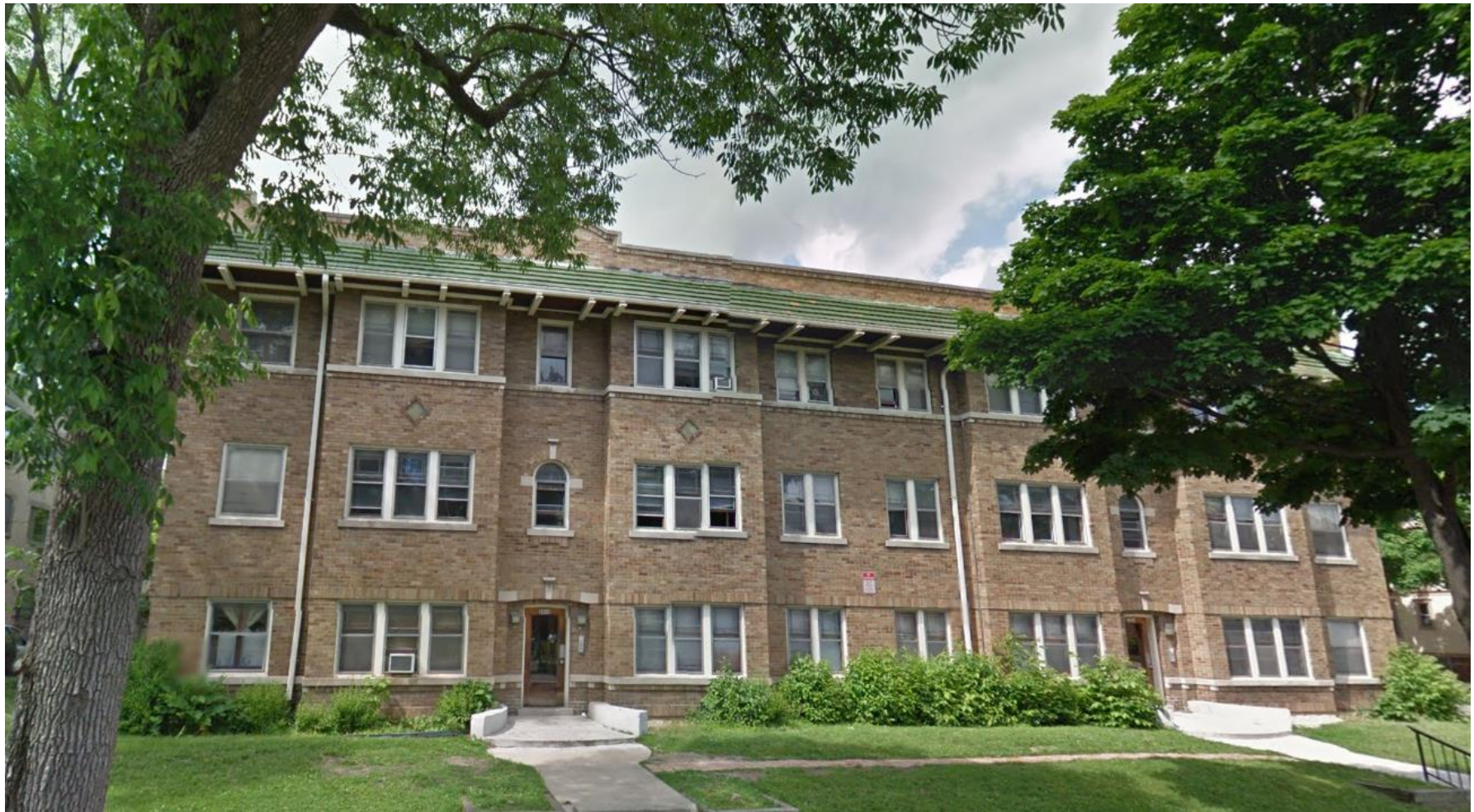
2011 photo showing location of all stained glass windows on front. All must be restored. Outside corner windows were leaded casement with no stained glass. See plans on later pages.
