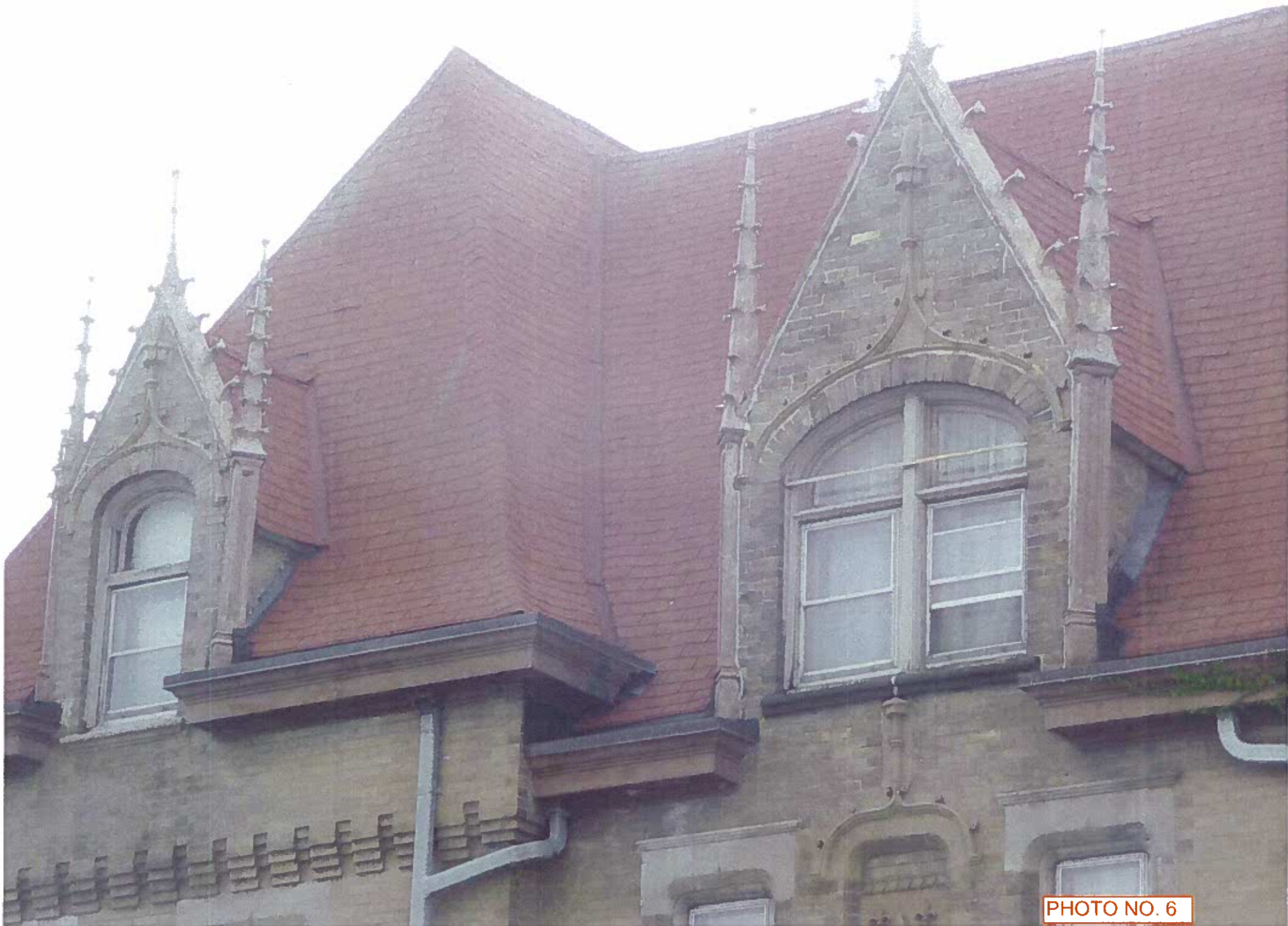
BLOODGOOD RESIDENCE - North elevation Typical condition of dormer windows and decorative elements
