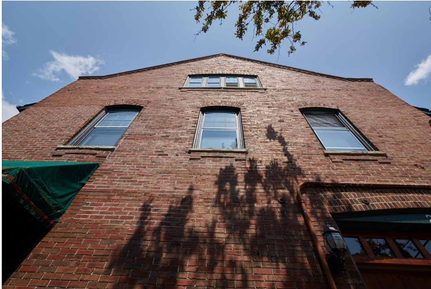
Primary wall with issues.
