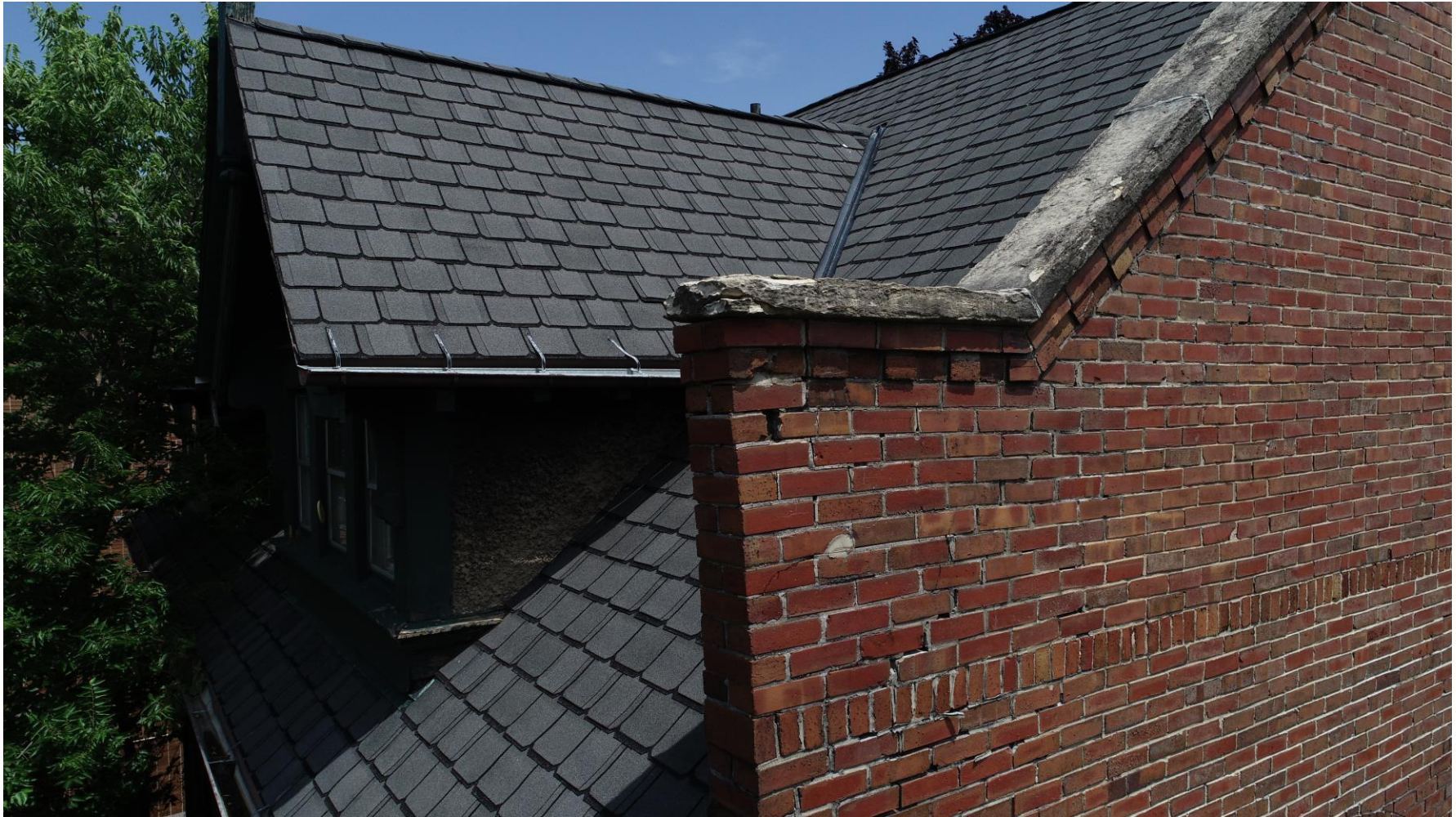
Typical damage and detail of parapet.
