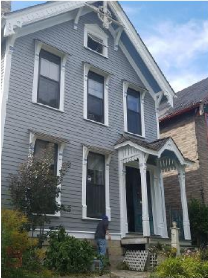
front of house with existing porch which will be repaired (note: at the time of this photo, railings were removed to complete painting of trim and columns)
