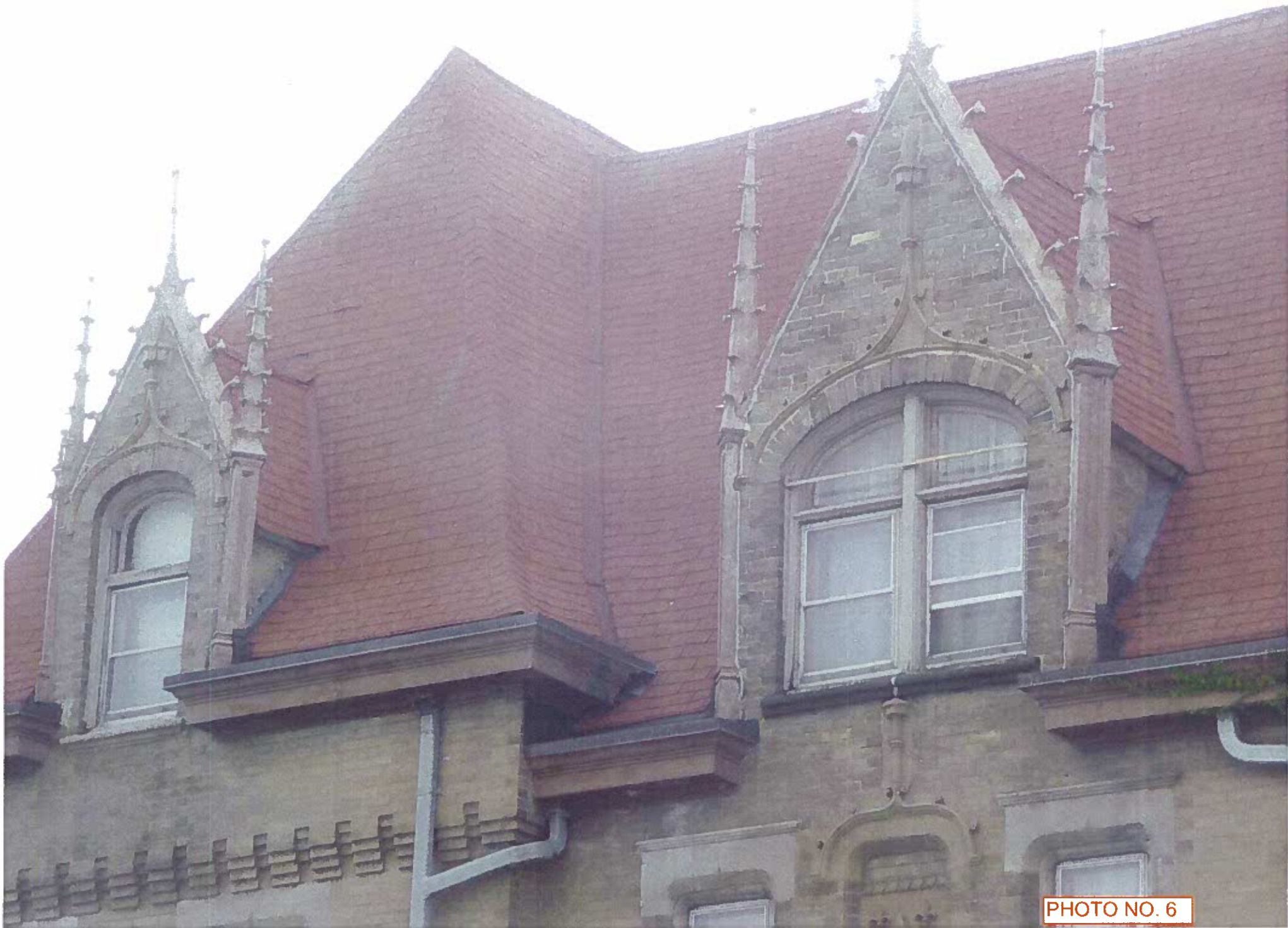
BLOODGOOD RESIDENCE - North elevation Typical condition of dormer windows and decorative elements
