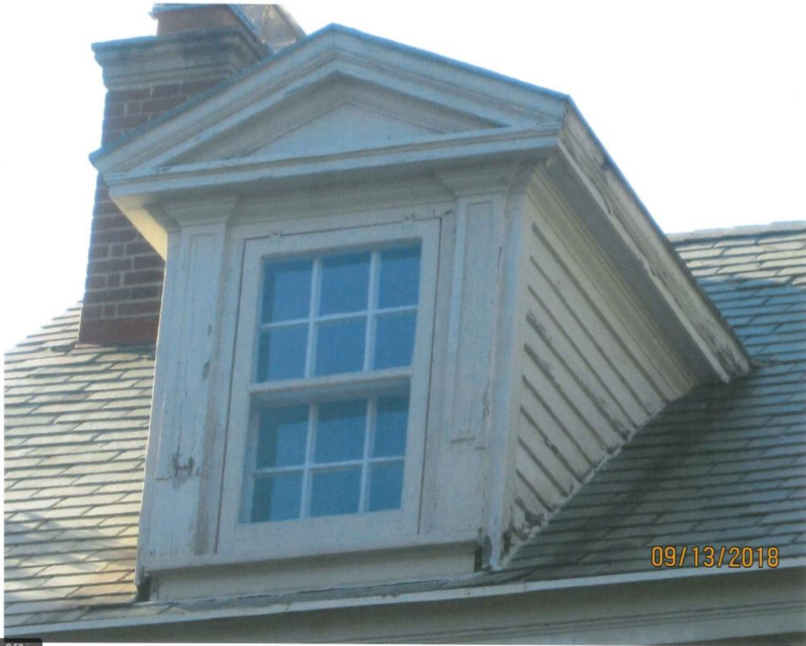
11:00 AM 2:50 PM Typical dormer window conditions. Repairs and replacement to replicate existing details exactly will be completed.
