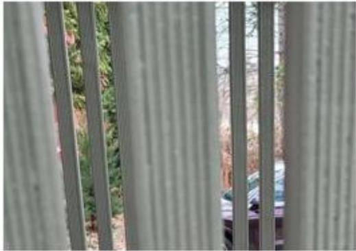
Existing Spindles (Front Porch)
