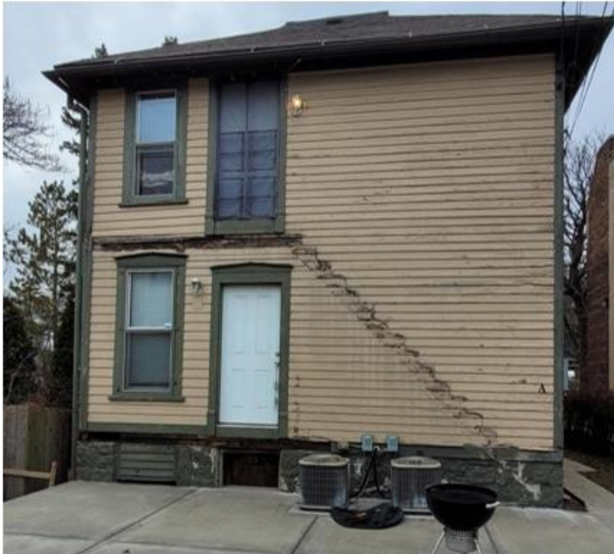
Existing Rear Elevation (After demo) Note existing non-compliant stair rise and run (slope) on paint.
