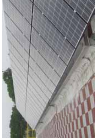
Photovoltaic Panels Cooper School - Milwaukee, Wisconsin
