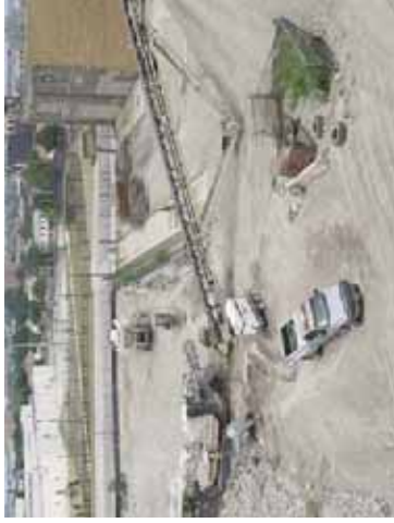
The Brewery Project will be able to save many of the existing buildings for adaptive re-use: but as for the buildings that were razed, 80% to 85% of the materials are being recycled. One third of the demolition costs are being off-set by the salvage value.
