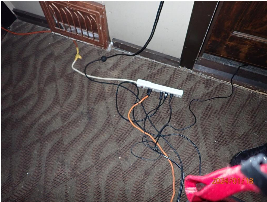
Above – Spliced Electric Cord (yellow tape) and cord leading out of door. Below, additional hazard.
