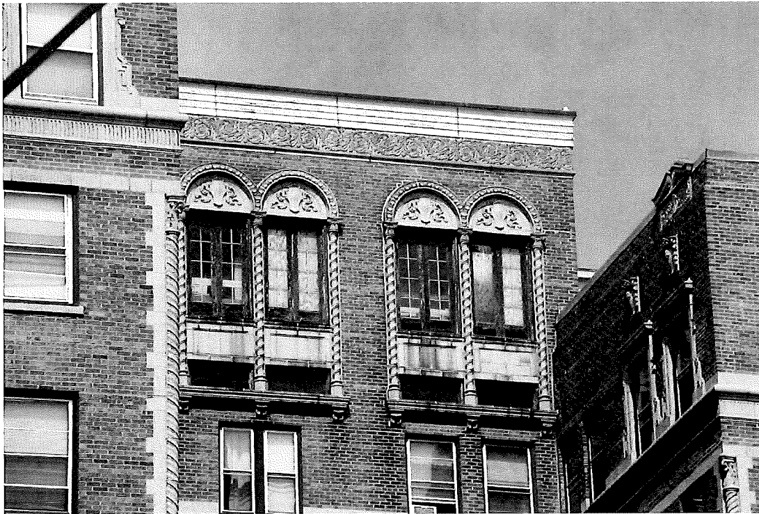
Figure 9. Wisconsin Architecture and History Inventory, Record #113449. Photo taken 2015. Detail of windows on the front elevation, view facing west
