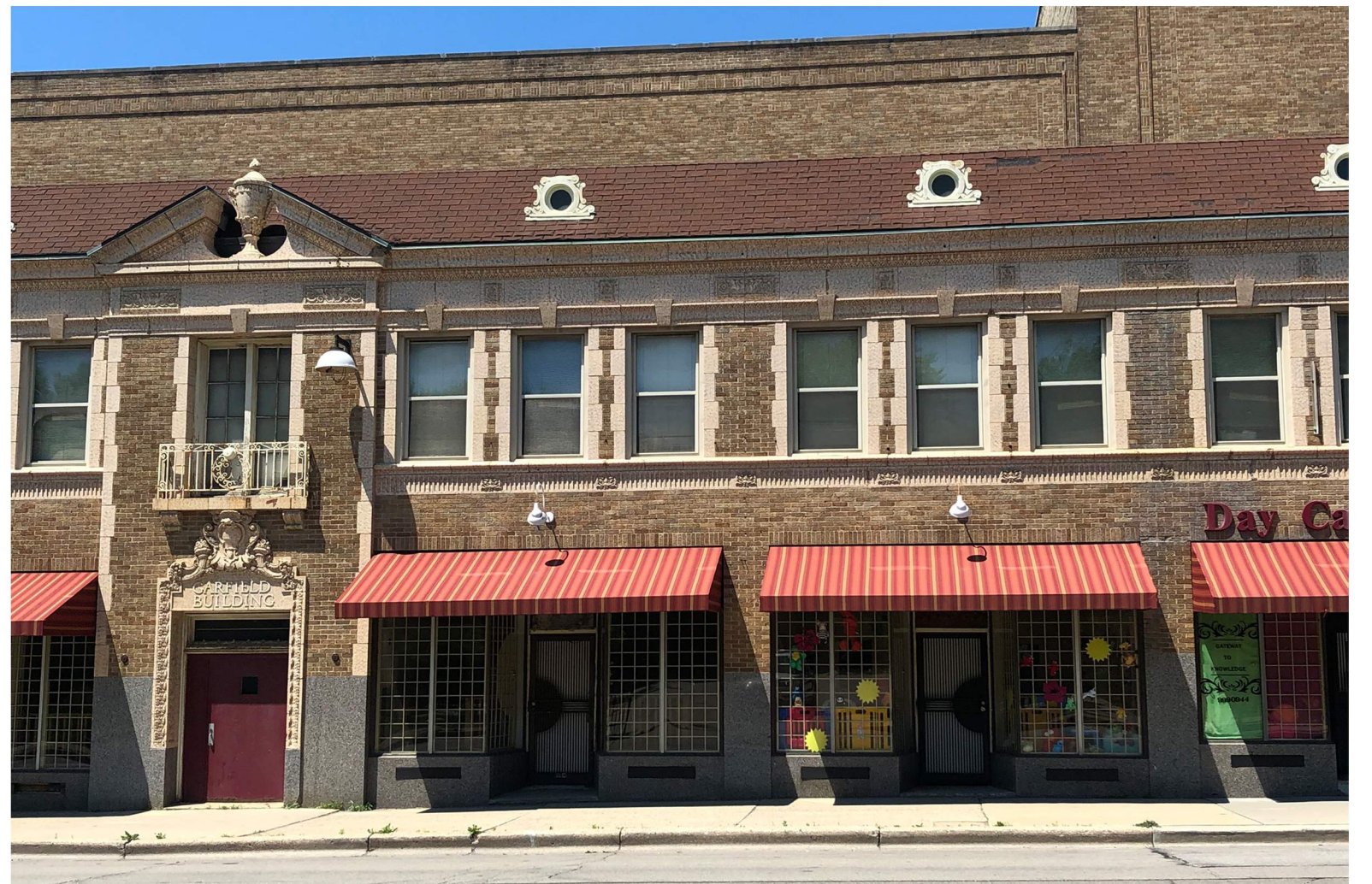
Existing detailed brick, terra cotta, and tile to be preserved, new exterior walls coordinated to match
