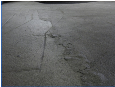
Loose membrane at 3rd floor
