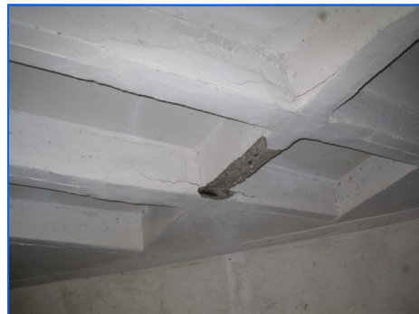
Paint finish with rust
