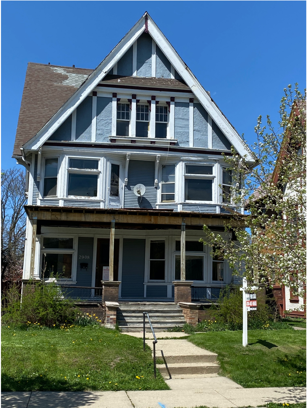
Front of House Note the Missing Shingles on the Roof
