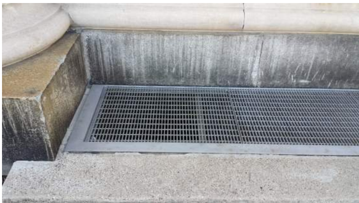
Photo 36 – WINDOW AREA WELL GRATE. O247. West elevation, grate no. 8, typical. Installation of new stainless steel grates, frames, fasteners. Annual maintenance required for “tea stains” resulting from oxidation (superficial only) caused by seasonal use of chemical deicers.
