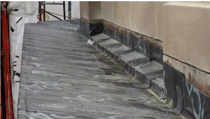
Photo 12 – West elevation. Installed dutchman, waterproofing membrane over treated plywood substrate on structurally sloped cornice gutter stone. Existing stone reglet, at back wall, cleaned and re-used at installation of the new metal counter-flashing.
