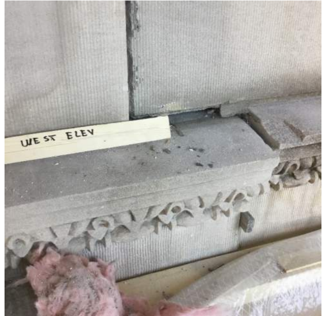
Photo 32 – Northwest cartouche. Found condition of lower edge of stone displacement.
