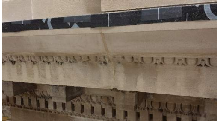
Photo 8 - West elevation. Installed, mortar-joint, cornice edge Dutchman. Waterproofing membrane laps over substrate of treated plywood with stainless steel end channels at border for continuous rigidity between plywood panels. Pending gutter flashing.
