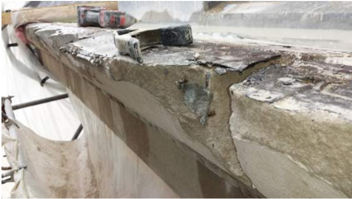
Photo 1 – O118 CORNICE GUTTER EDGE Southeast elevation. Existing condition with flashing removed. Nails shown held “filler” in-place. Damage done by power-fastening gutter flashing.
