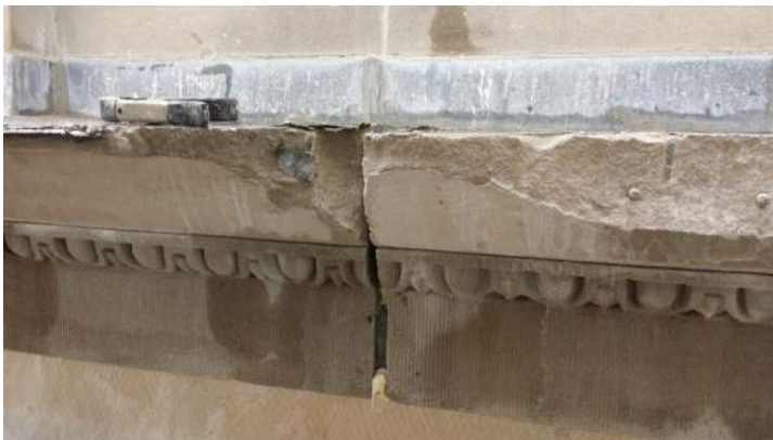
Photo 3 – East elevation. The horizontal cut is the first cut just above the carved egg and dart. Carefully made as this will seat the new Dutchman when damaged area is removed.
