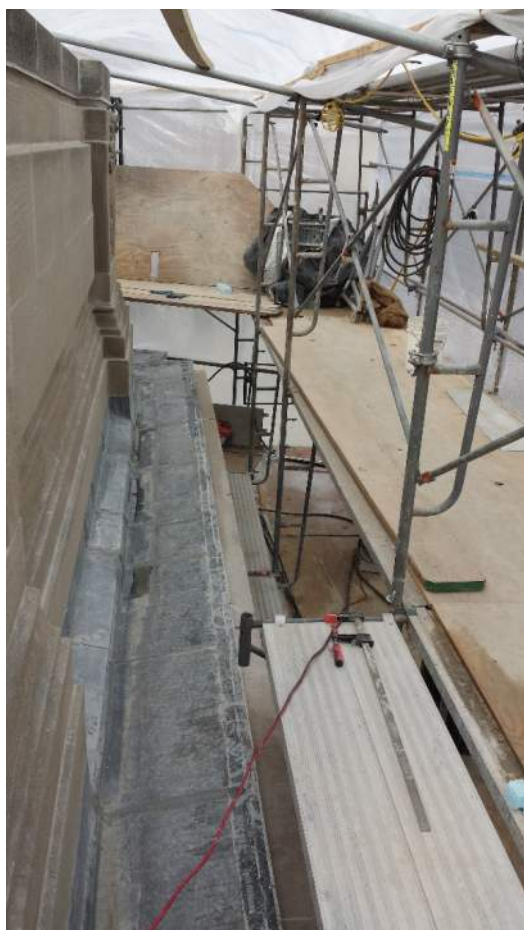
Photo 20 – West elevation, view from southern end. Parapet railing capstones reset. Cornice gutter edge removed by saw-cutting. Removal of existing flashing, in progress.
