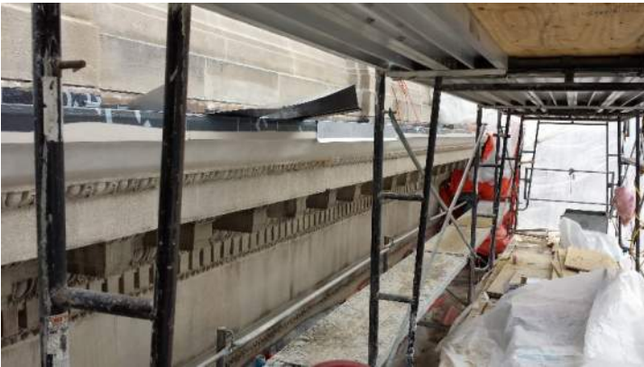
Photo 9 – West elevation. CORNICE GUTTER FLASHING. Lead-coated copper with expansion joints mock-up, in progress.
