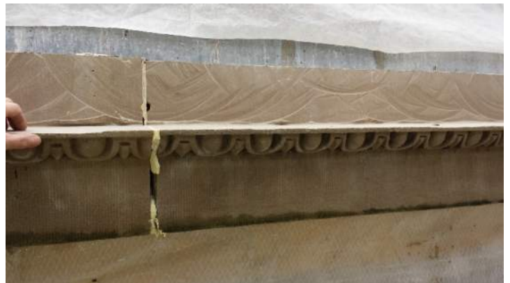
Photo 4 – East elevation. Removed the damaged stone. Note the successive lowering of the hand-held saw to the horizontal cut made, in the vertical cut.
