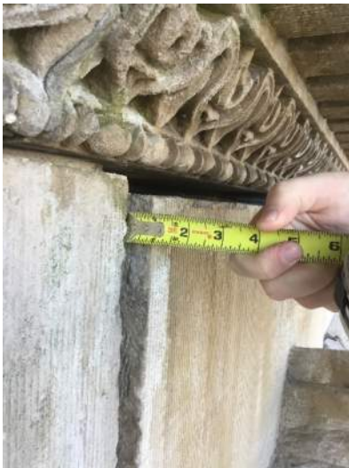
Photos 23 – North cartouche. Found condition of upper edge showing displacement.
