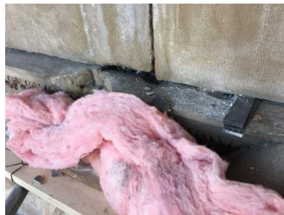
Photo 25 – North cartouche. Found condition of lower edge of displacement. Note insertion of dowels in the outer decorative stone band made in a past intervention.
