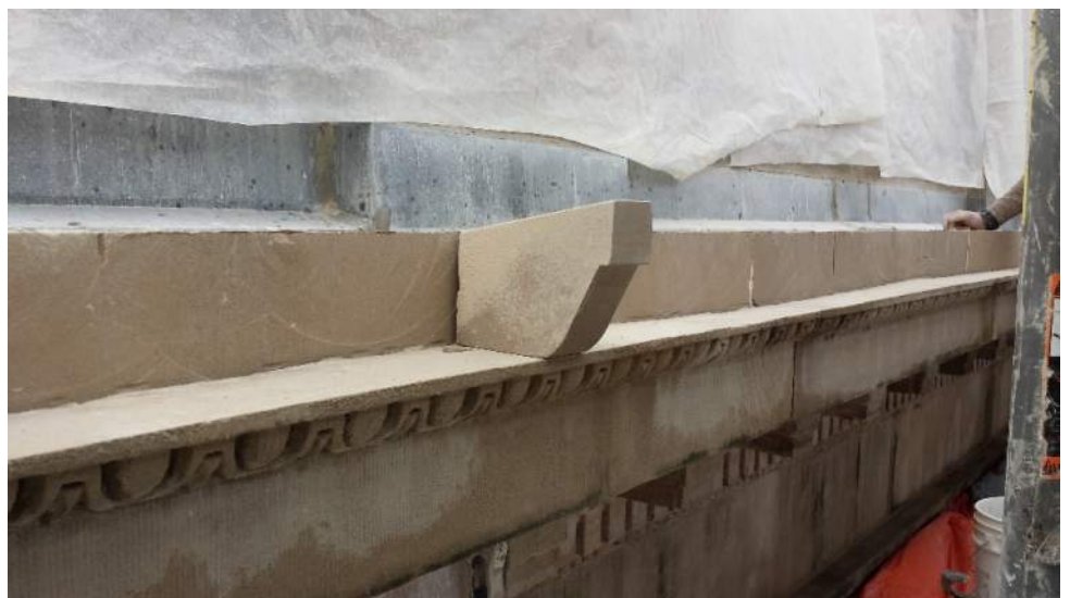
Photo 6 – East elevation. Preparatory work, sample Dutchman element, verifying drainage allotment and horizontal setting-bed.
