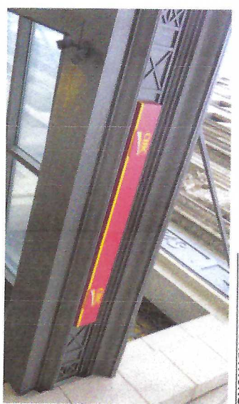
Existing 8" x 6'-0" sign to be removed & replaced. Wall patched and painted as required.
