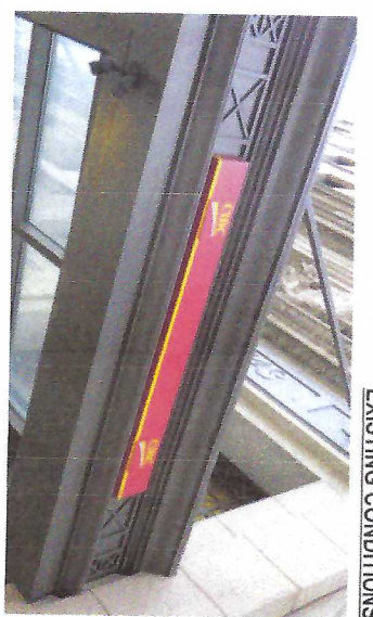
Existing 8" h x 6'-0" w sign to be removed & replaced. Wall patched and painted as required.
