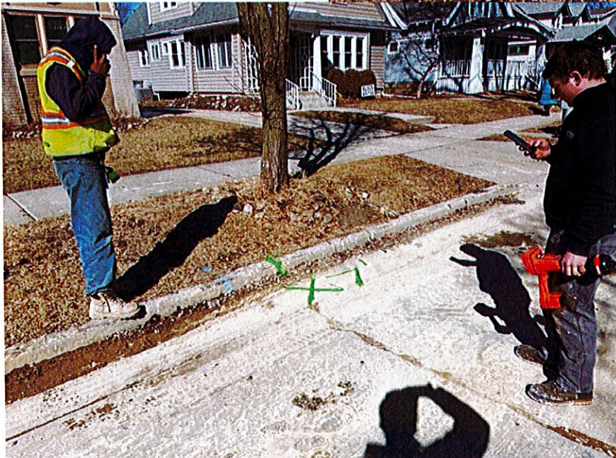
Photo #24: Heiden Plumbing marking and recording the location of city's broken lateral sewer drain pipe on March 11, 2022.
