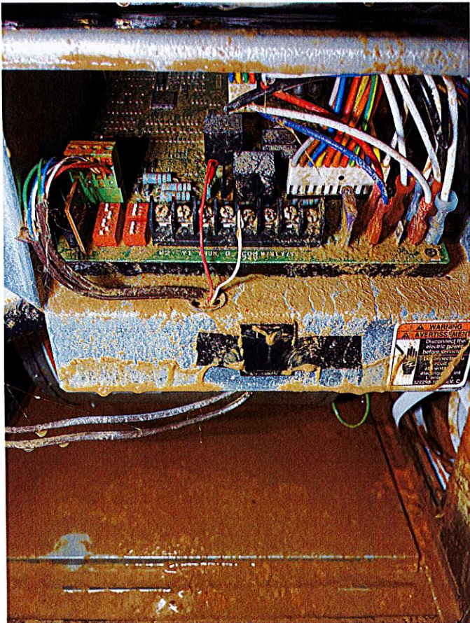
Photo #20: Furnace component damage revealed by Burkhardt technician on March 9, 2022.
