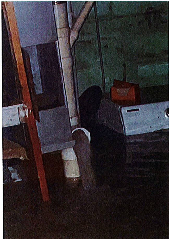
Photo #5: Water rushing in from sewer stack pipe clean out; photo taken at 10:16 p.m. on March 8, 2022.
