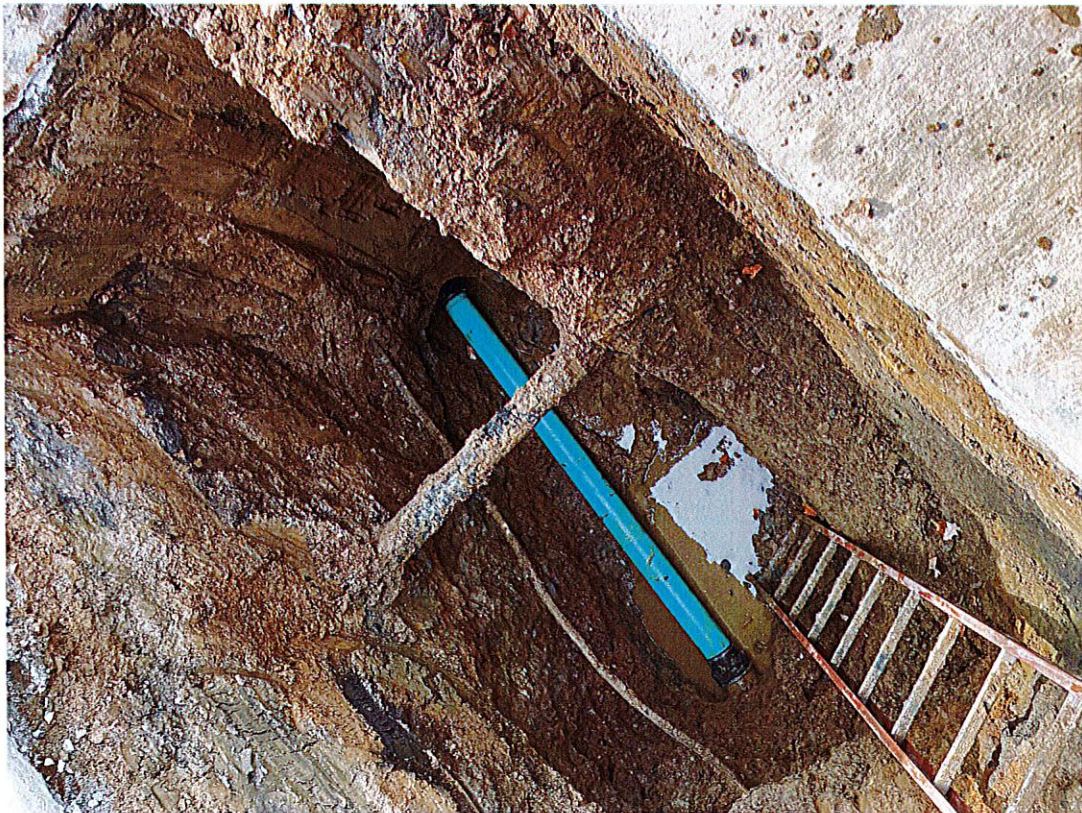
Photo #26: Heiden Plumbing's replacement of city's collapsed lateral sewer drain pipe; taken on March 14, 2022 at 3:19 p.m.
