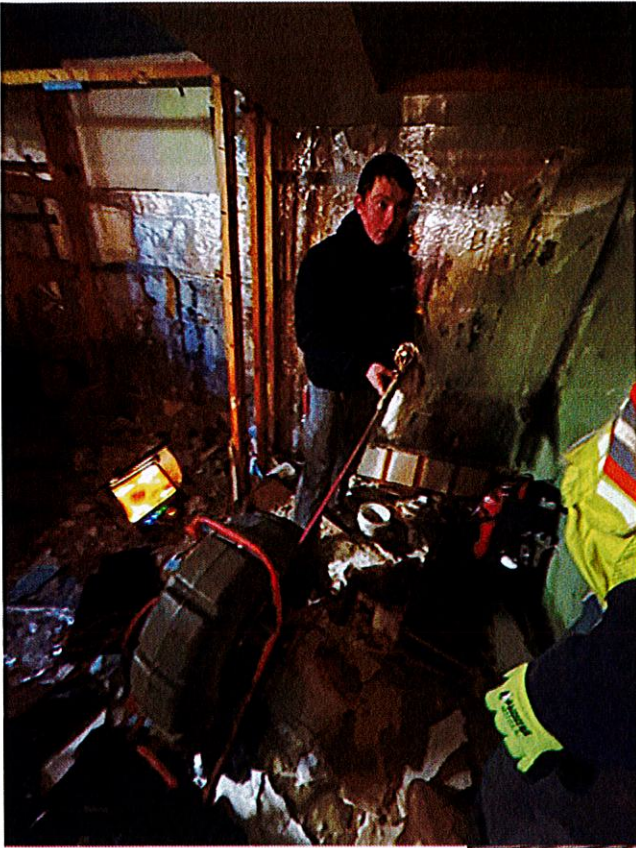
Photo #22: Heiden Plumbing scoping the sewer drain pipe on March 11, 2022 at 10:00 a.m.
