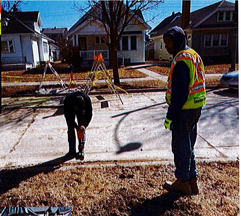
Photo #23: Heiden Plumbing identifying location of city's broken lateral sewer drain pipe on March 11, 2022.
