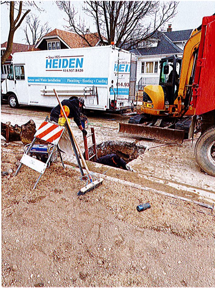
Photo #25: Heiden Plumbing's excavation work to reveal city's collapsed lateral sewer drain pipe; taken on March 14, 2022 at 11:43 a.m.
