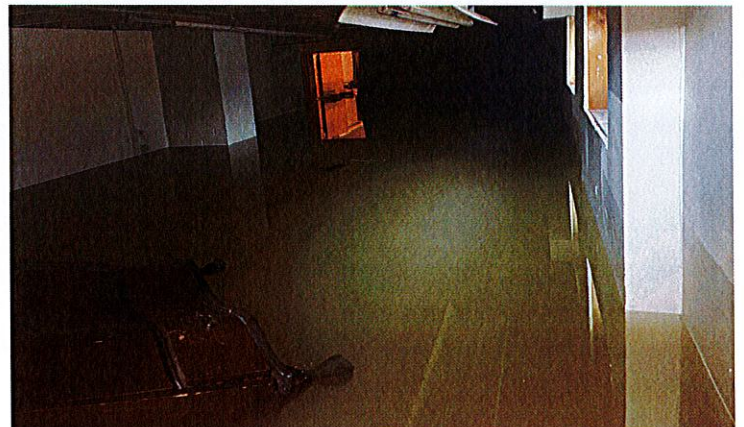
Photo #4: From house's rear door of basement; taken immediately after Patrick Russell arrived on March 8, 2022. Notice water line on wall.
