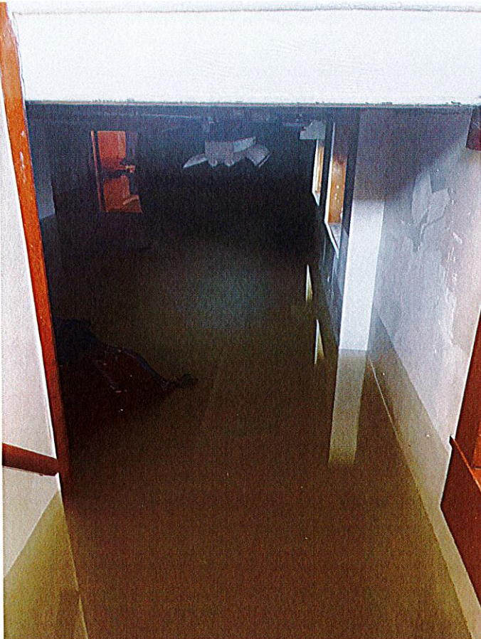
Photo #3: From house's rear door of basement; taken immediately after Patrick Russell arrived on March 8, 2022. Notice water line on wall.
