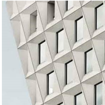
METAL and PRE-CAST PANEL
